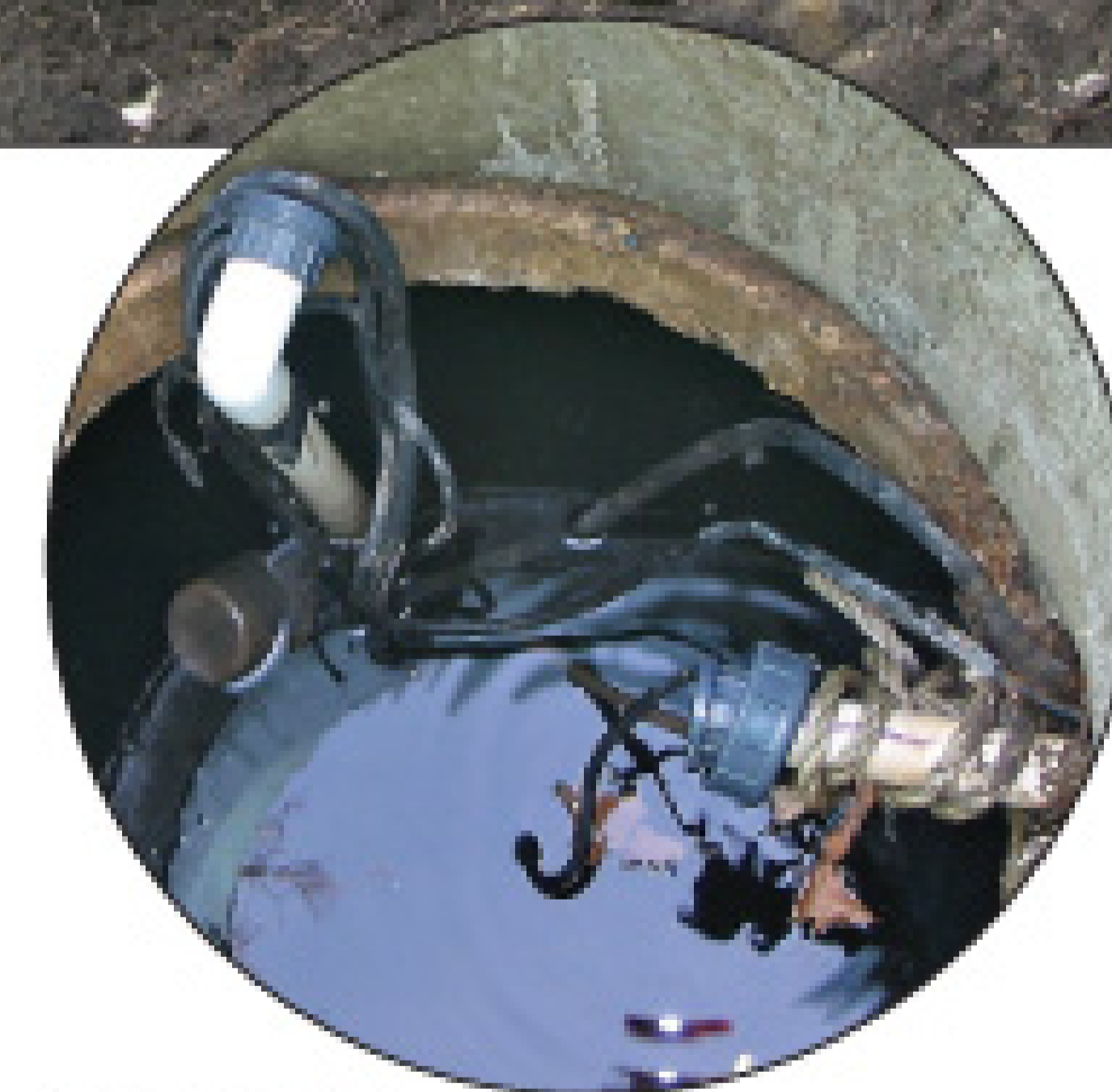
Make sure pumps and controls are accessible from the surface for maintenance and repair.
