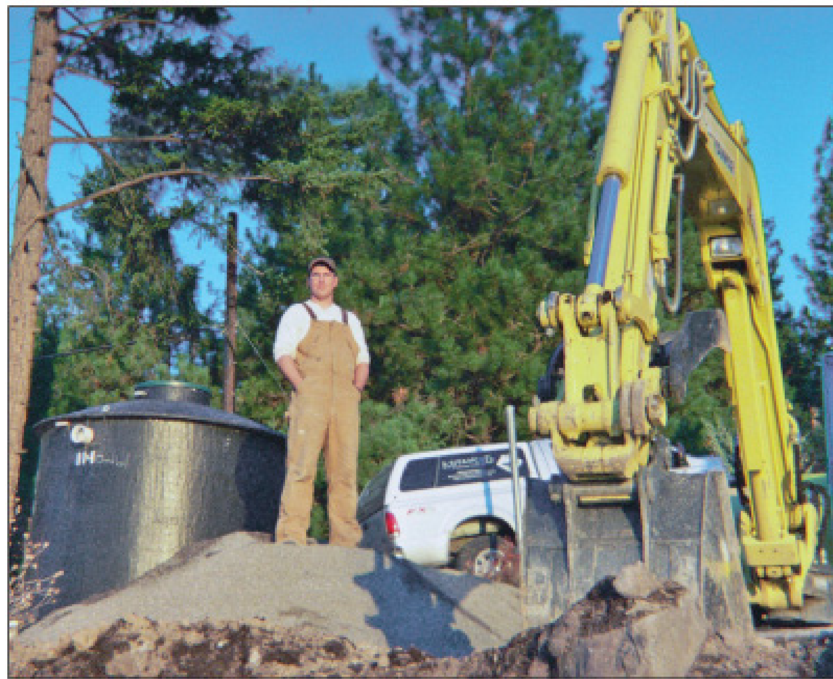
George Miles is shown next to pretreatment unit on a waterfront lot.
