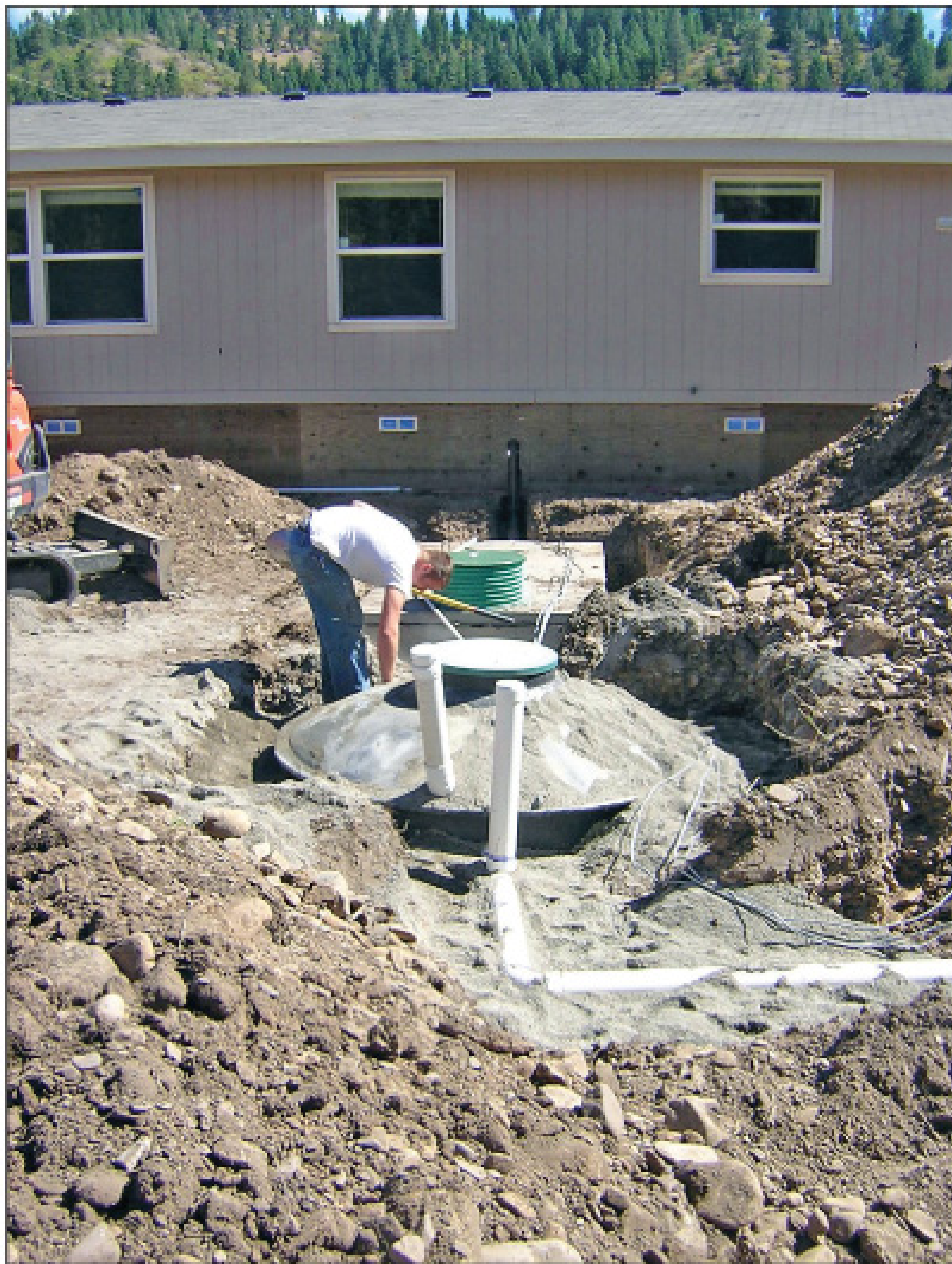
Matt Watts installs a dosed cap and fill drainfield with Delta DF60 treatment unit at Wolf Lodge in Coeur d'Alene, Idaho.
