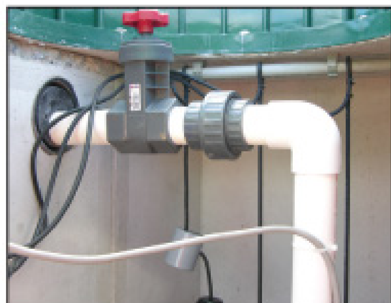
A quick disconnect in a pump tank is an aid to maintenance.
