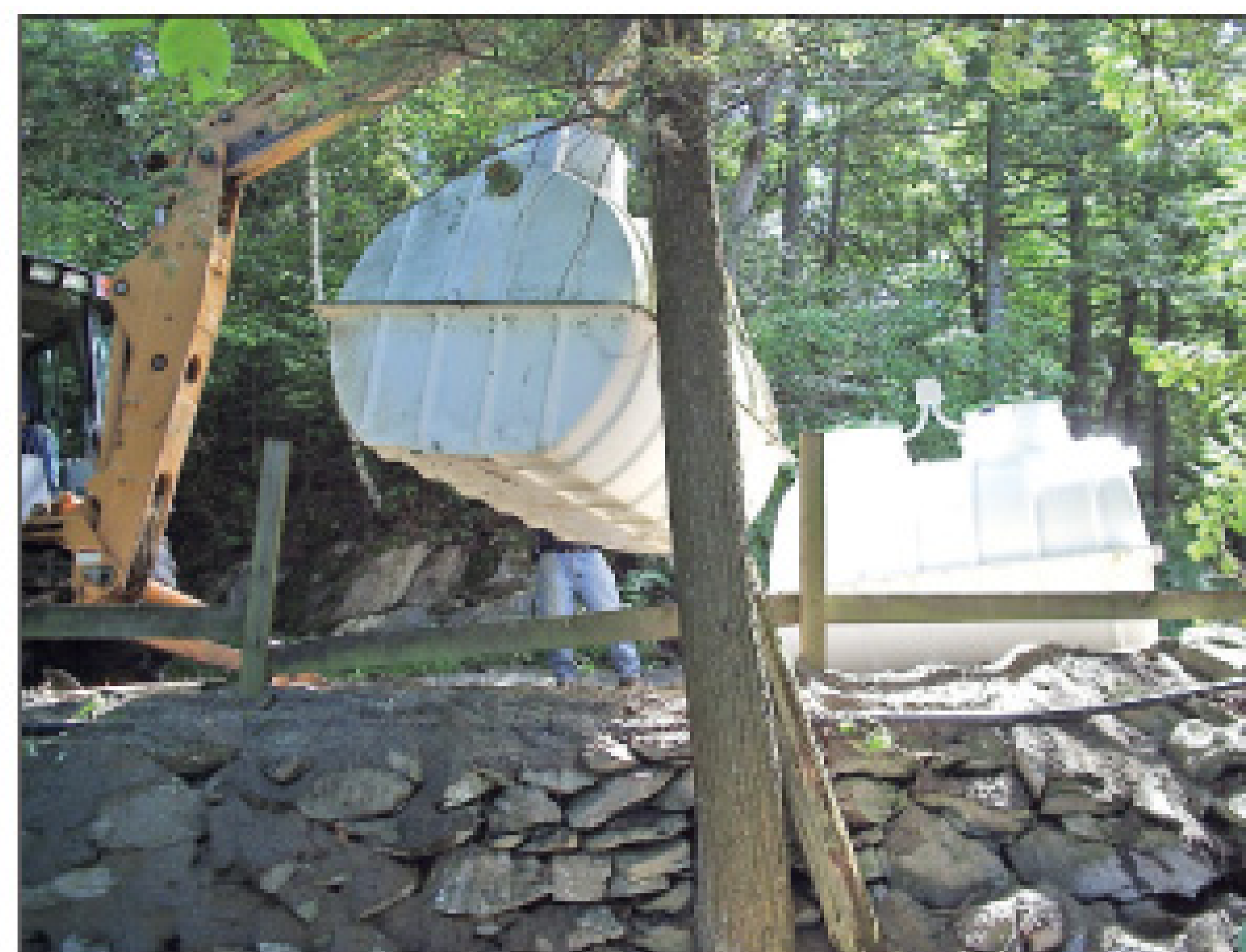
The CA-5 sequencing batch reactor (background) is shown awaiting installation as a backhoe operator hoists the old module from what will become the drainfield.
