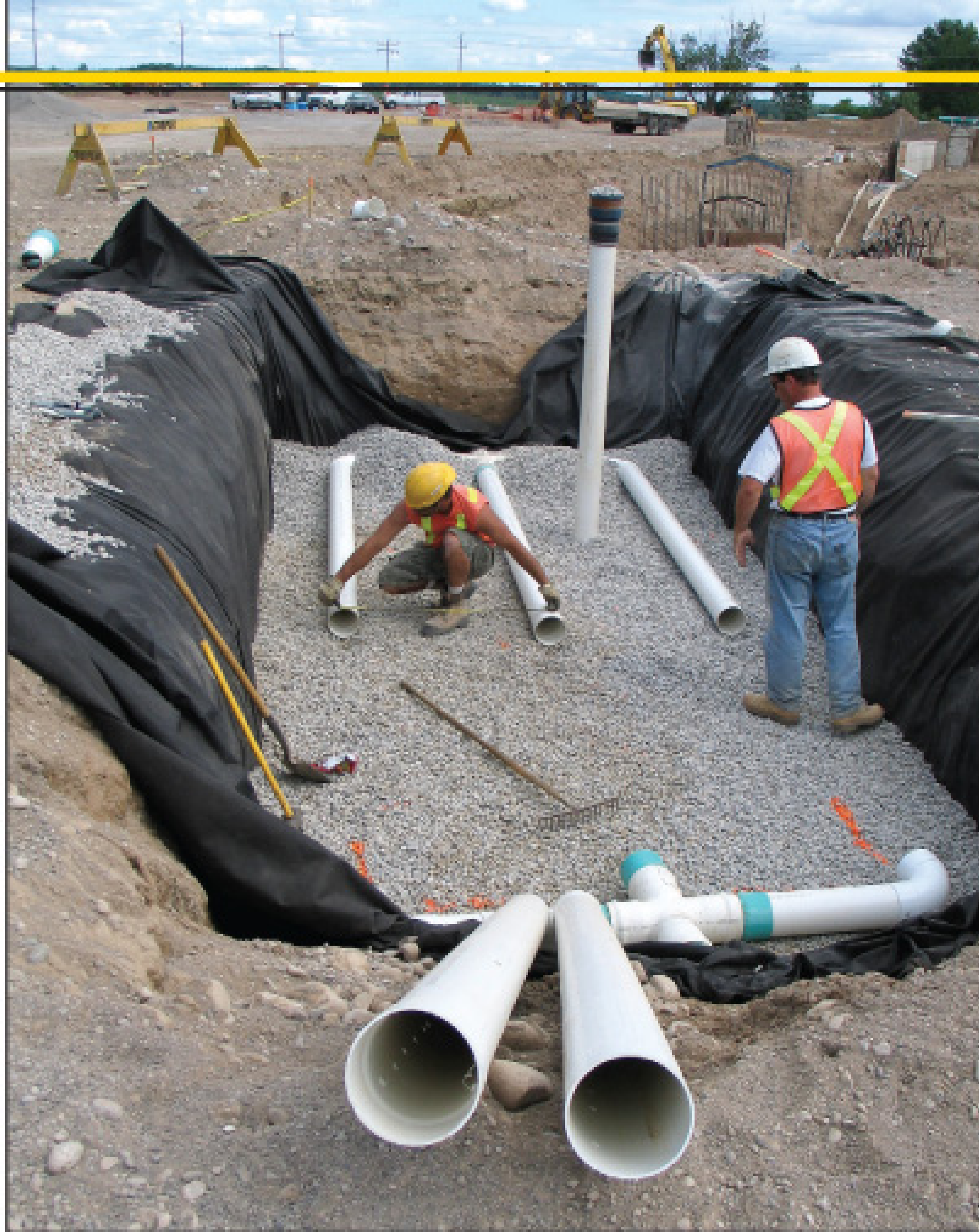
John Van Neiuwenhuizen (left) and Dave Mc Cready from D.W. Cooper Contracting install a rainwater infiltration gallery.
