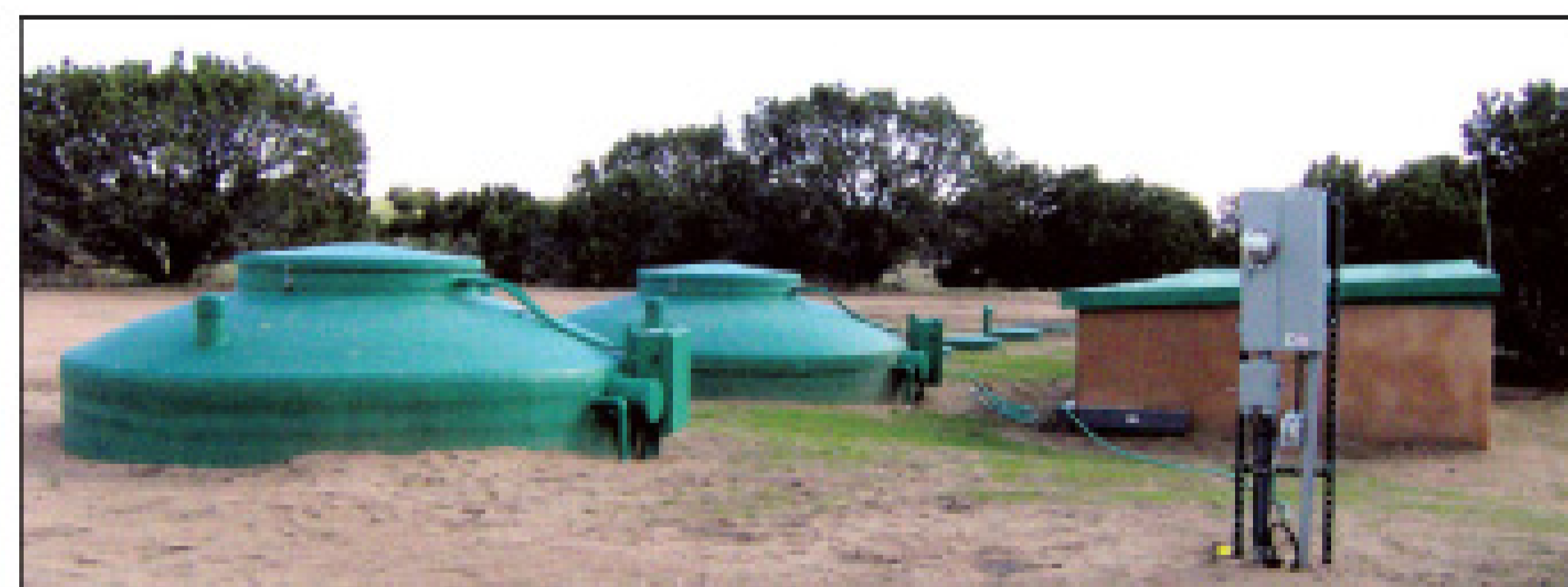
Recirculating trickling filter systems from Koi Environmental Inc.
