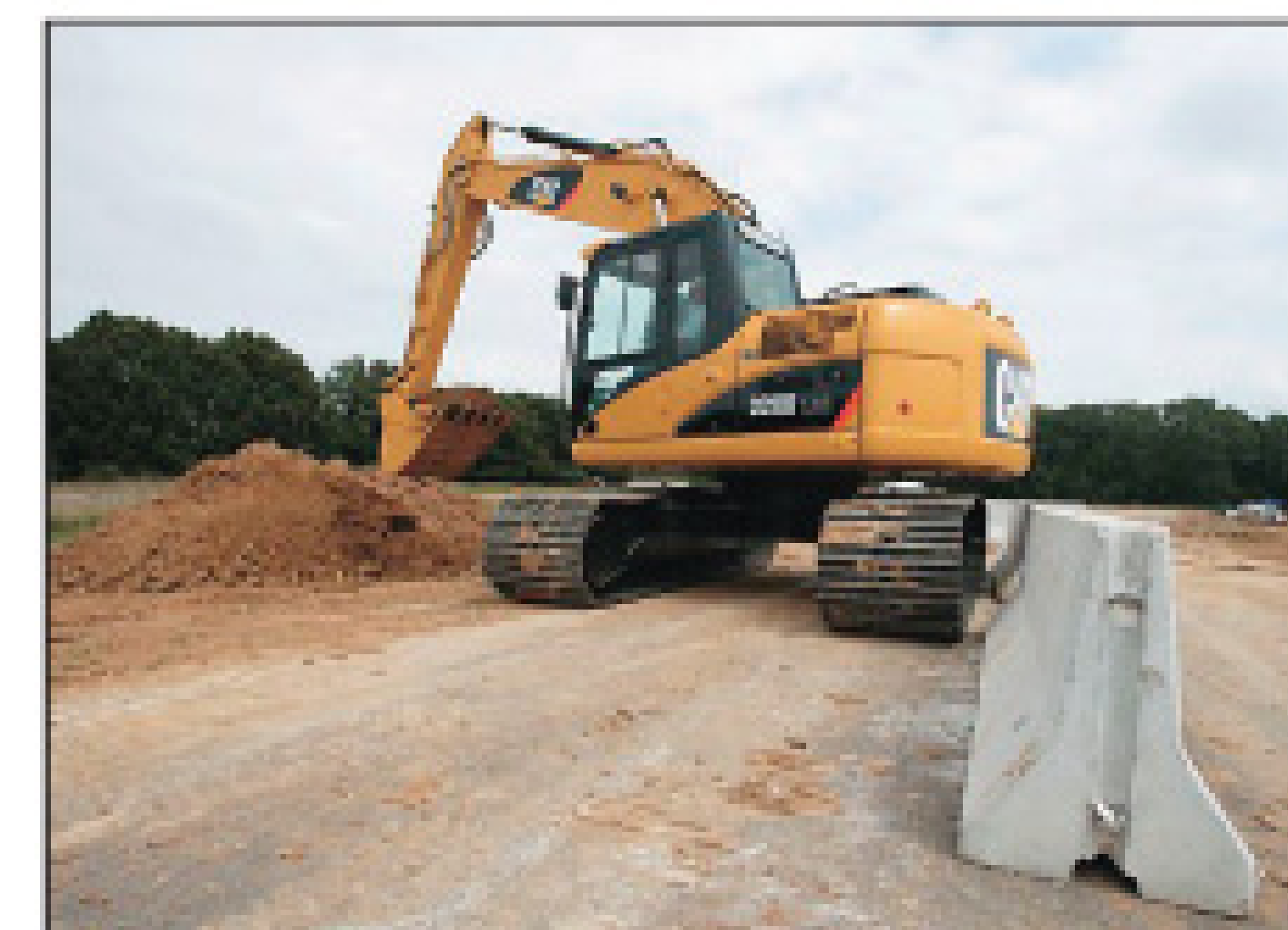
The Cat 320D LRR reduced-radius excavator illustrates a tail-swing radius that is shorter than a conventional machine but longer than a compact-radius excavator.
