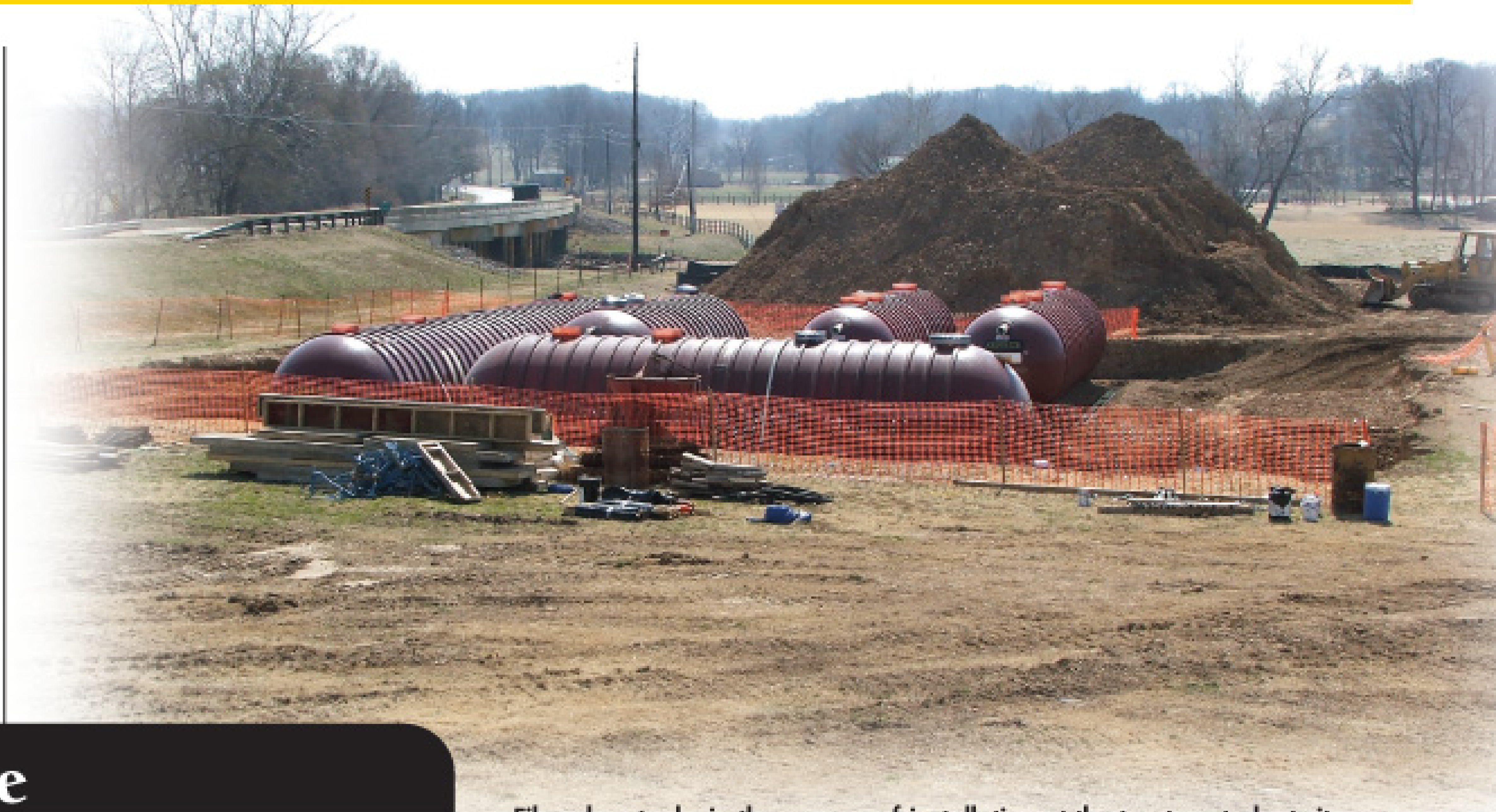
Fiberglass tanks in the process of installation at the treatment plant site. (Photos courtesy of Aqua Tech Systems LLC)
