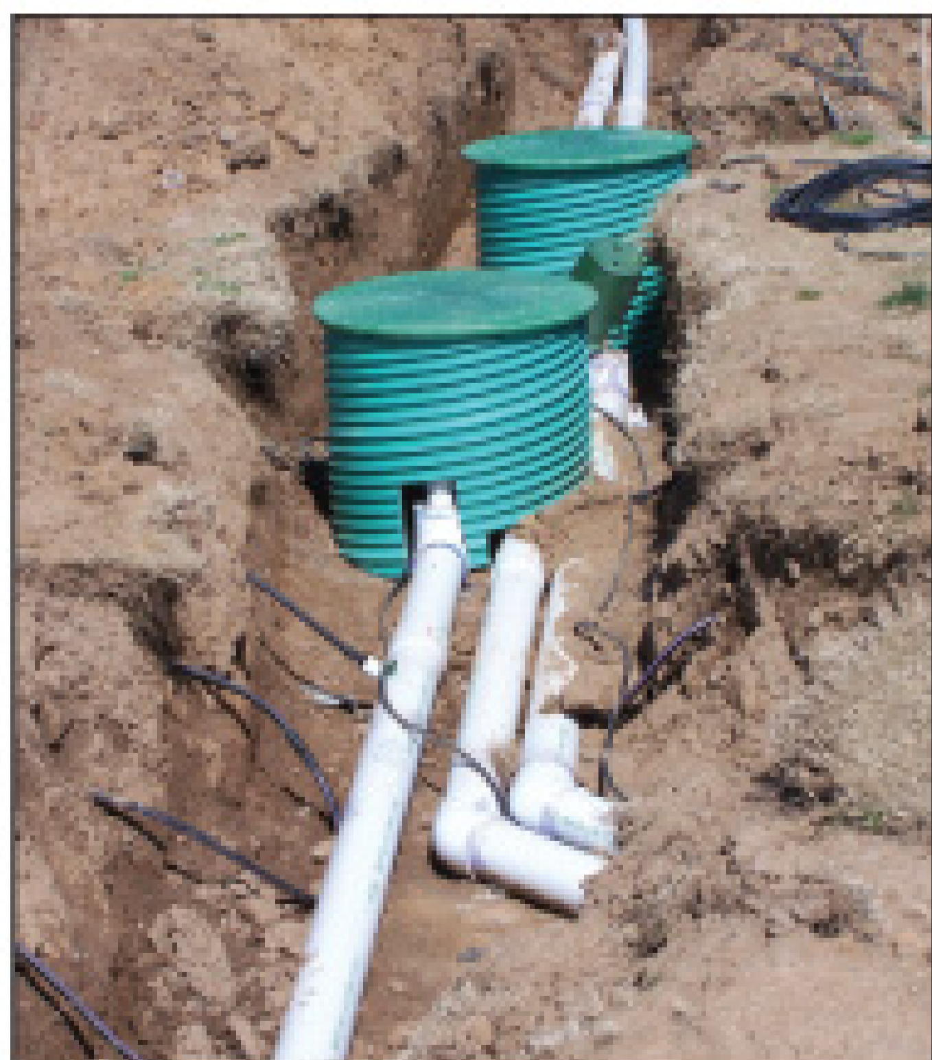
Electronic zone valves (inside risers) are shown at Dripfield 2.
