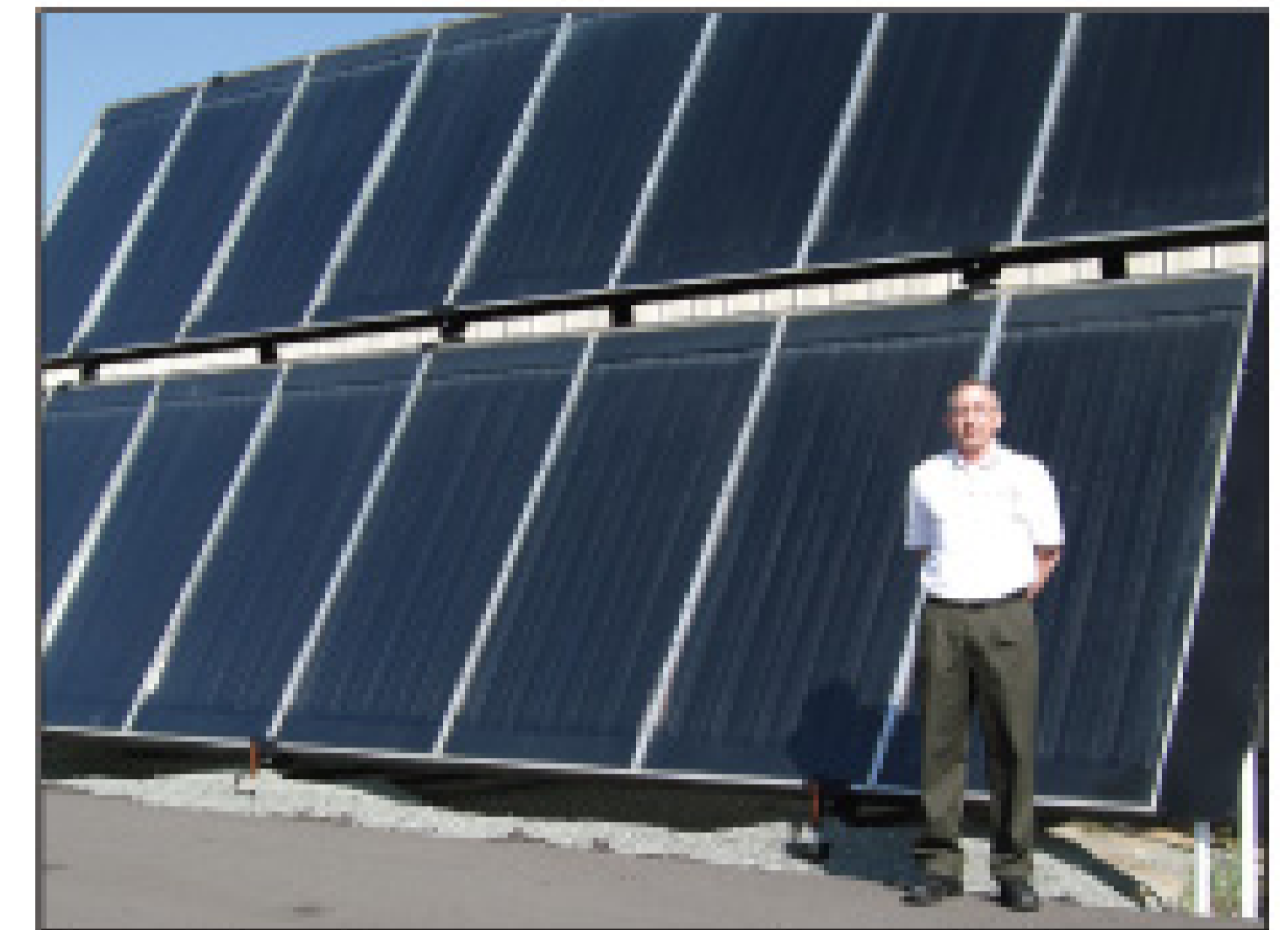
Jerard Nighorn, vice president of sales, stands next to the solar heat panels installed at the Lenzyme facility.
