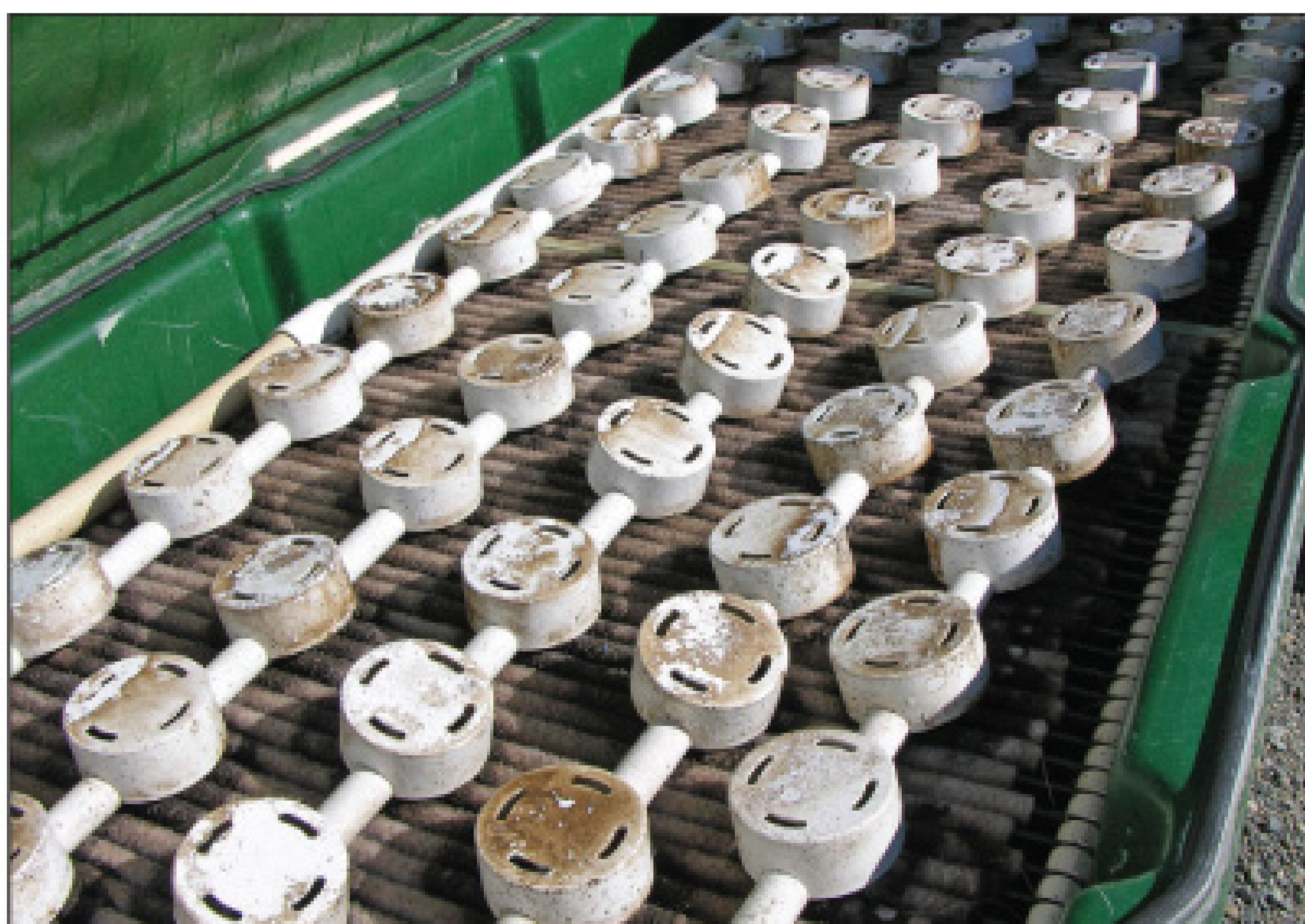
A textile filter like this one provides additional treatment to septic tank effluent.
