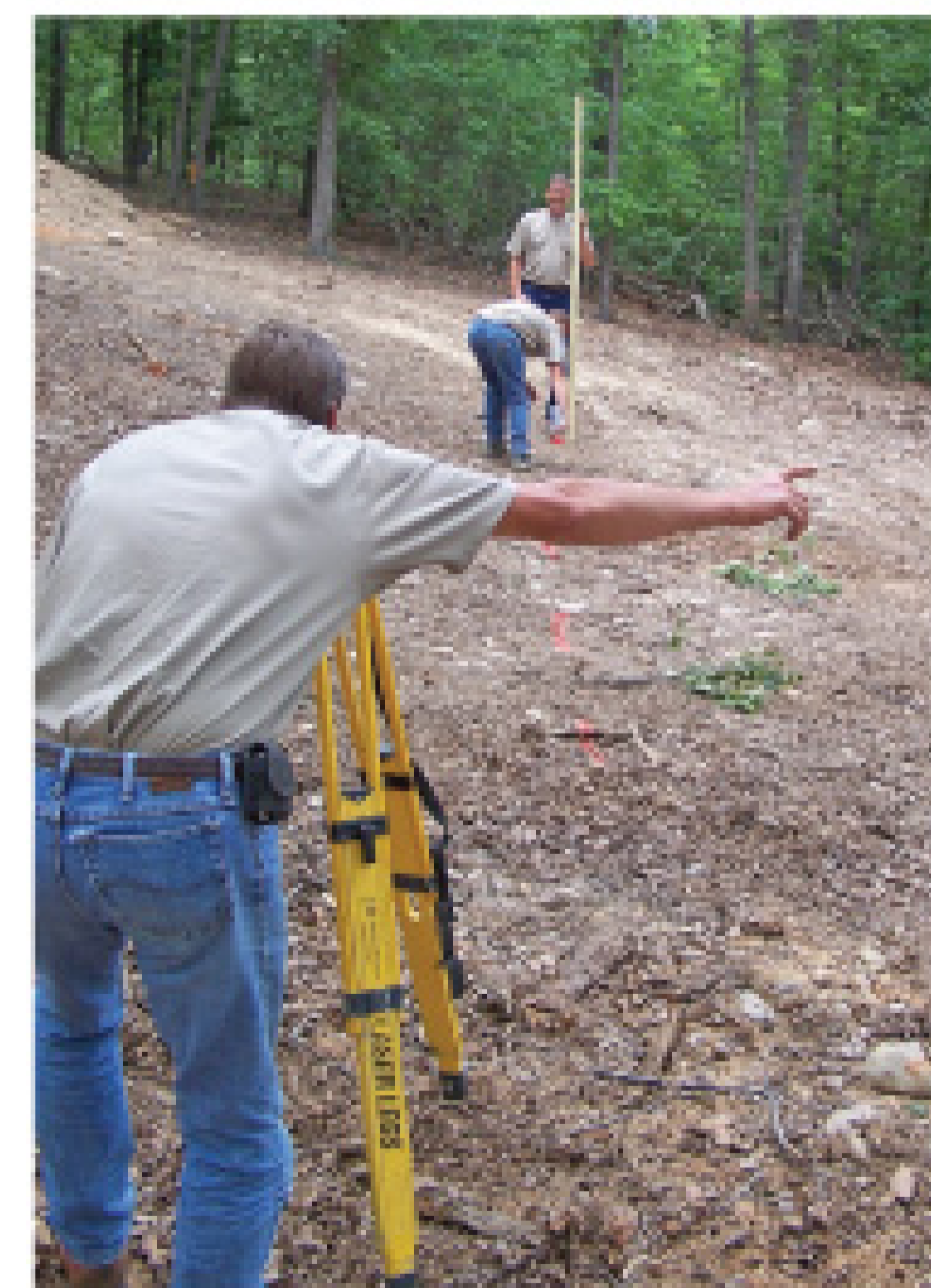
The team at Megeath Contracting marks contour lines at an installation site in Andy Guest Shenandoah River State Park. Drip tubing will be placed on the site.
