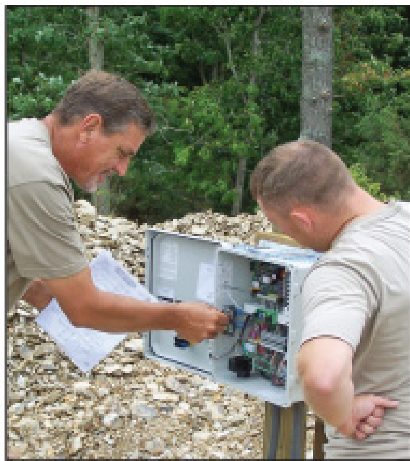
Art Megeath, owner of Megeath Contracting, goes over an onsite system's controls with the new owner, Jeremy Ramos.
