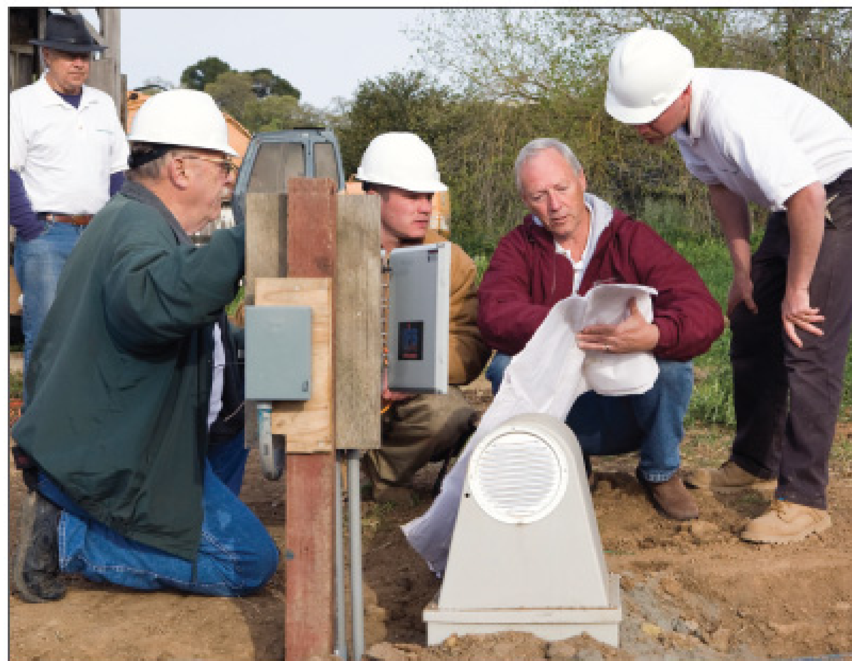
Engineer Terry Craven and the Engineered Septic team set a control panel before final inspection. (Photo by Paige Green)
