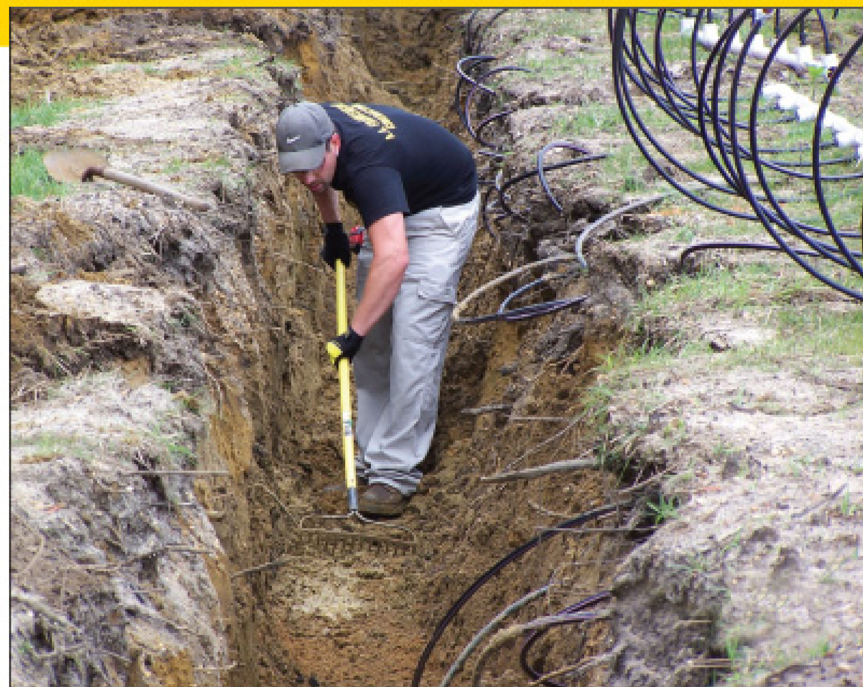
Tim Wolf levels a trench before connecting the drip lines. (Photos courtesy of AA Frankenfield Contracting)
