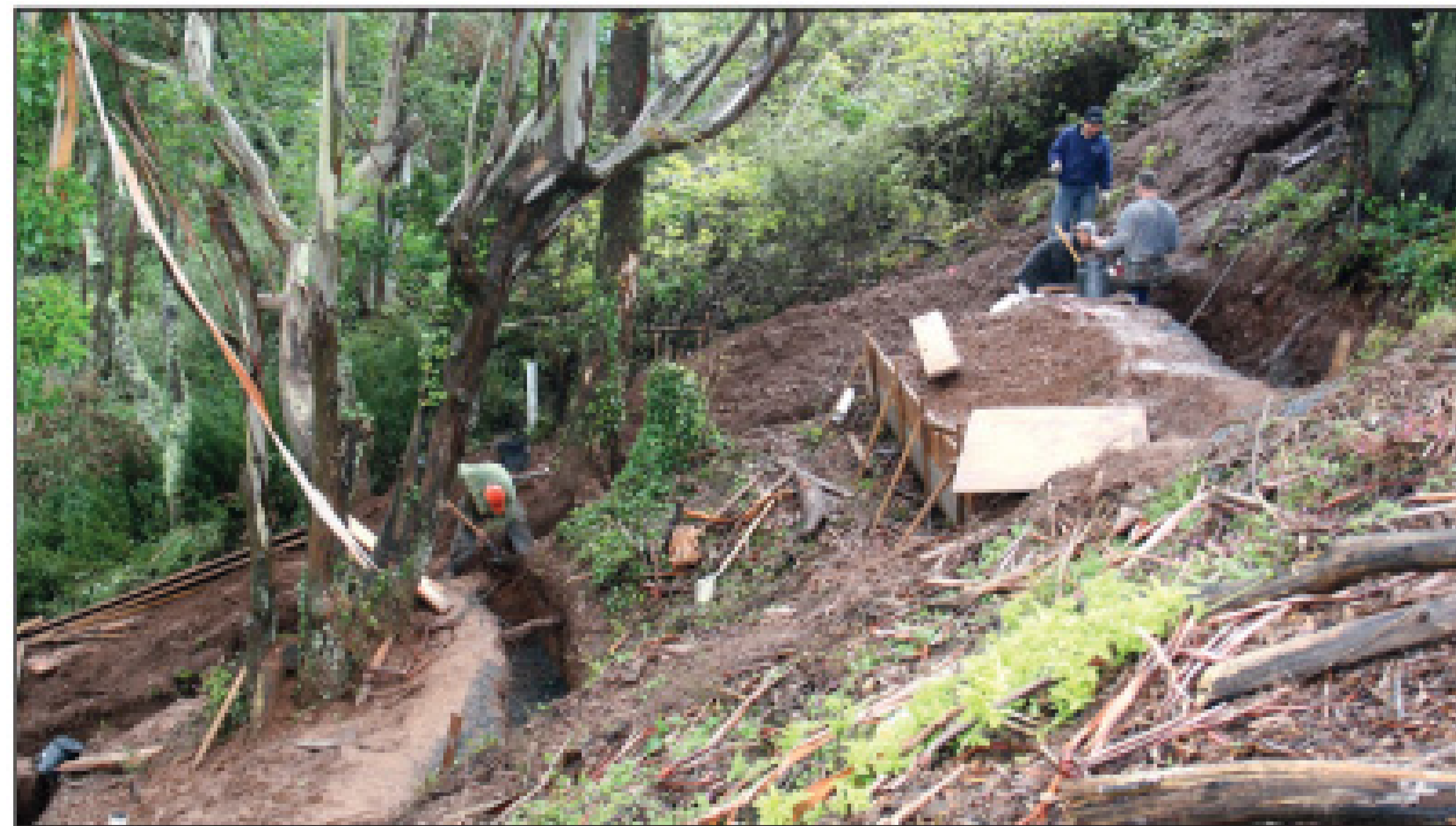
A work crew is shown with a hand-dug leachfield next to Golden Gate National Recreation Area. (Photo by Ashley Wexler)
