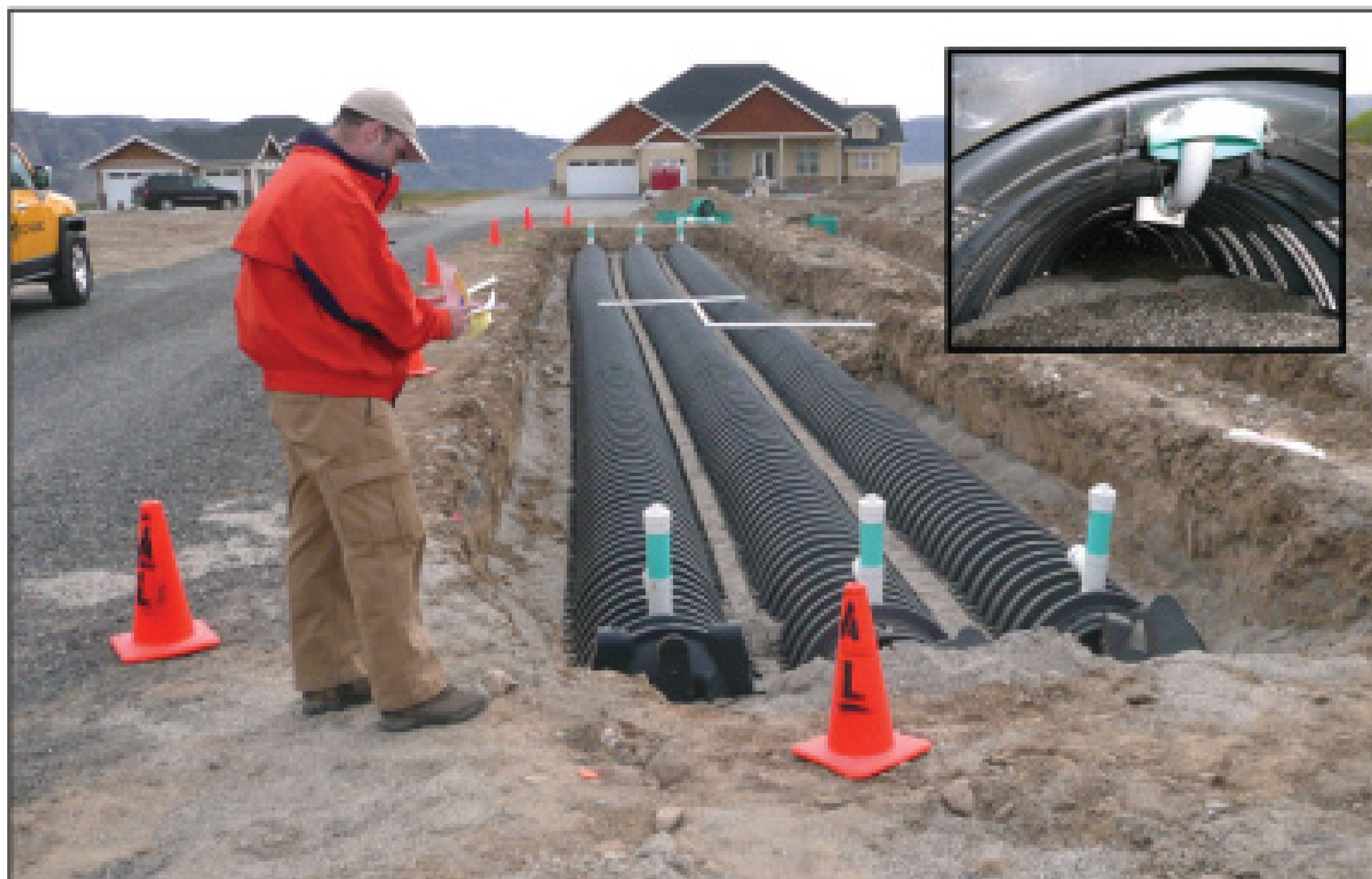
PHOTO B: A center manifold drainfield with improved ports is being inspected. Unlike the standard design, these ports can be used for squirt testing as well as for inspecting the interior of the drainfield. The inset shows the base of the port inside the last vault with the lateral sweep held in place by a quick-tie.
