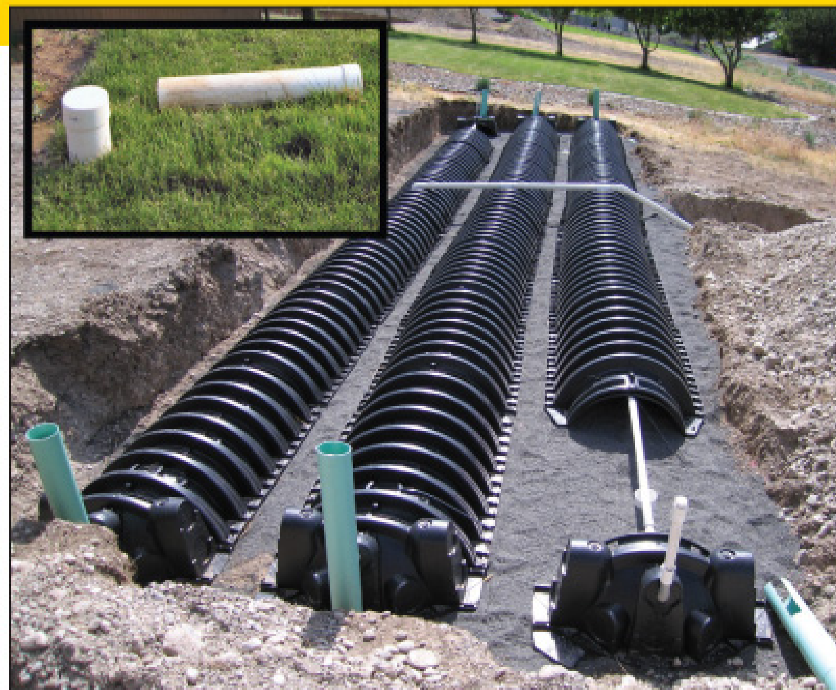
PHOTO A: A conventional drainfield is shown almost ready to cover. The inset photo shows the finished lawn with the slip caps sticking up. One has been extracted from the system by the owner. (Photos courtesy of John Glassco)
