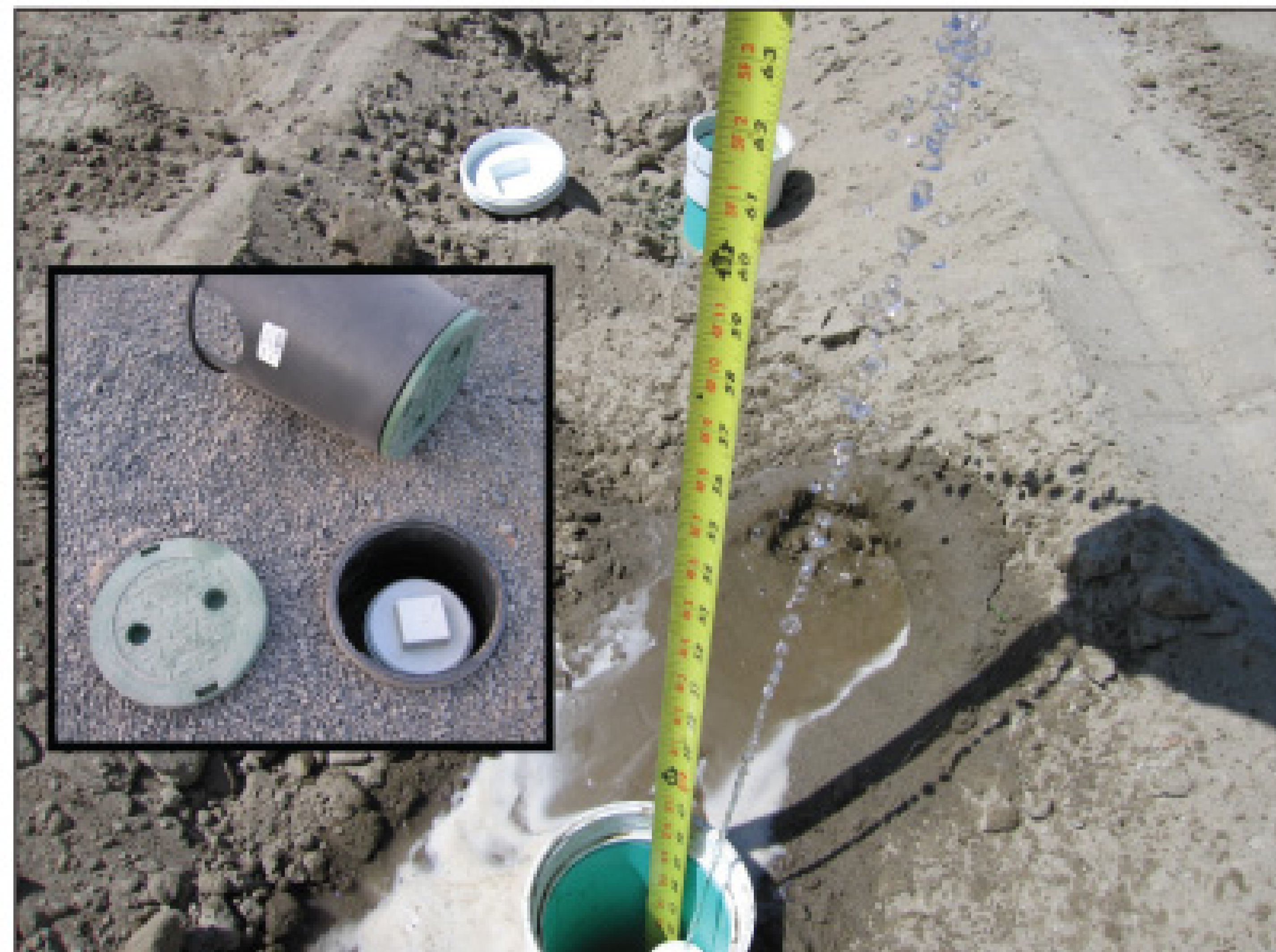
PHOTO C: This system is being squirt tested and shows a 64-inch squirt. The tape is hooked on the bottom of the port at the lateral elevation. The inset photo shows the finished appearance using 7-inch PVC round valve vaults.
