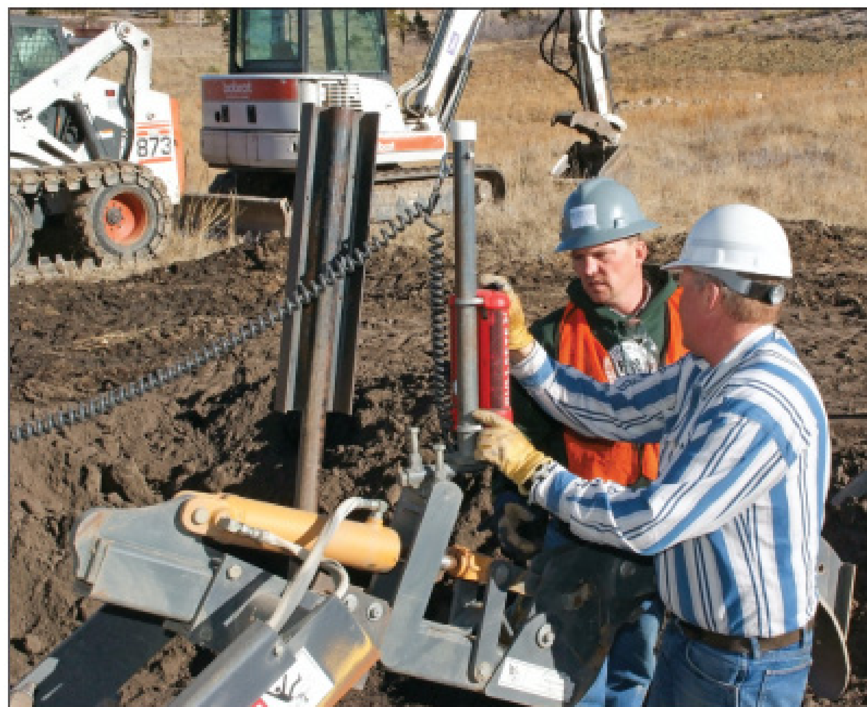
Scott Kellogg (left) digs a leachfield with a Case 660 trencher. His firm offers a menu of services in an approach he describes as a “one-stop dirt shop.”
