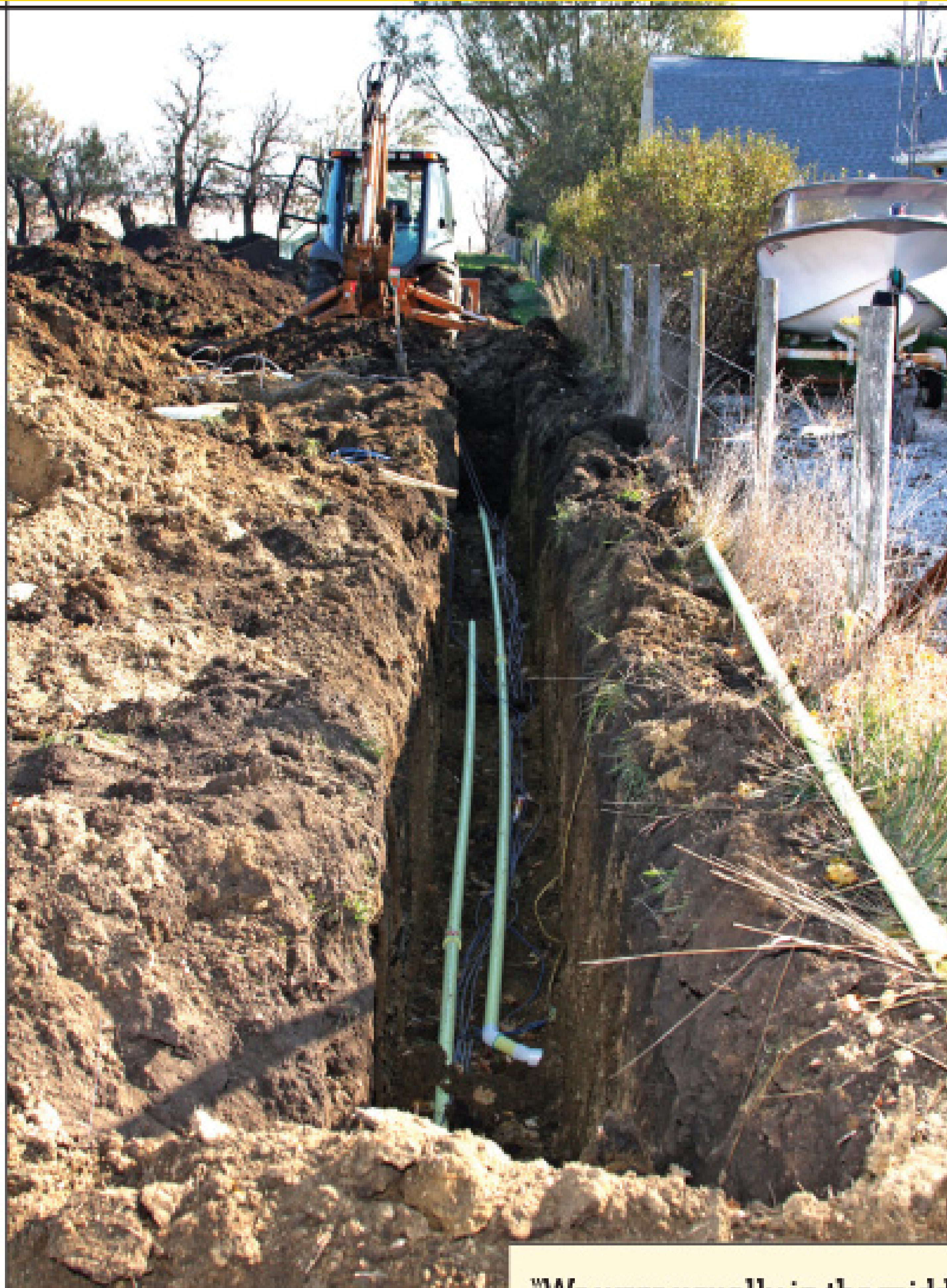
A 2-inch pressure line connects the home to the septic tank.
