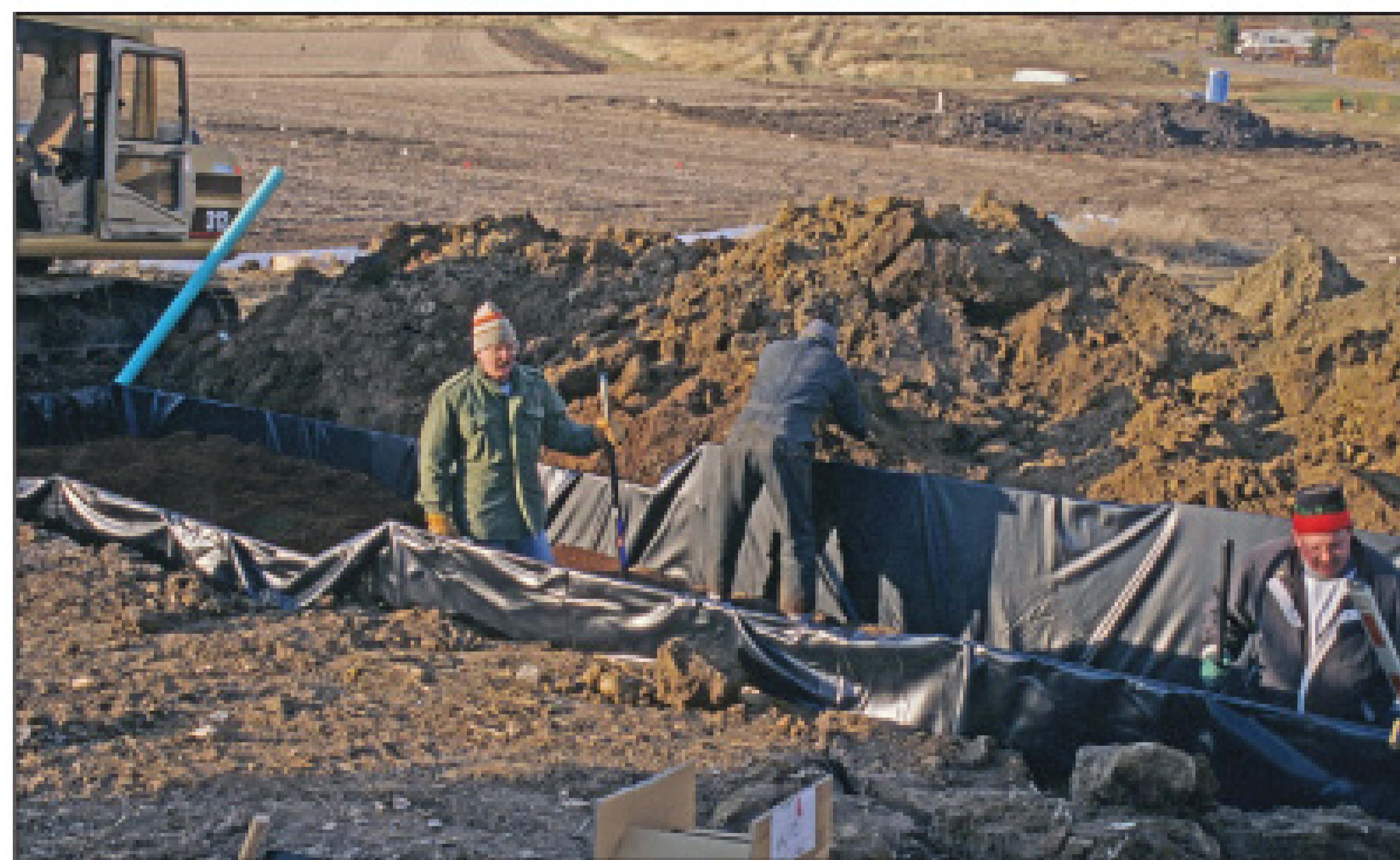
Proper installation of lining material is essential to long-term filter performance and effective treatment.
