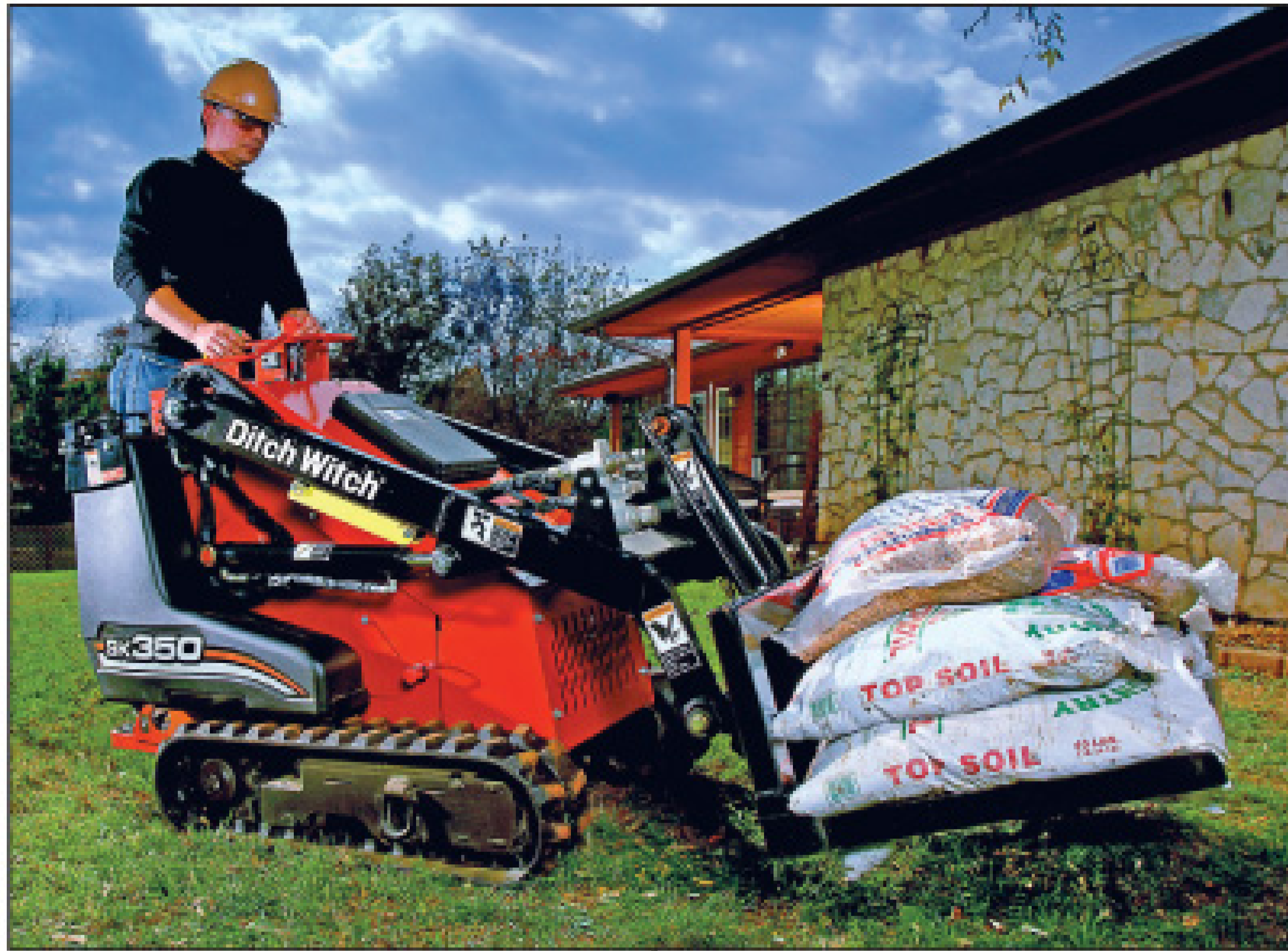
This Ditch Witch SK350 mini-loader makes quick work of a landscaping job.
