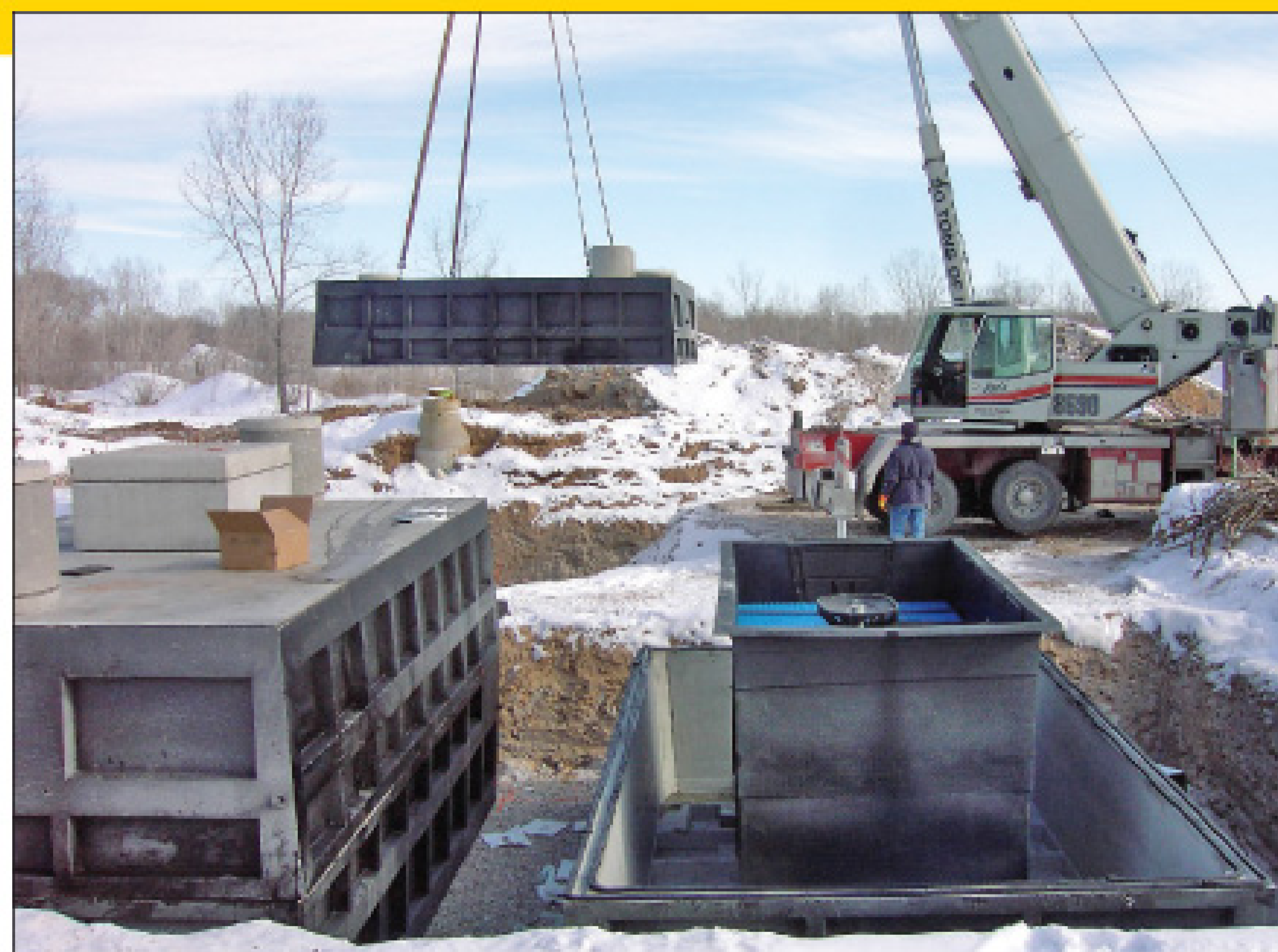
An operator from Jon's Crane and Rigging of Fond du Lac, Wis., uses a 90-ton Link-Belt crane to set the top half of the tank on the south FAST unit. (Photos courtesy of Martenson & Eisele Inc.)
