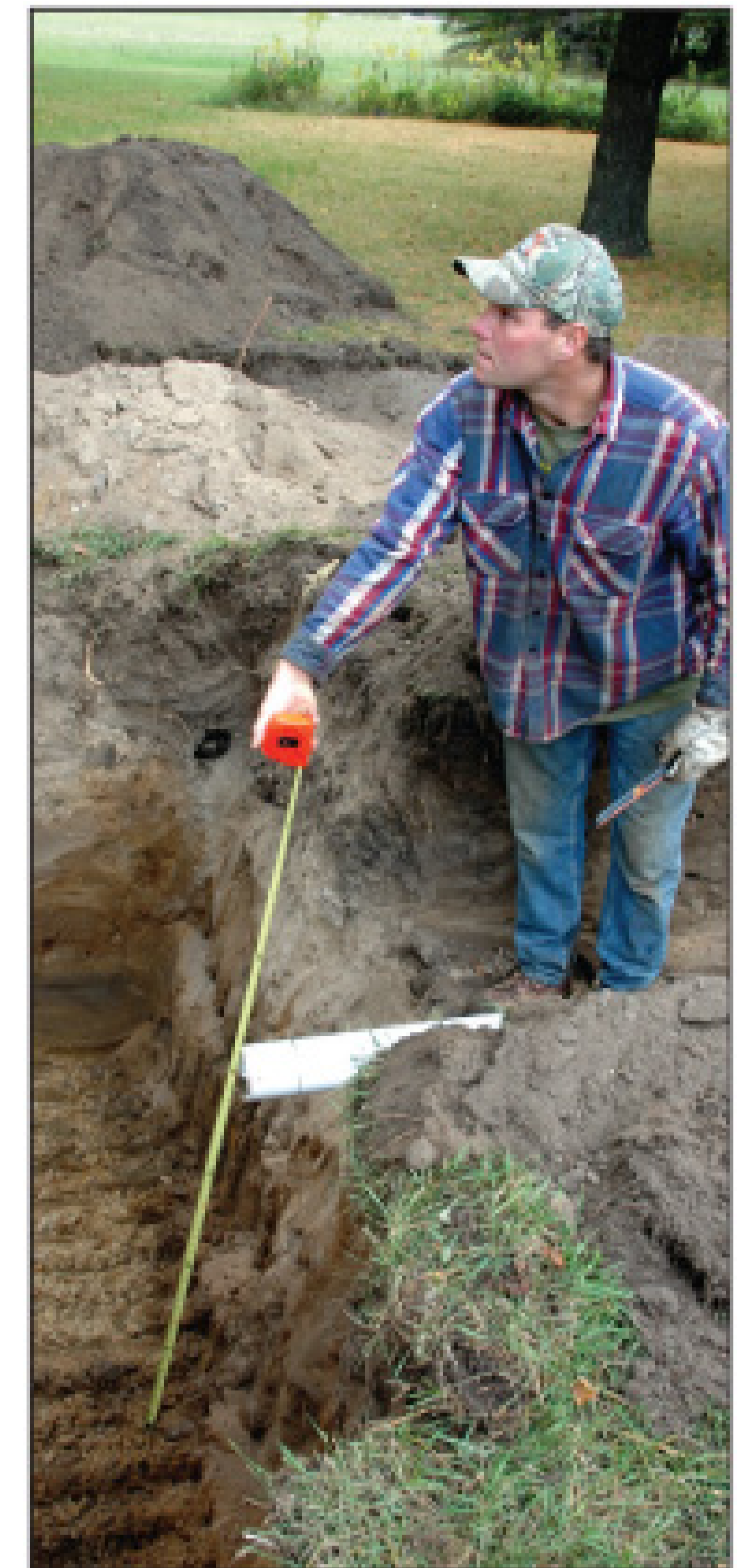
Louis Roggenkamp takes final measurements and makes a level check to ensure that a septic tank will be placed correctly.
