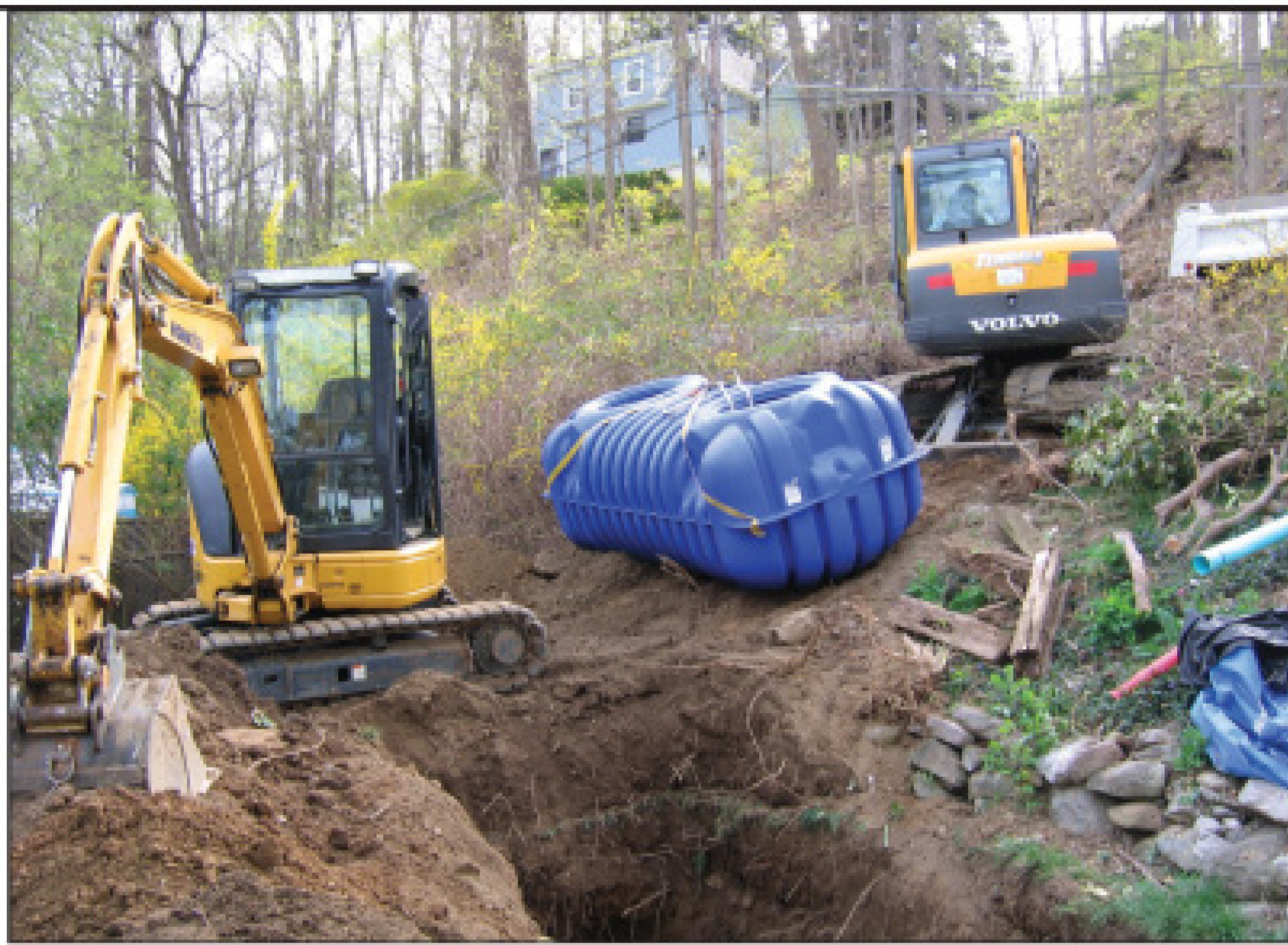
The septic tank is ready to install at the lakeside lot to serve a three-bedroom home in Carmel, N.Y. (Photo courtesy of John Kalin)
