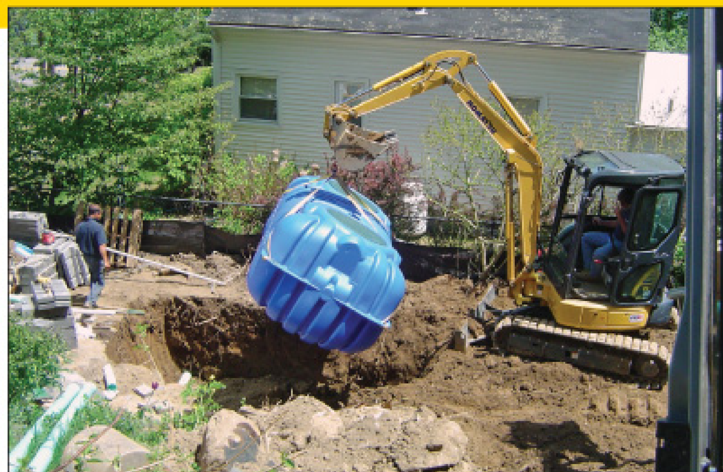
An excavator operator places a 1,000-gallon dual-compartment Fralo Plastech septic tank from Roth Global Plastics within the 500-foot distance from the high-water mark of Lake Carmel. (Photo courtesy of Pat Tyndall)
