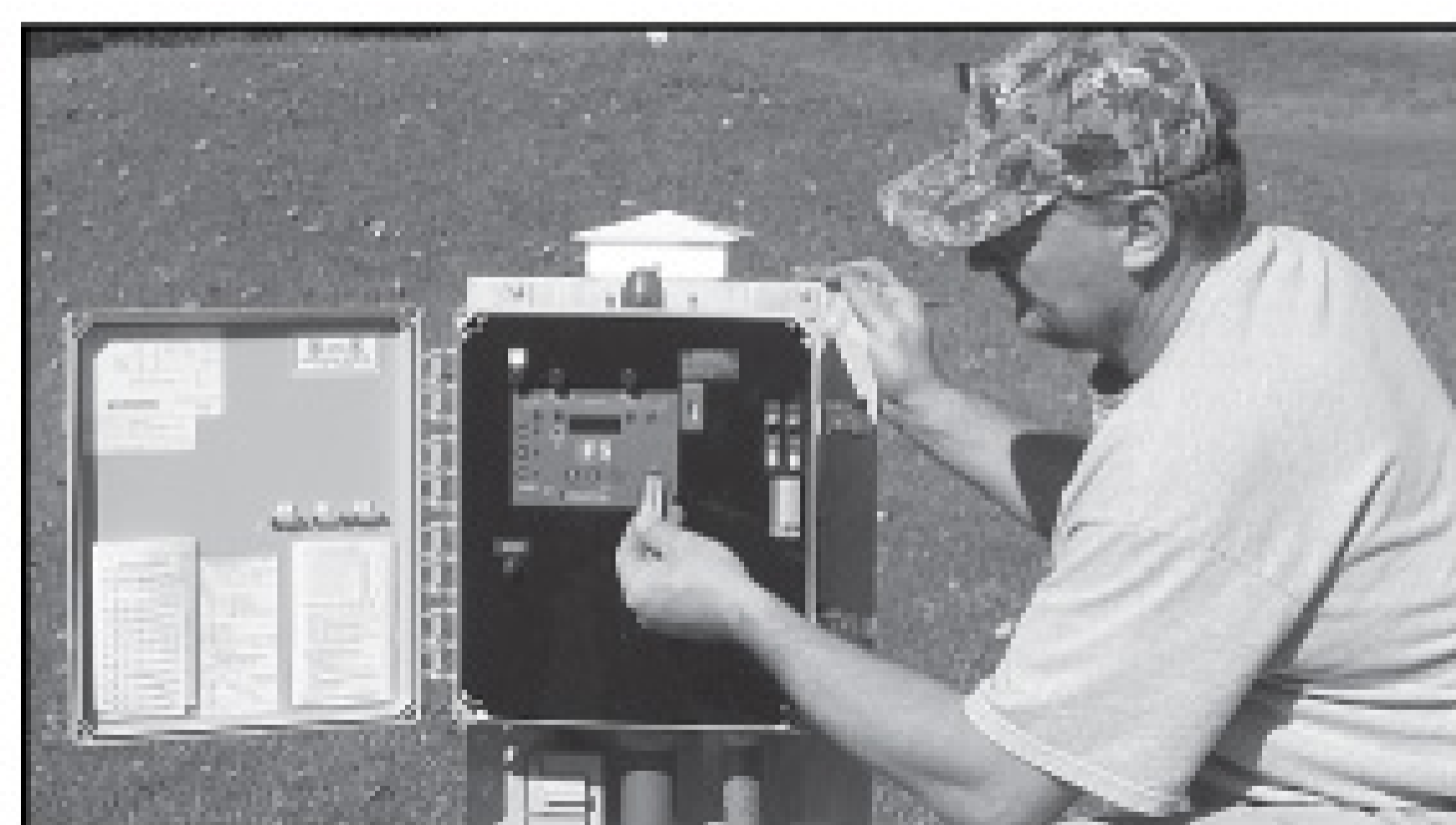
IFS In-Site Event Monitoring Control Panel
