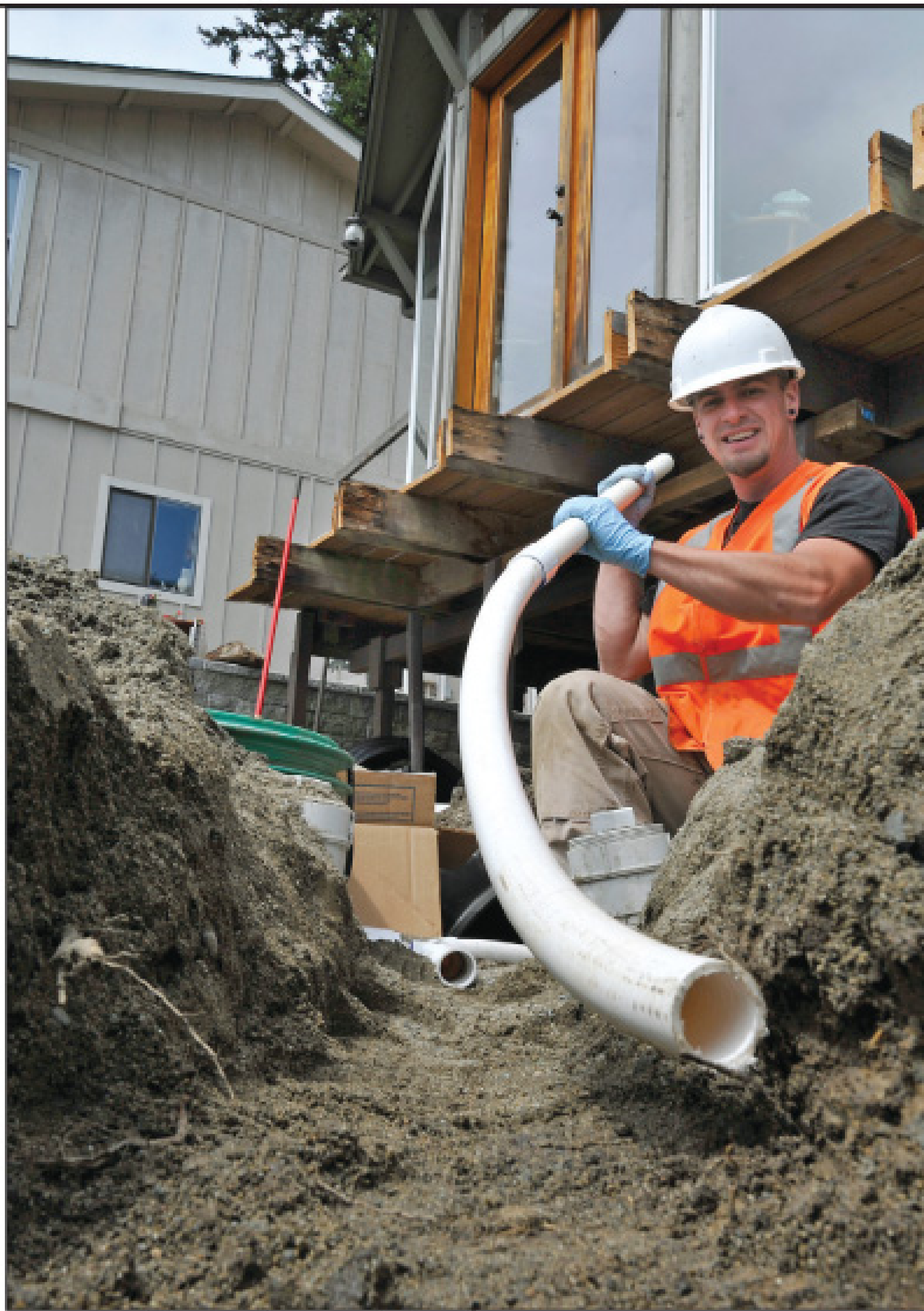
Adam Jewell cuts and glues plastic drainfield lateral piping for a homeowner's onsite system.
