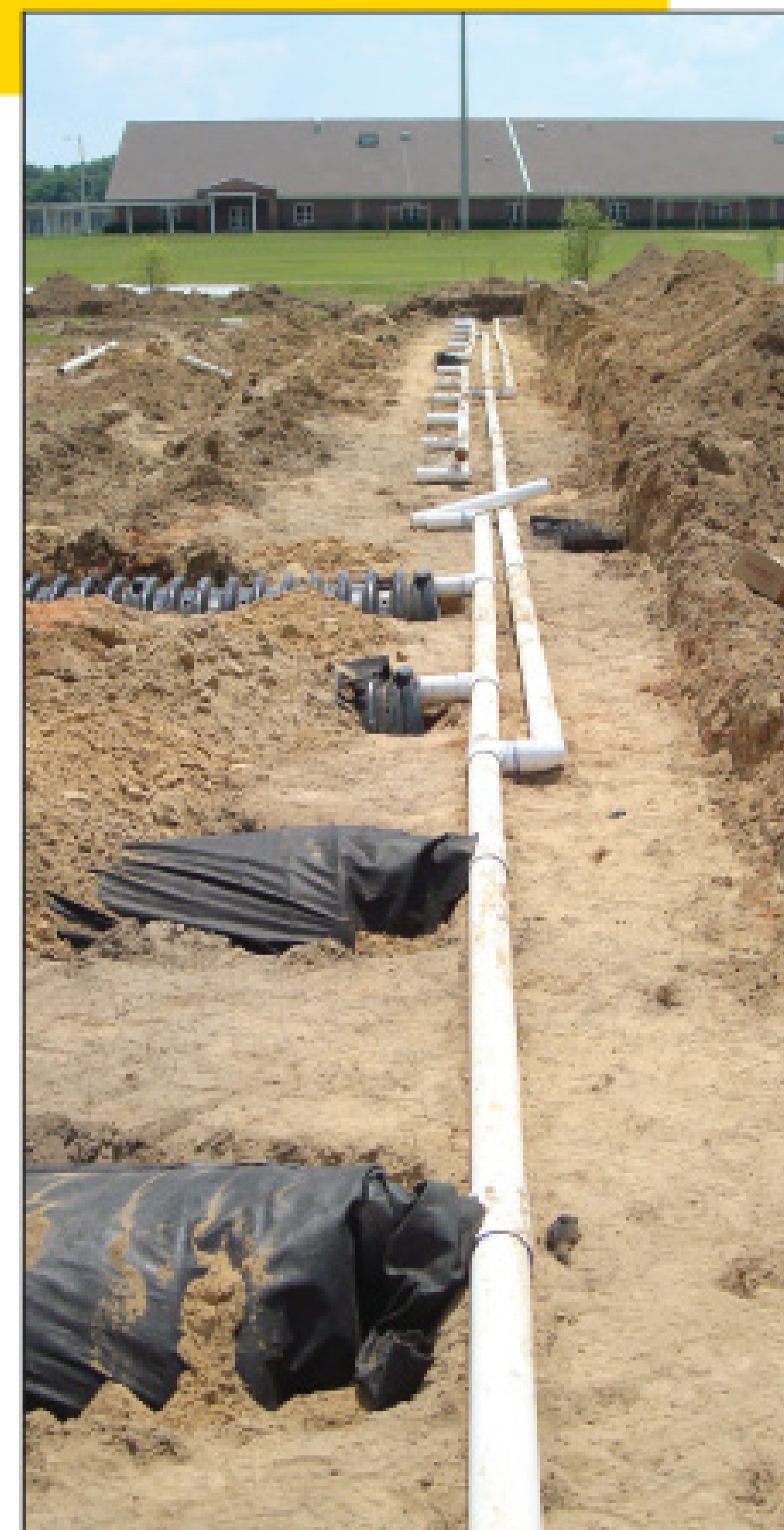
Some of the 1,400 Hi-capacity Envirochambers are shown installed in the Phase 2 drainfield. (Photos courtesy of Hughes Plumbing & Utility Contractors Inc.)
