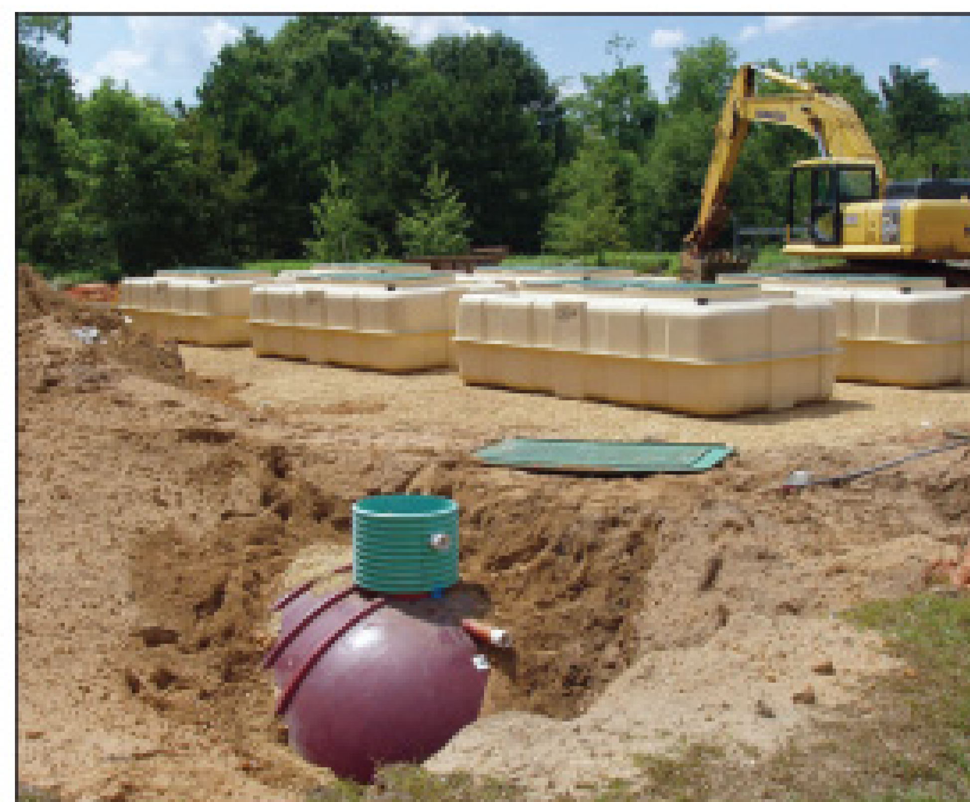
Workers positioned the six 5,000-gallon AeroCell fixed-film treatment modules on the surface next to the recirculation tank.
