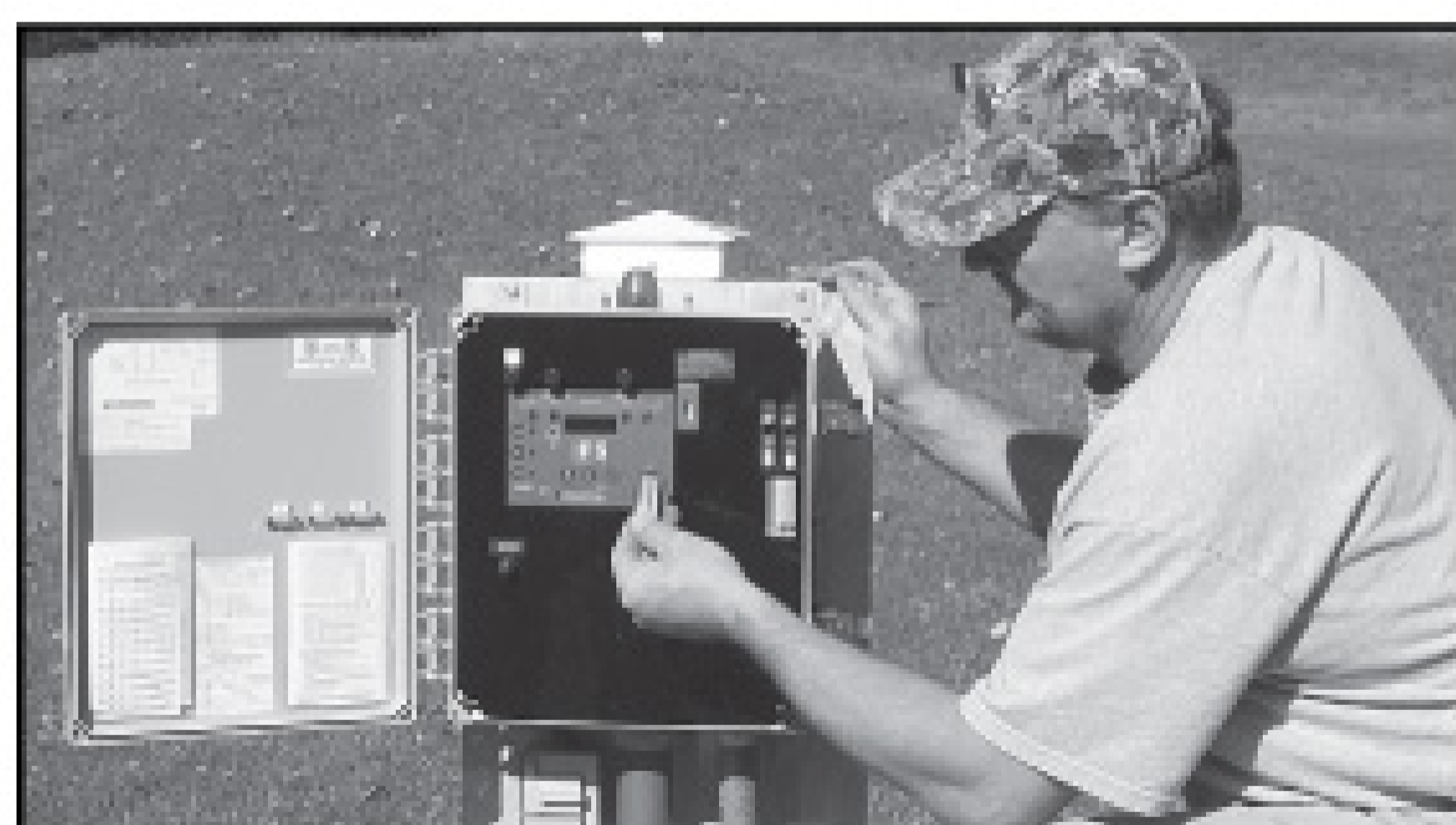
IFS In-Site Event Monitoring Control Panel
