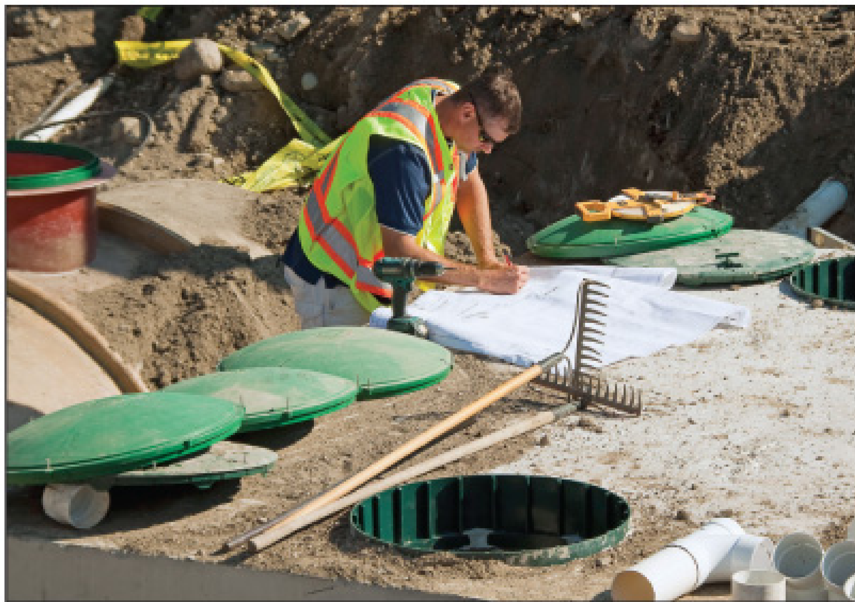
Engineer Rob Arden, system designer, makes preparations to observe a squirt test on a Rivermist onsite system and to inspect the installation.
