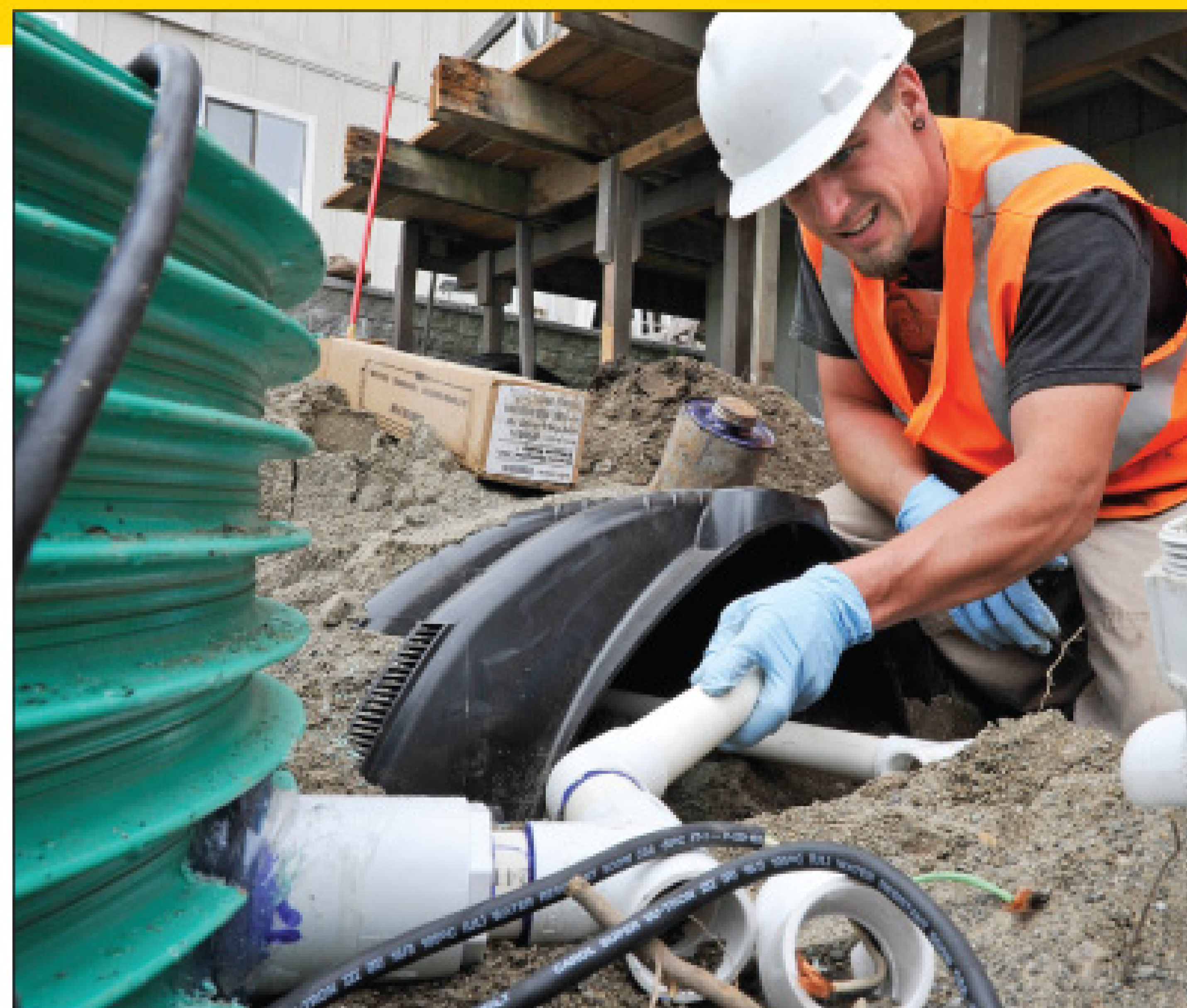
Adam Jewell assembles the transport line for the graywater treatment system. (Photos courtesy of A Advanced Septic Services Inc.)
