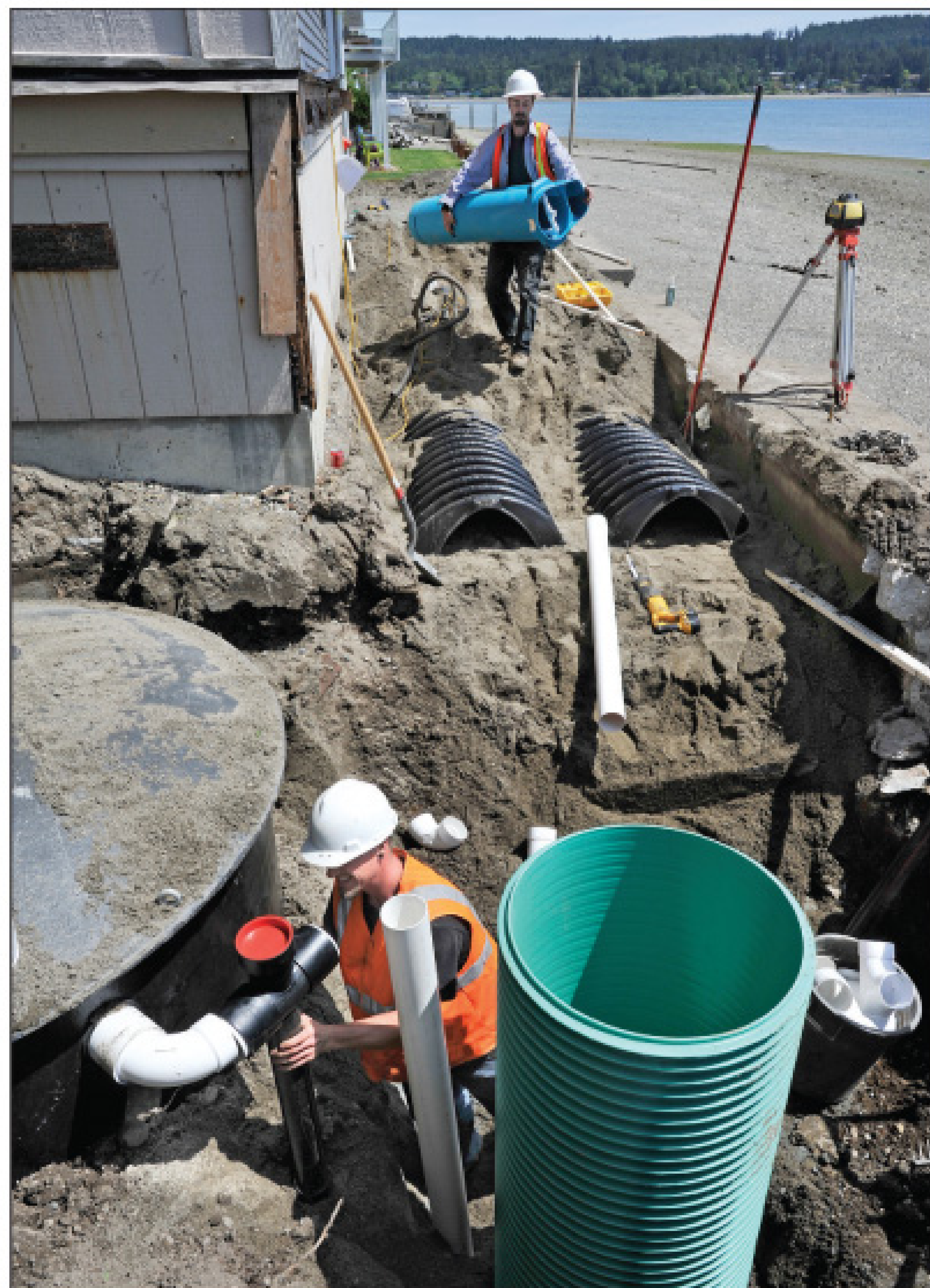
Adam Jewell plumbs the disinfection unit as Doug Hyland brings the Orenco filter and turbine pump chamber.
