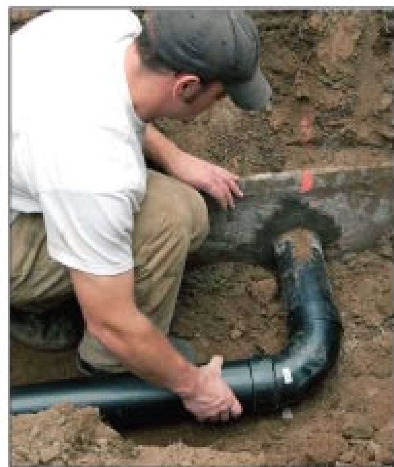
Hammerschmidt plumbs a 4-inch ABS pipe from the existing septic tank's gravity line to the treatment unit.
