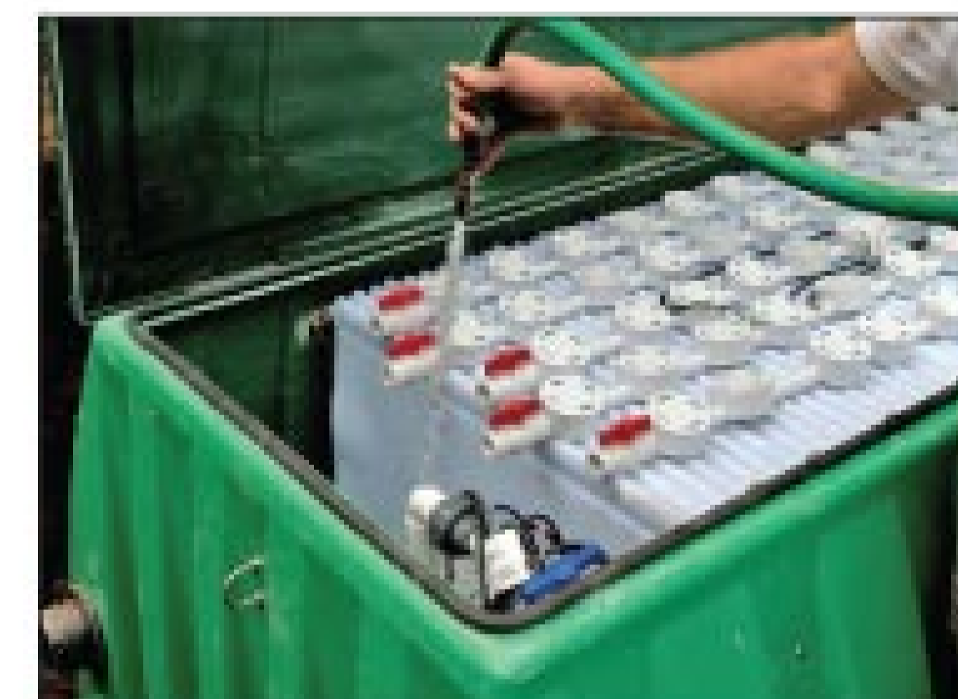
After plugging the inlet, outlet, and vent line, Hammerschmidt fills the treatment unit with water to check for leaks.
