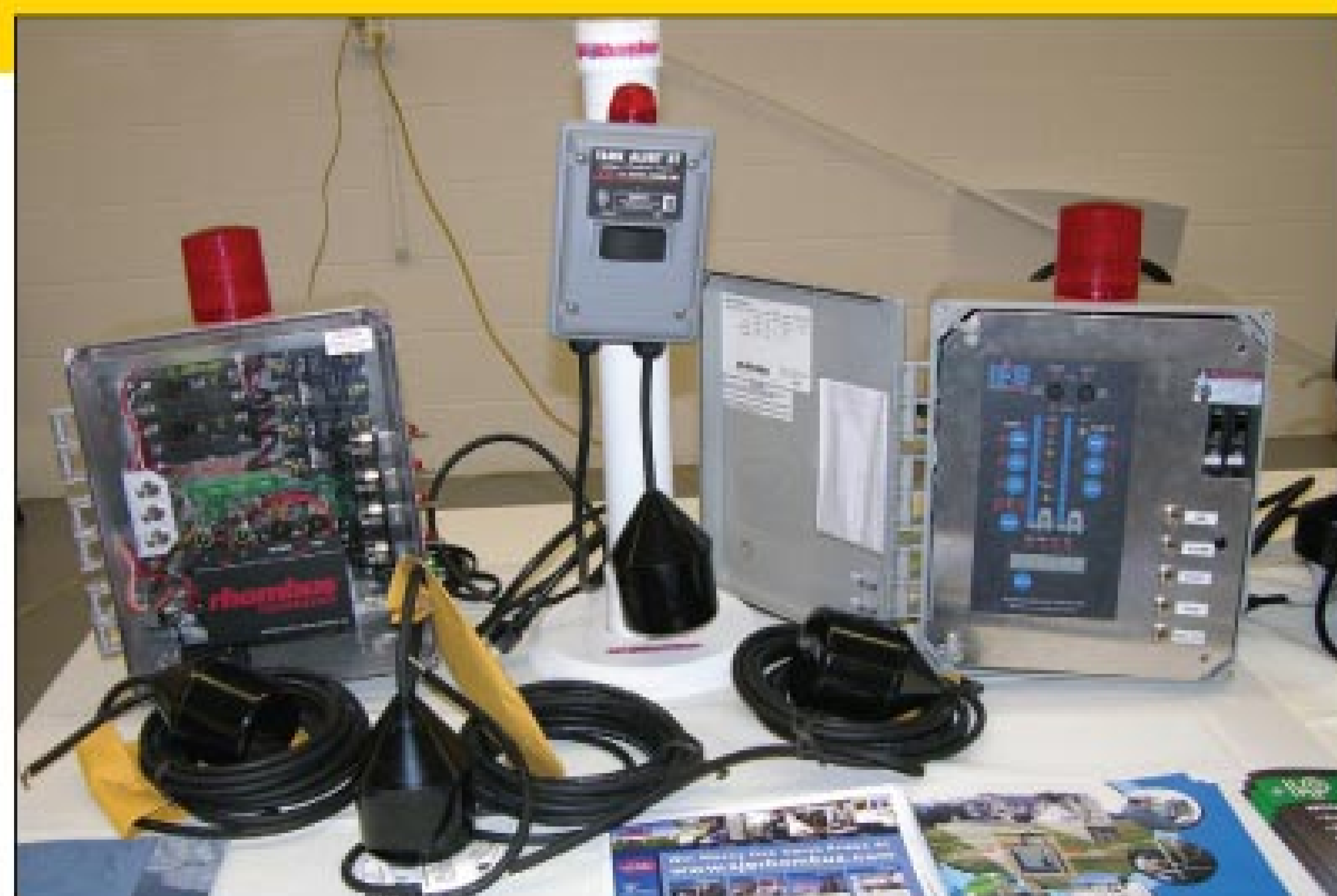
Control floats and control panels with alarms regulate the performance of pumps. Alarms notify homeowners or service providers when failures occur.
