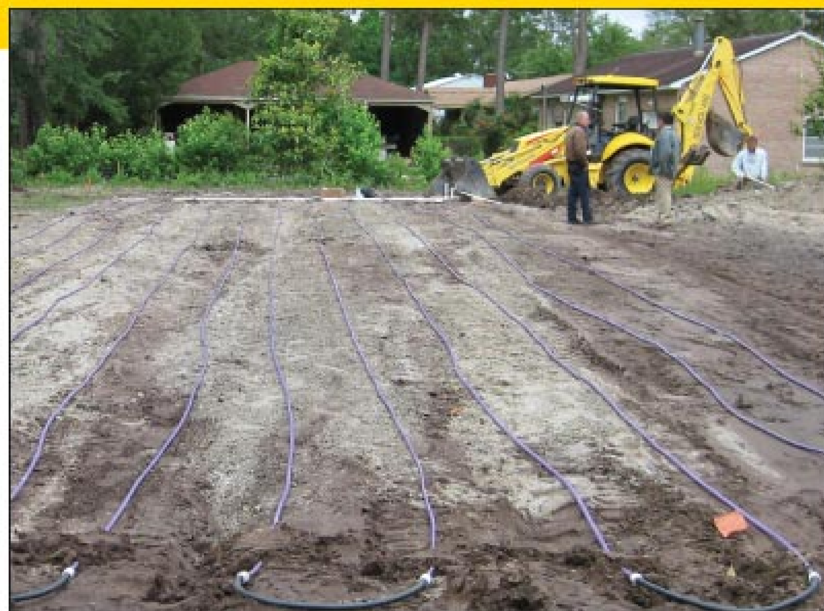
Ernest Rentz (left) and two employees inspect a newly excavated supply trench from the Perc-Rite filtration unit to the drip-zone manifold. (Photos courtesy of American Manufacturing Company Inc.)
