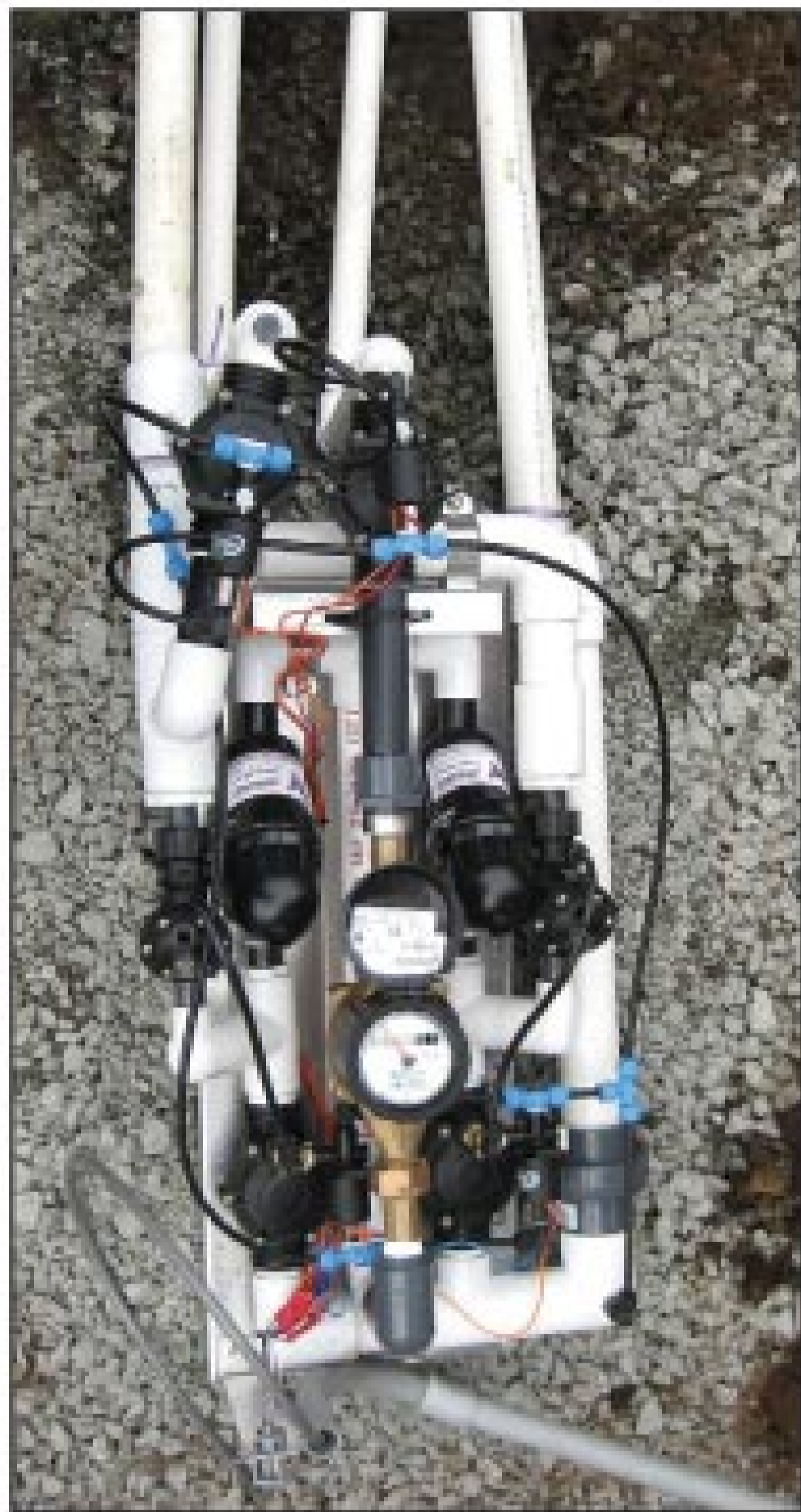
The Perc-Rite hydraulic filtration unit sits on a gravel bed.
