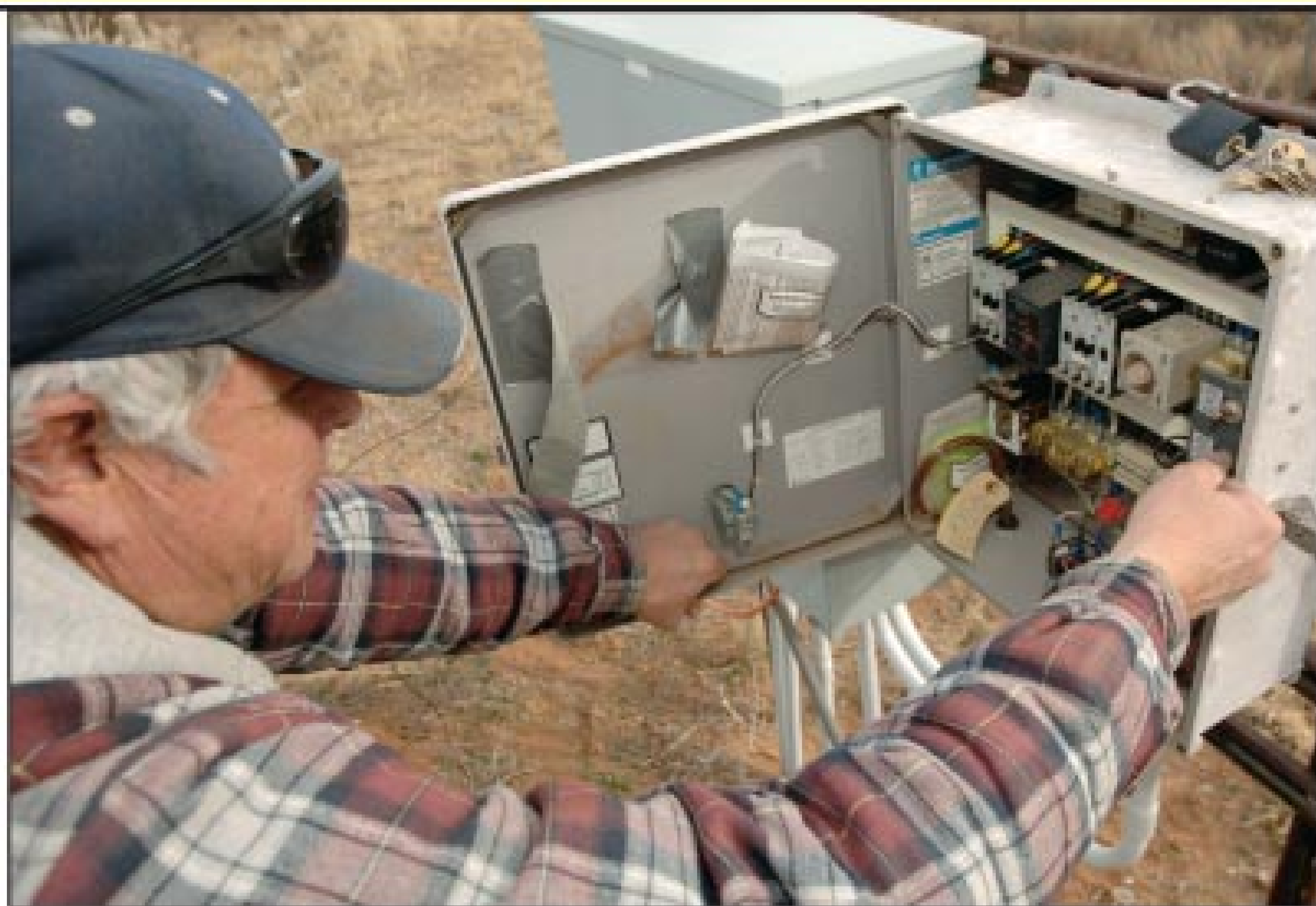
Gene Bassett works on the control panel for a Nibbler treatment unit, manufactured by Aqua Test Inc., on a commercial installation for a small shopping center.
