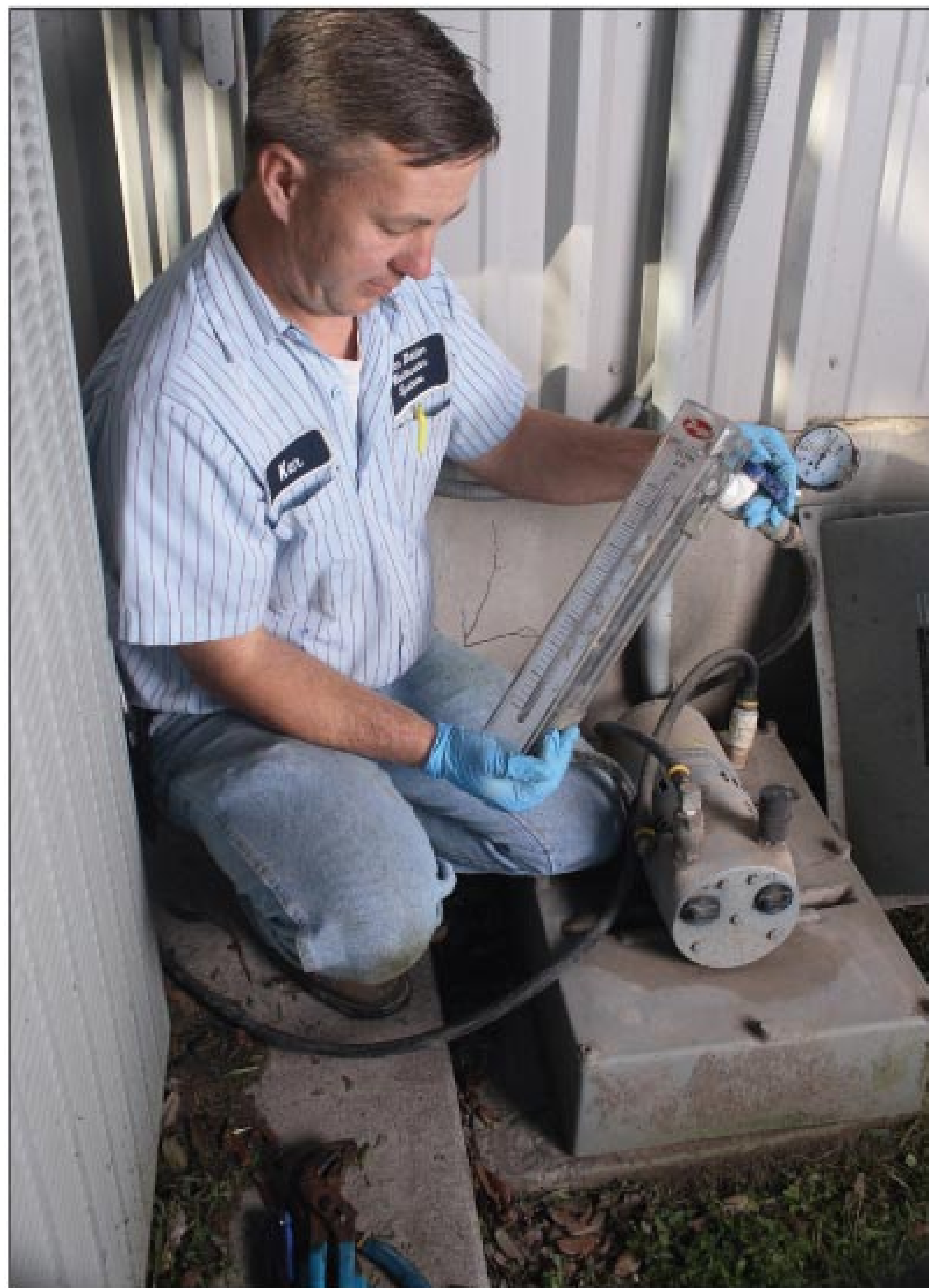
Service technician Ken Munson uses a flowmeter from Dwyer Instruments Inc. to check the airflow volume on an aerobic treatment unit.
