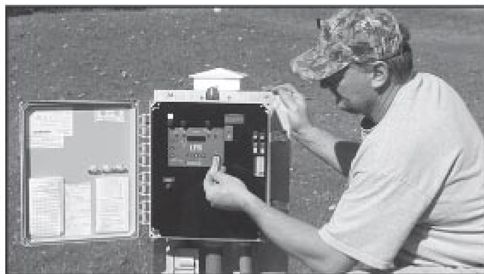
IFS In-Site® Event Monitoring Control Panel
