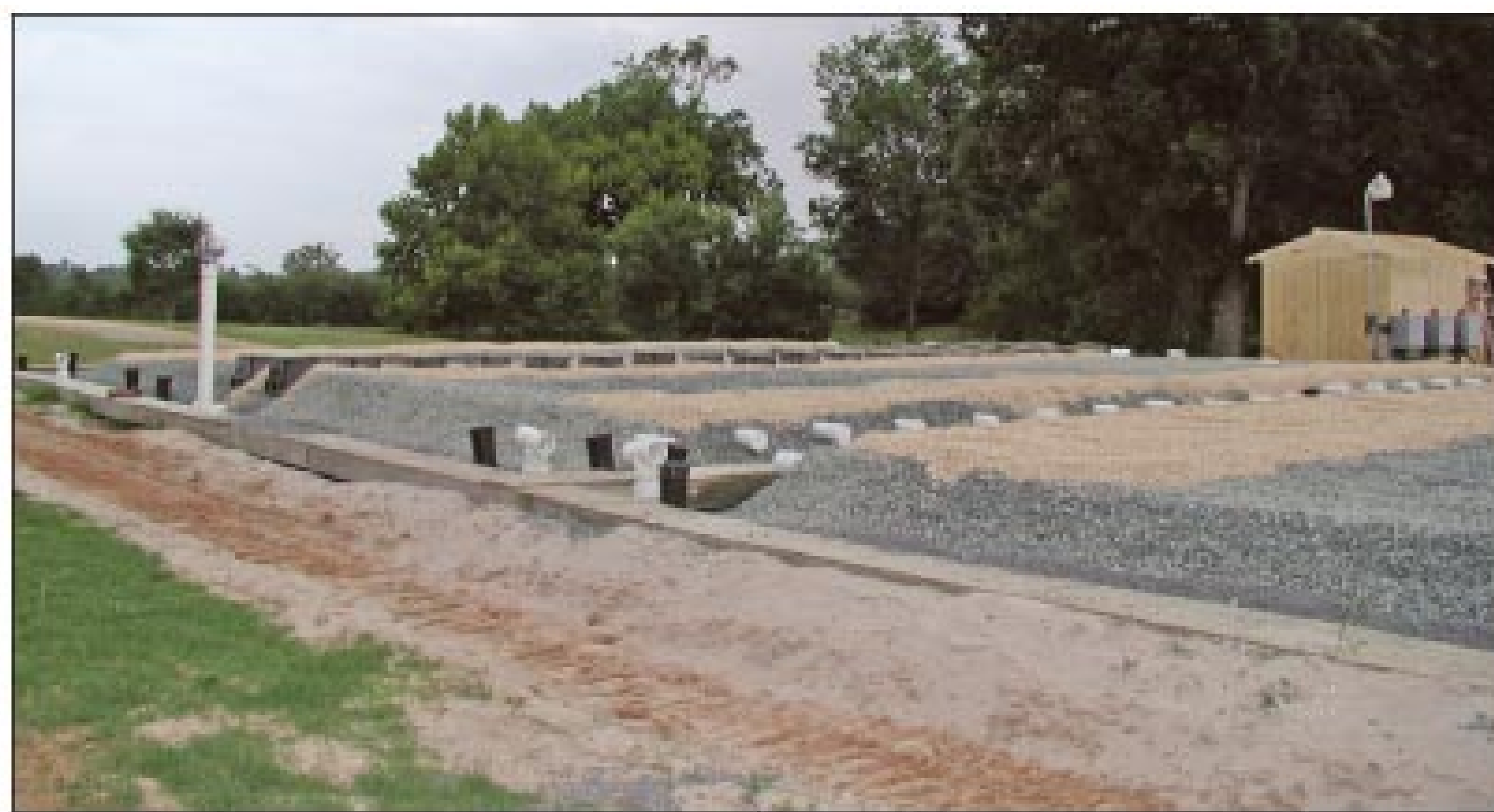
The sand filters with a partial cover of 5/16-inch Stalite.
