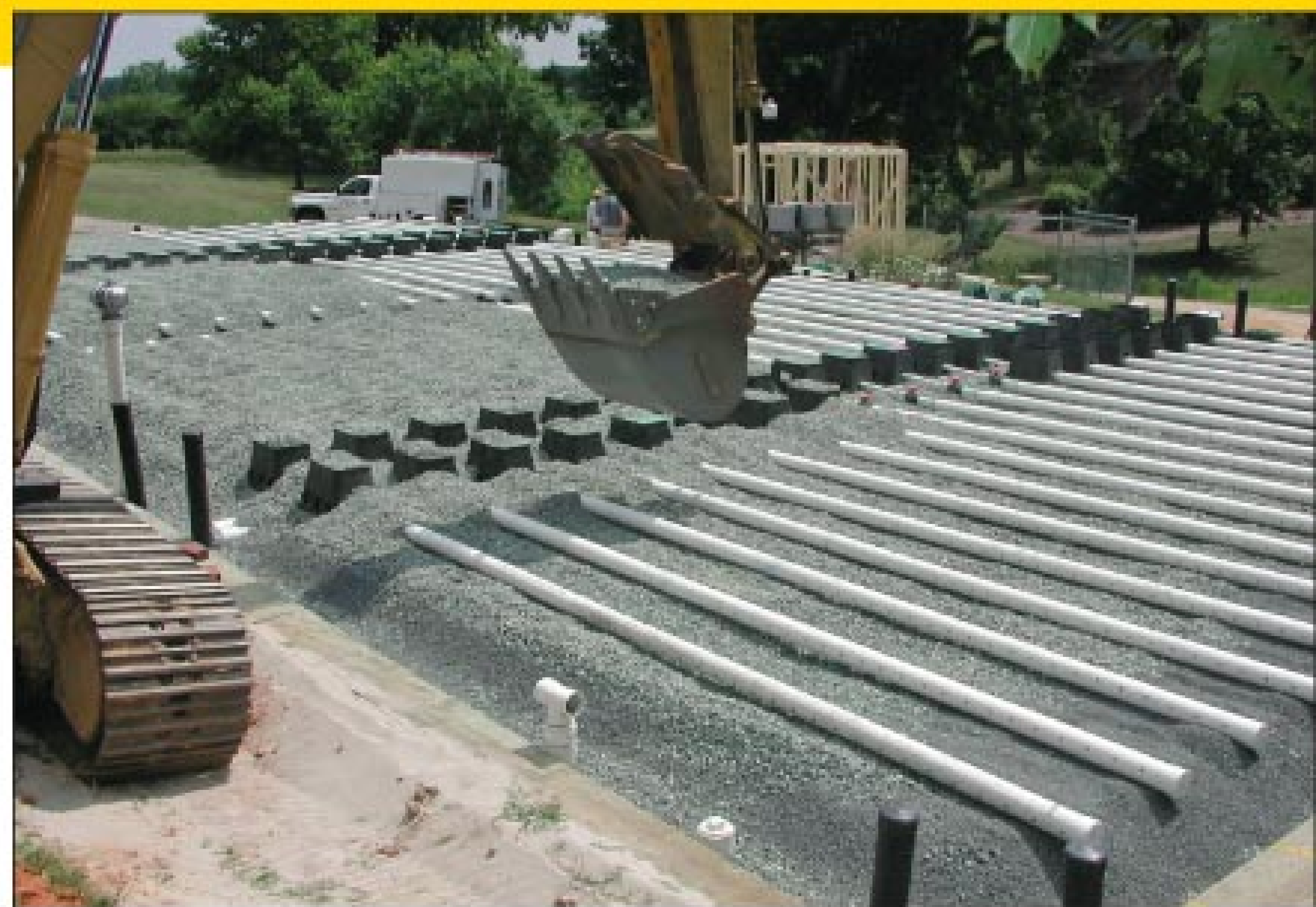
The excavator operator covers the sleeved 1.25-inch low-pressure distribution lines with 1/4-inch pea gravel 2 inches deep. Each sand filter has two rows of 18 laterals, 20 feet long on 2-foot centers with individual observation ports in the middle. In the background is the framing for a maintenance building. (Photos courtesy of Integrated Water Strategies)
