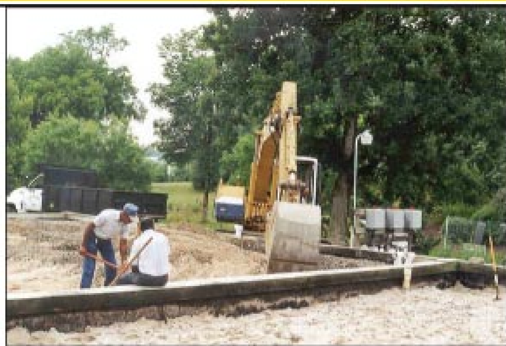
The excavator operator removes 2 feet of sand and gravel from one of two masonry block boxes containing the original sand filters.
