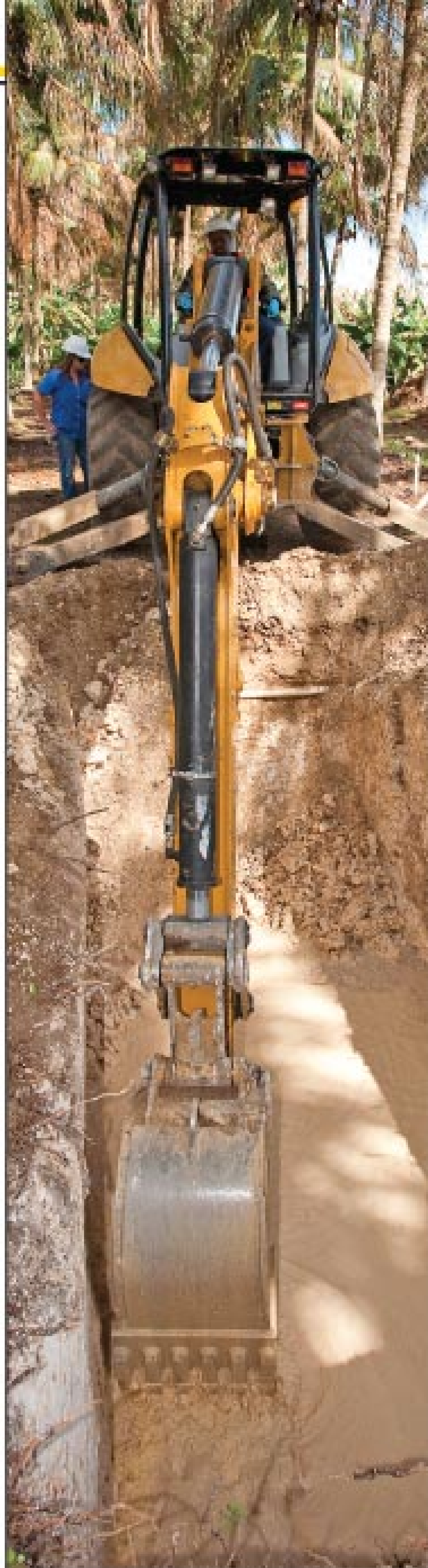
Anthony Sweat uses the company's Caterpillar 430E backhoe to dig the hole for a septic tank. The company's service area includes lands underlain by "bedrock" that is actually coral from the floor of ancient oceans.
