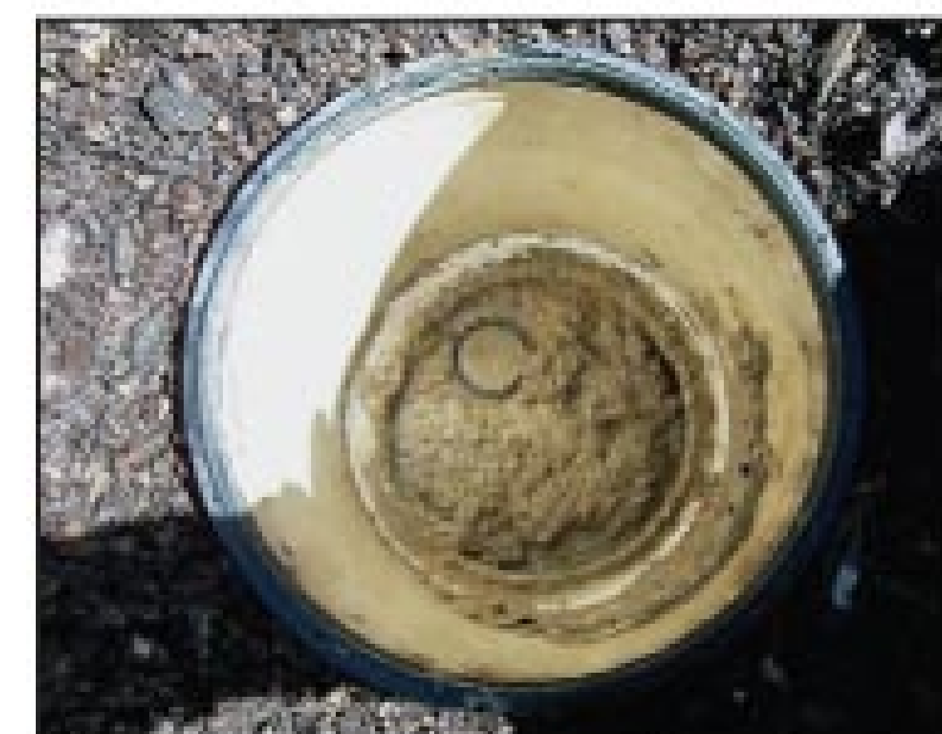
Scum caused by fats, oils and grease (FOG).
