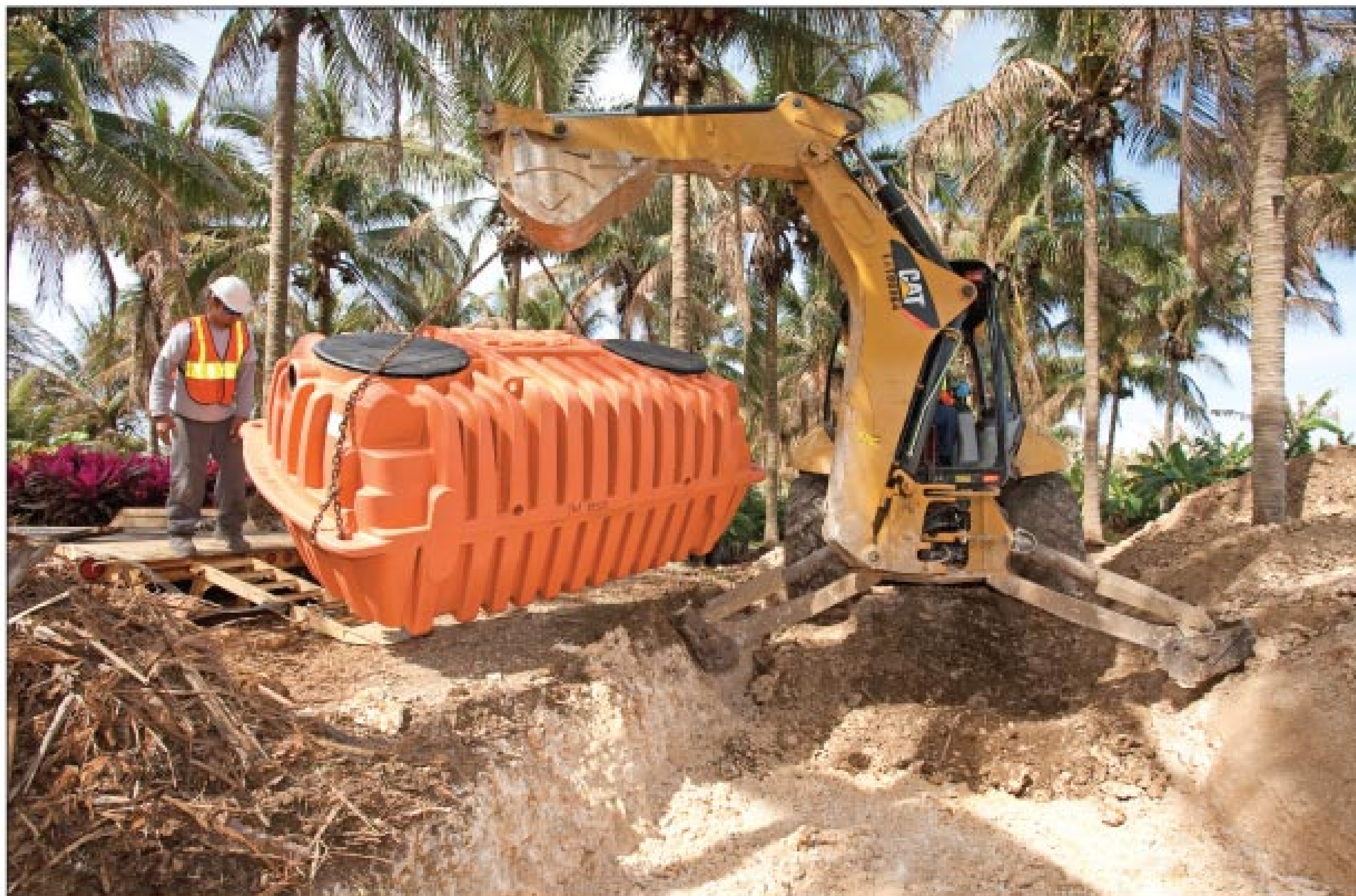
The team prepares to place a plastic septic tank from Infiltrator Systems Inc.
