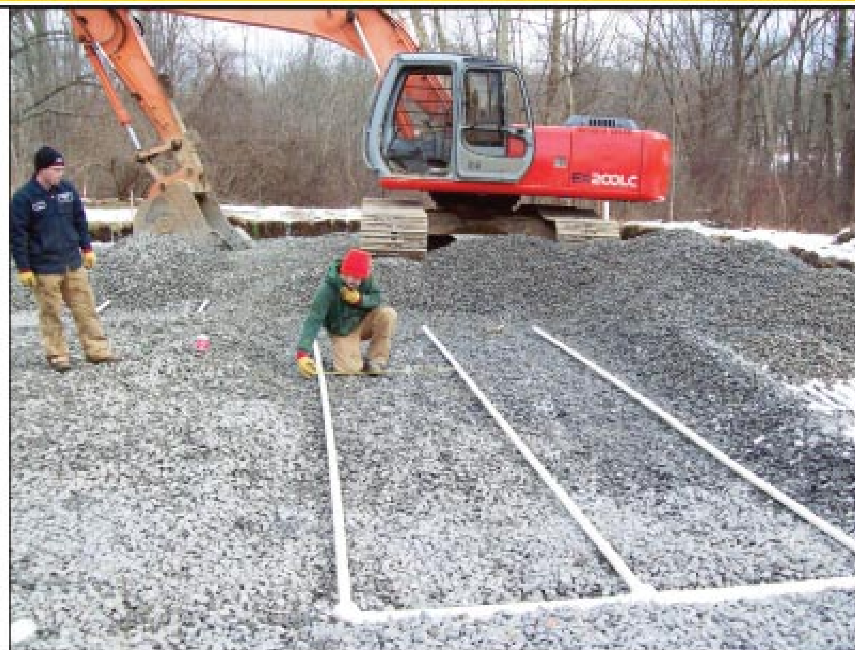
Bob Jewell Jr., measures the distance between laterals to ensure that they are on 3.75-foot centers. Chris Hovencamp observes. The EX 200LC Hitachi excavator is parked at the far end of the drainfield.
