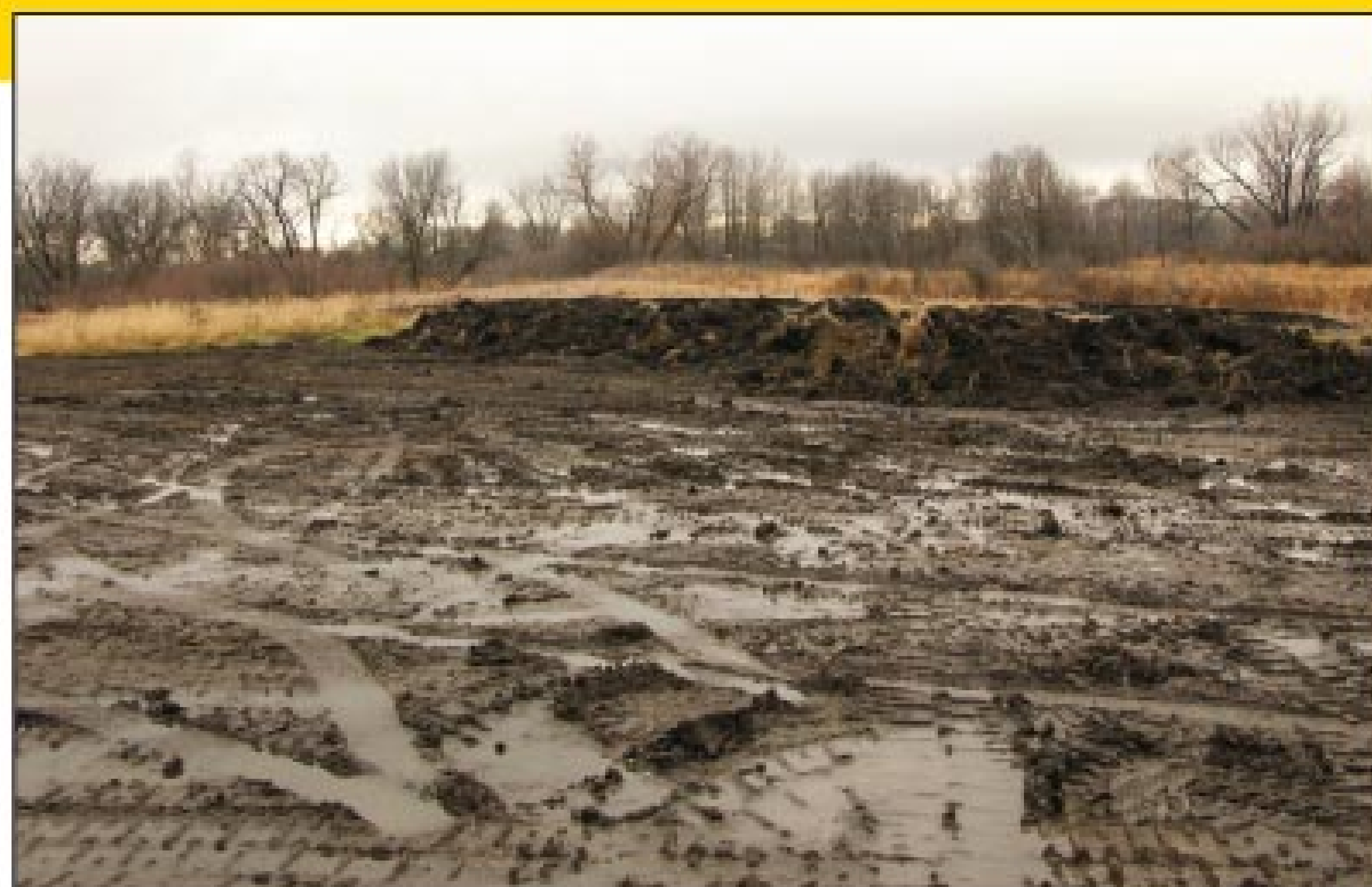
Here is an example of how not to prepare a surface for an aboveground onsite treatment system.
