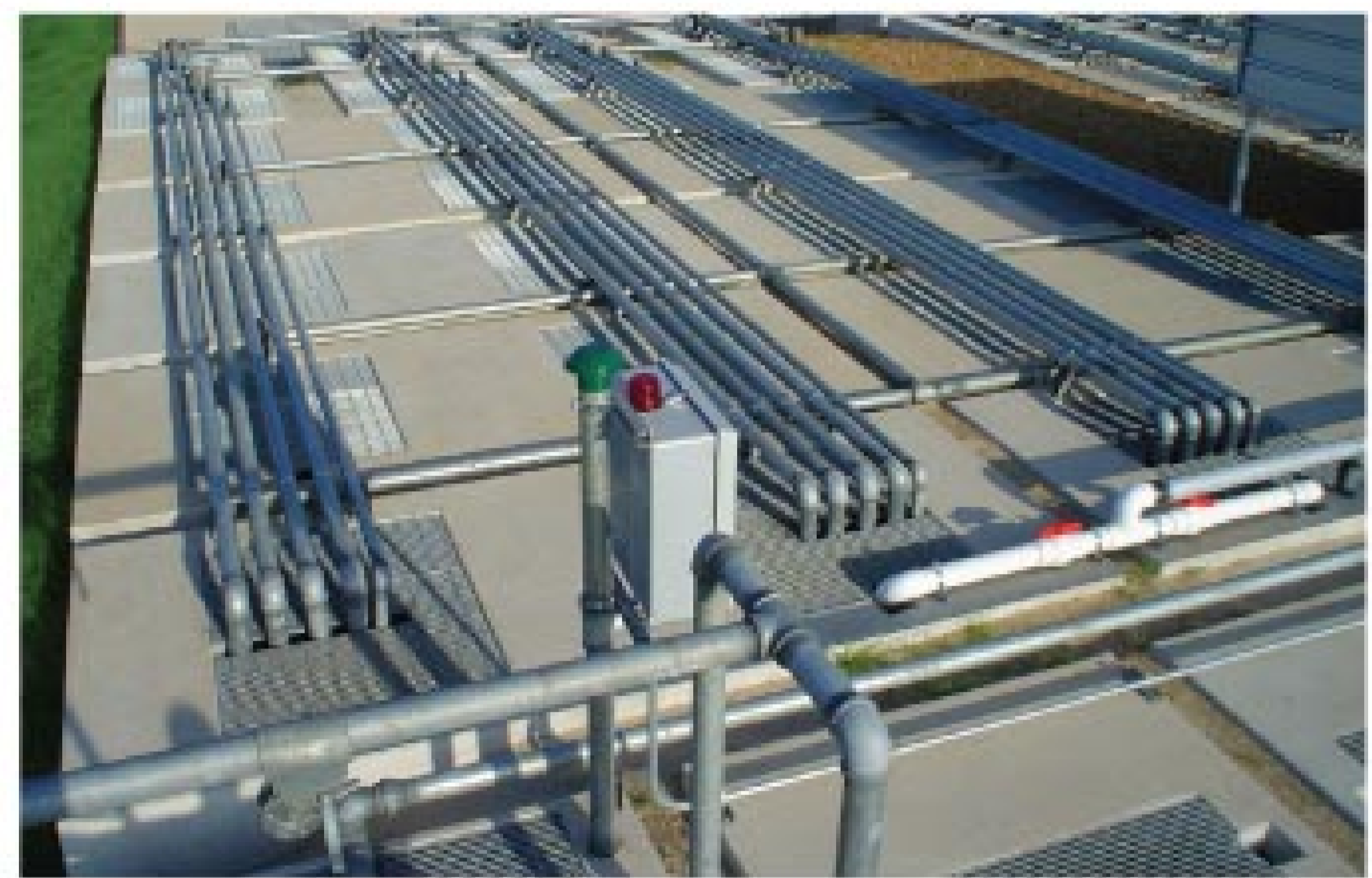
120,000 GPD system for a 300-home subdivision.
