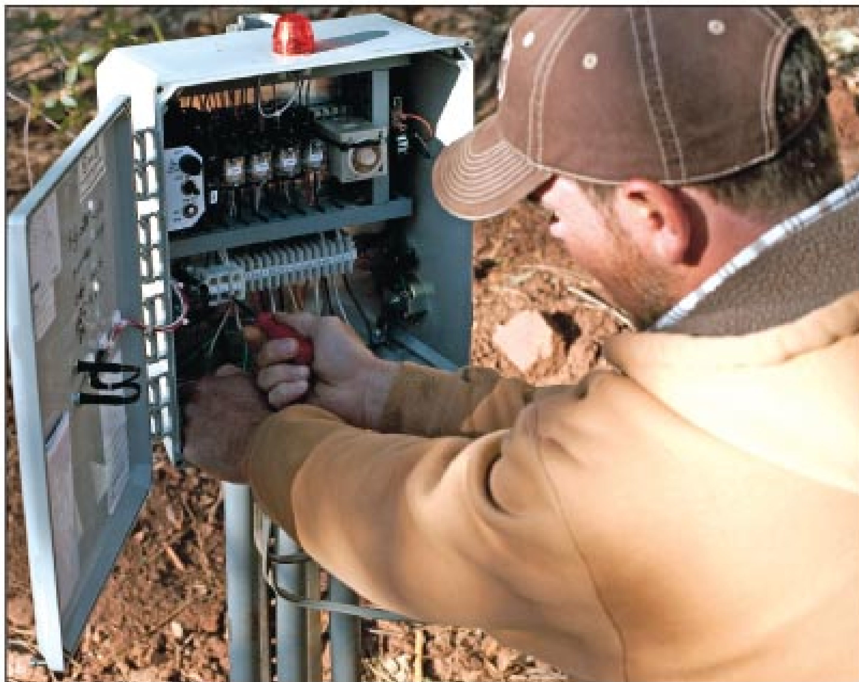
Owner Levi Brownlee builds his own control boxes for use on a variety of onsite systems.
