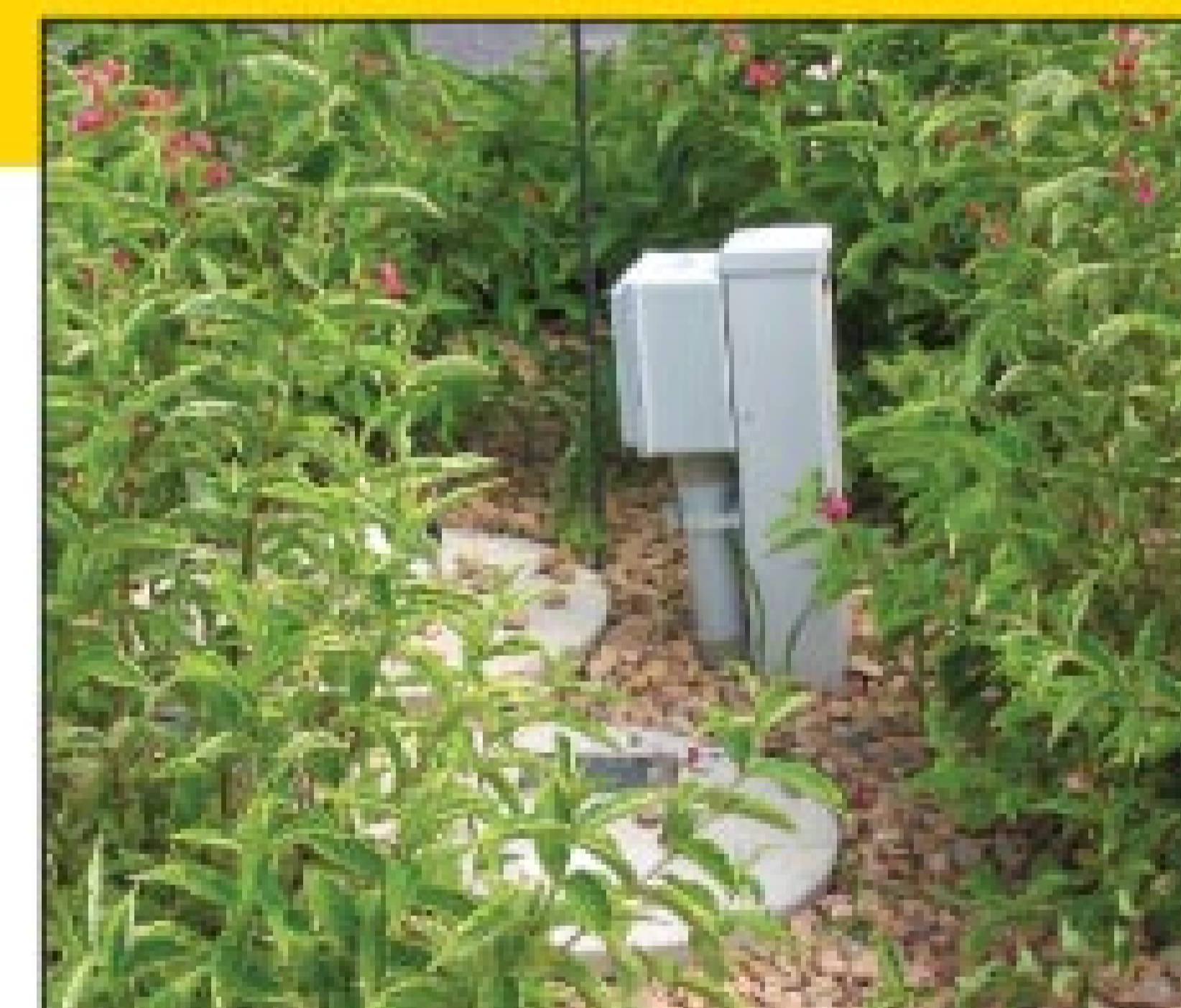
An example of a good wiring installation with the wiring box outside the pump station.
