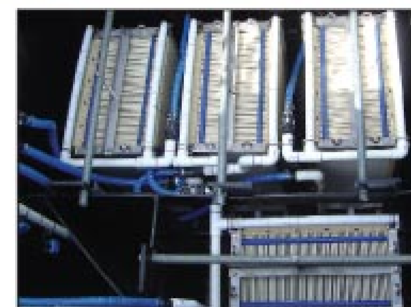
Four microfiltration flat-sheet membrane modules in the bioreactor for the Grizzly Bear system screen solids through pores of 0.03 to 1.1 microns. A piping system attached to each module transfers permeate to a tank in the control room.
