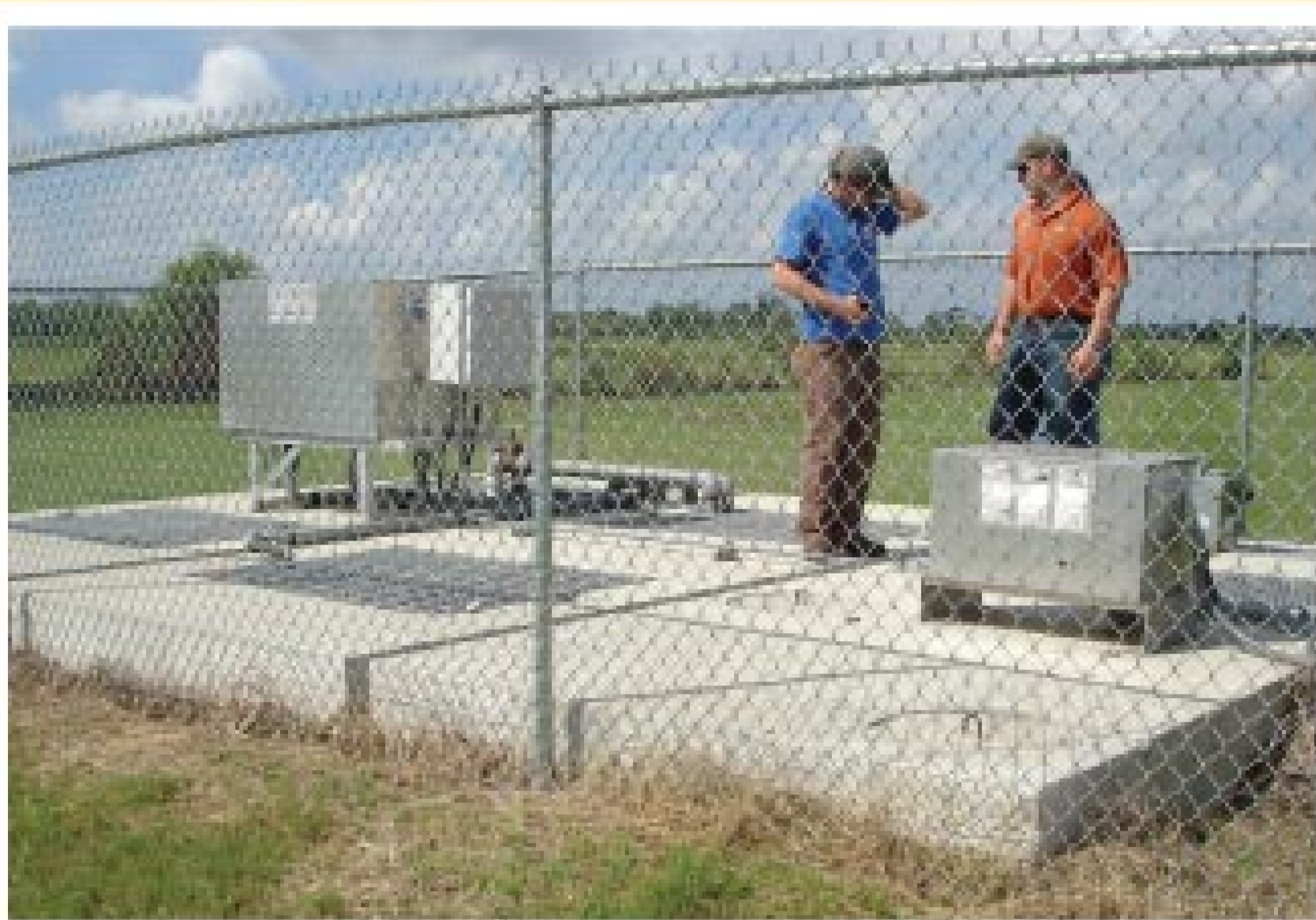
10,000 GPD system at a school.
