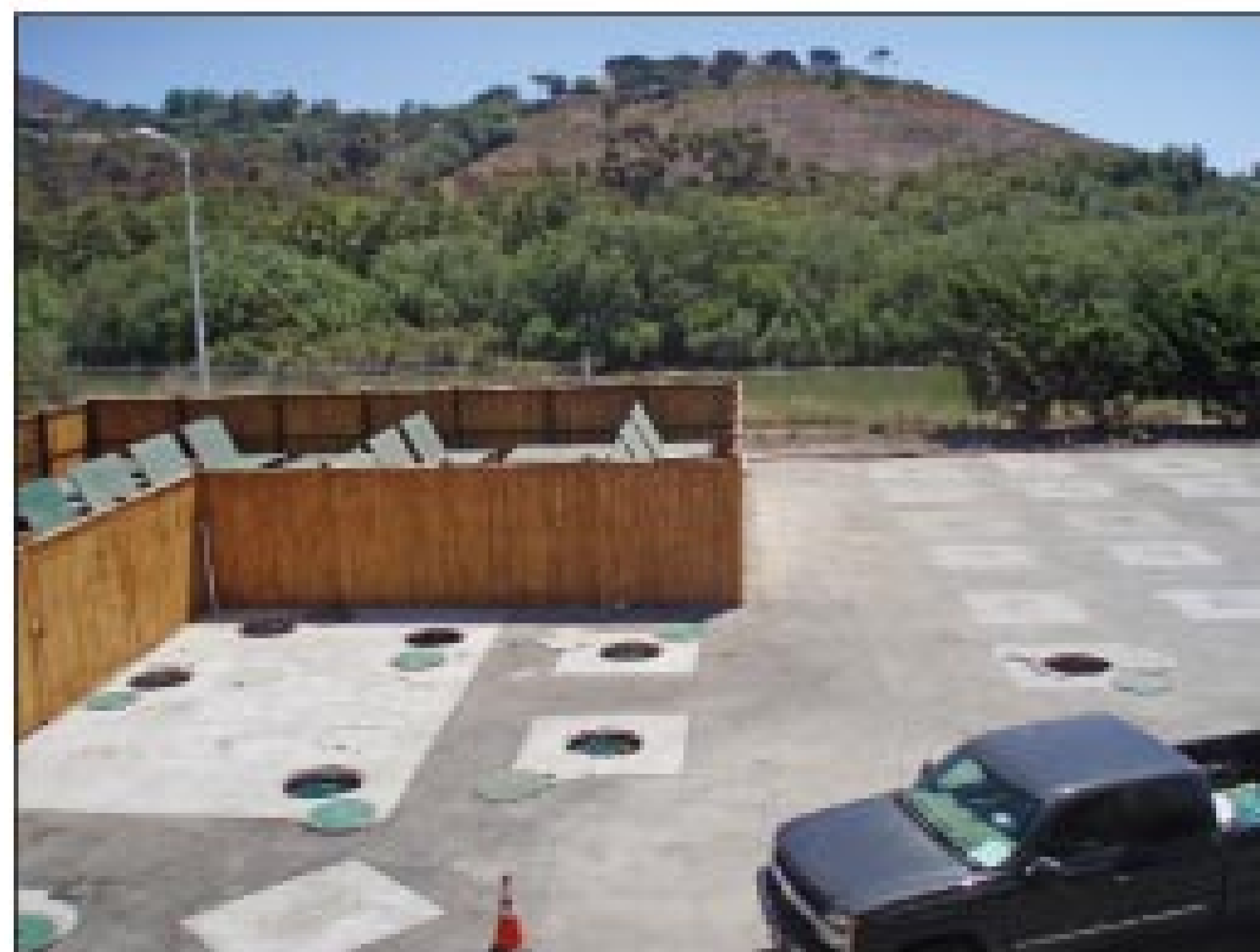
Onsite system from Lombardo Associates Inc.
