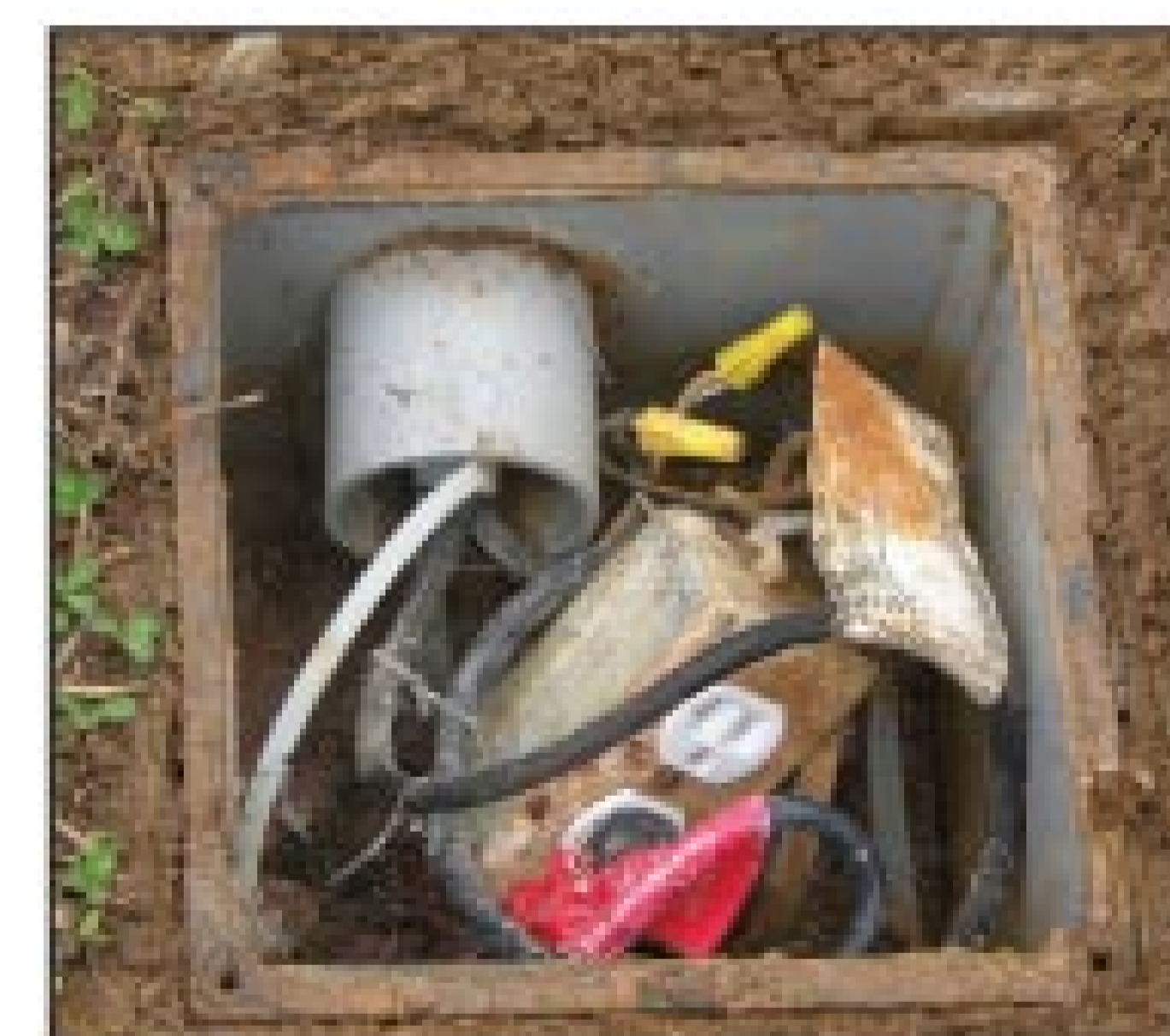
An example of the right idea, but poor execution. The wiring box is not watertight or sealed.
