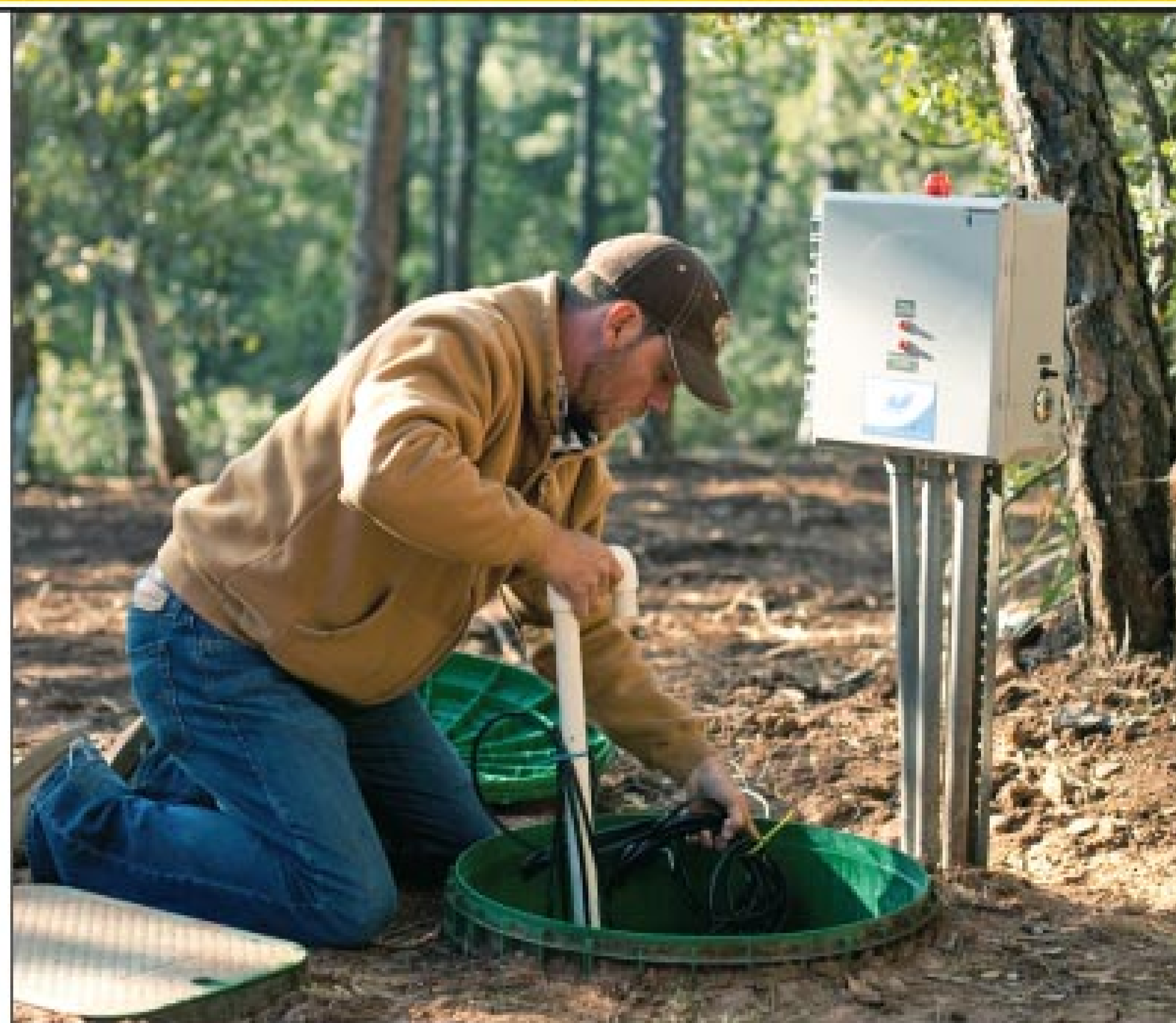
Levi Brownlee checks the control floats in a pump chamber tank.
