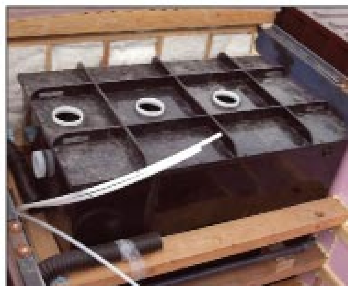
An extrusion welded insulated membrane tank in a compartment for the Denali River Cabins system.
