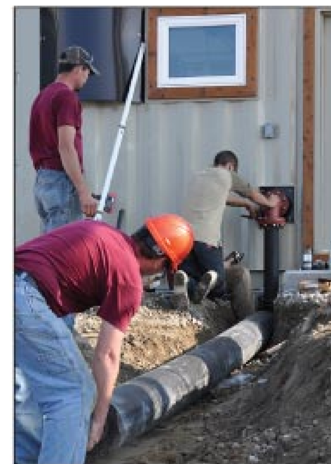
COURTESY OF LIFEWATER ENGINEERING CO.
