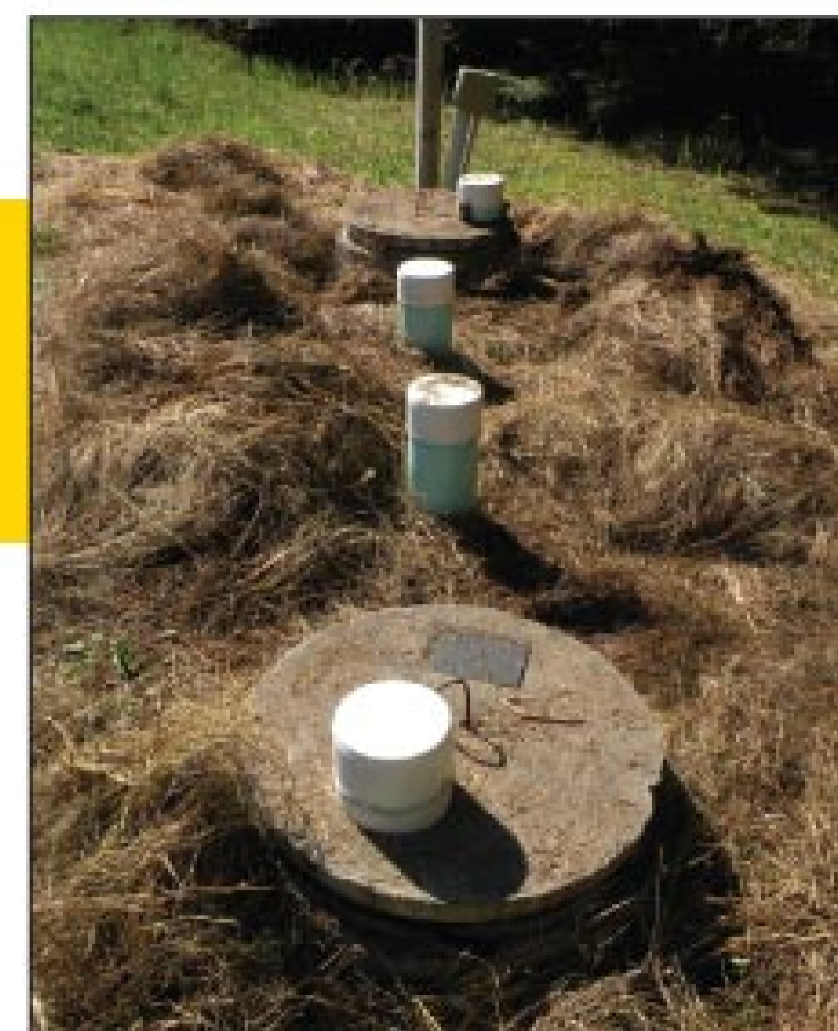
Covers brought to the surface can be a source of odors if not properly sealed.
