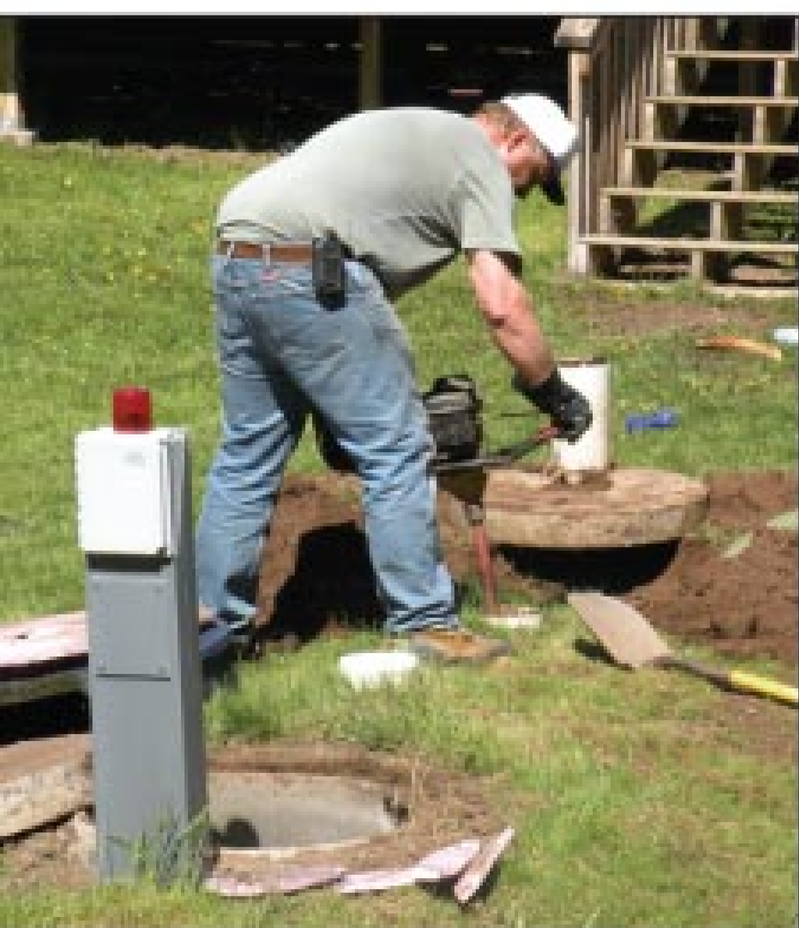
Odors may be present just after cleaning of the septic tank.
