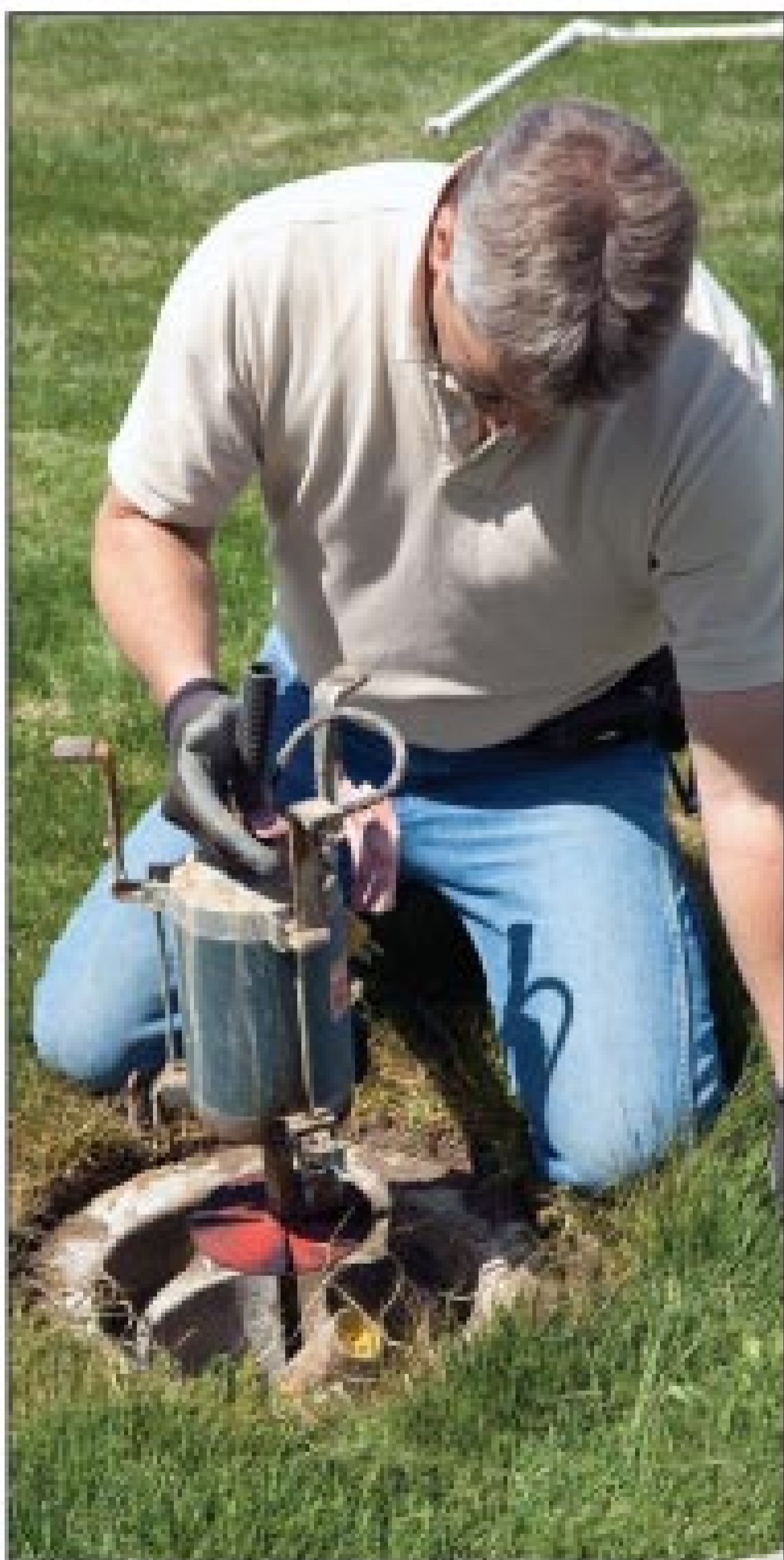
Walker services a treatment system from Jet Inc.
