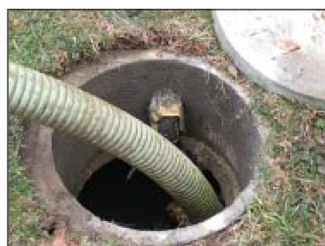
Good septic tank maintenance is a part of any restoration strategy.
