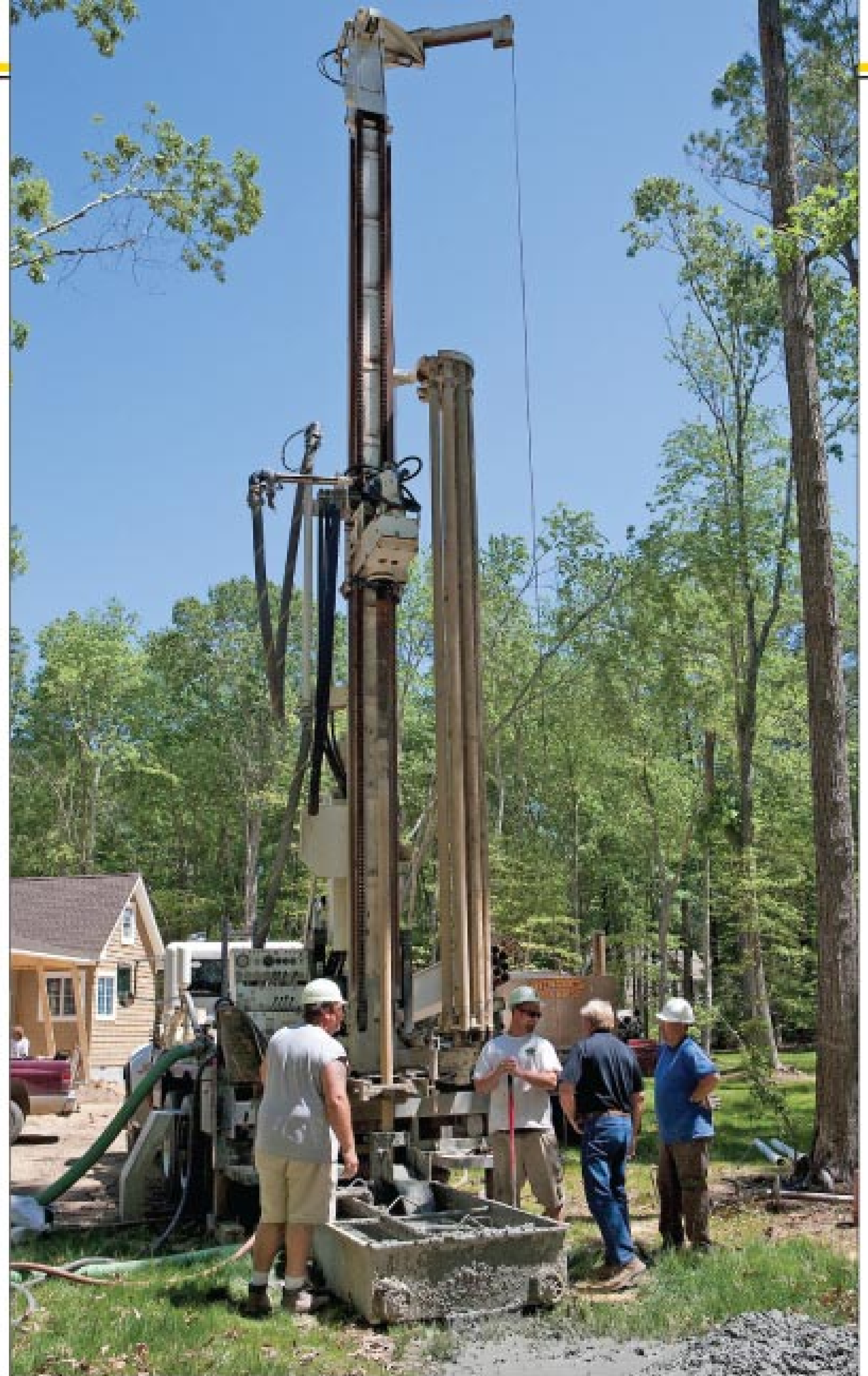
Jimmy Bundick checks in with employees Jerry Fisher and Jason Cooper and well driller Barron Justice on a residential well-drilling job.
