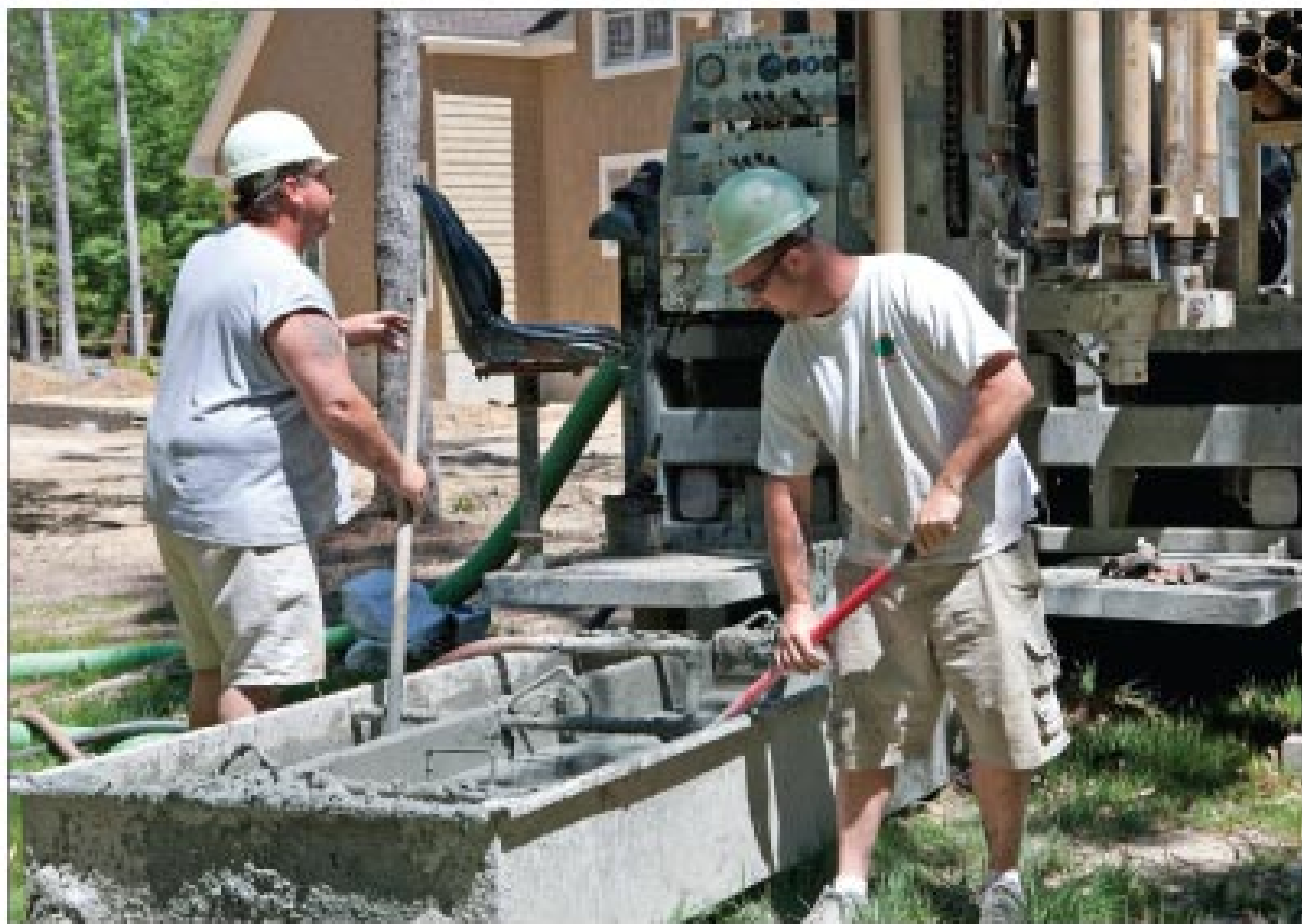
Well driller and drill supervisor Jerry Fisher and well driller assistant Jason Cooper work on a domestic water well, drilling more than 250 feet.
