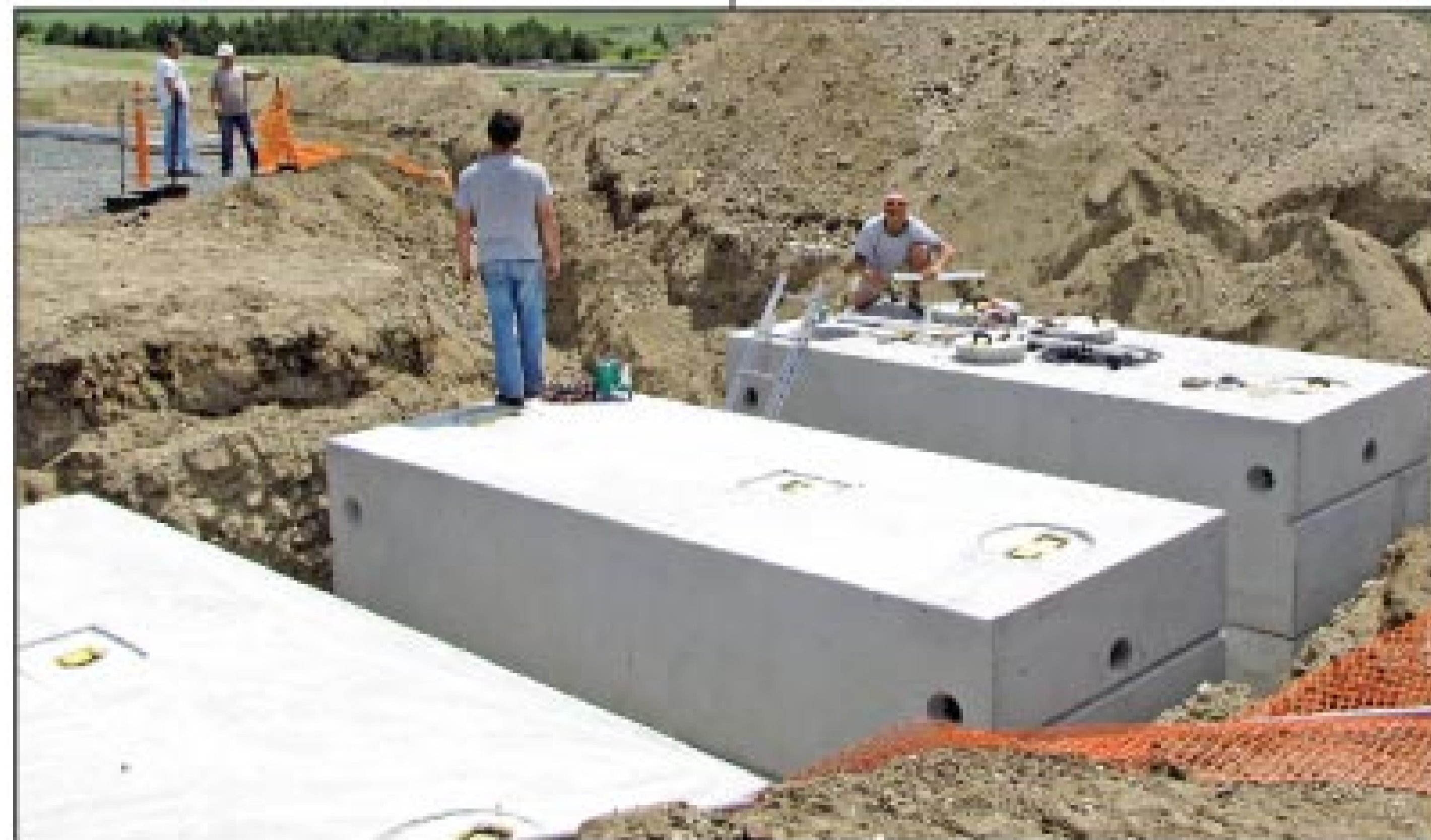
The two 2,400 gallon septic tanks are in the foreground; the Eliminite fixed-film bioreactor tank is in the background.
