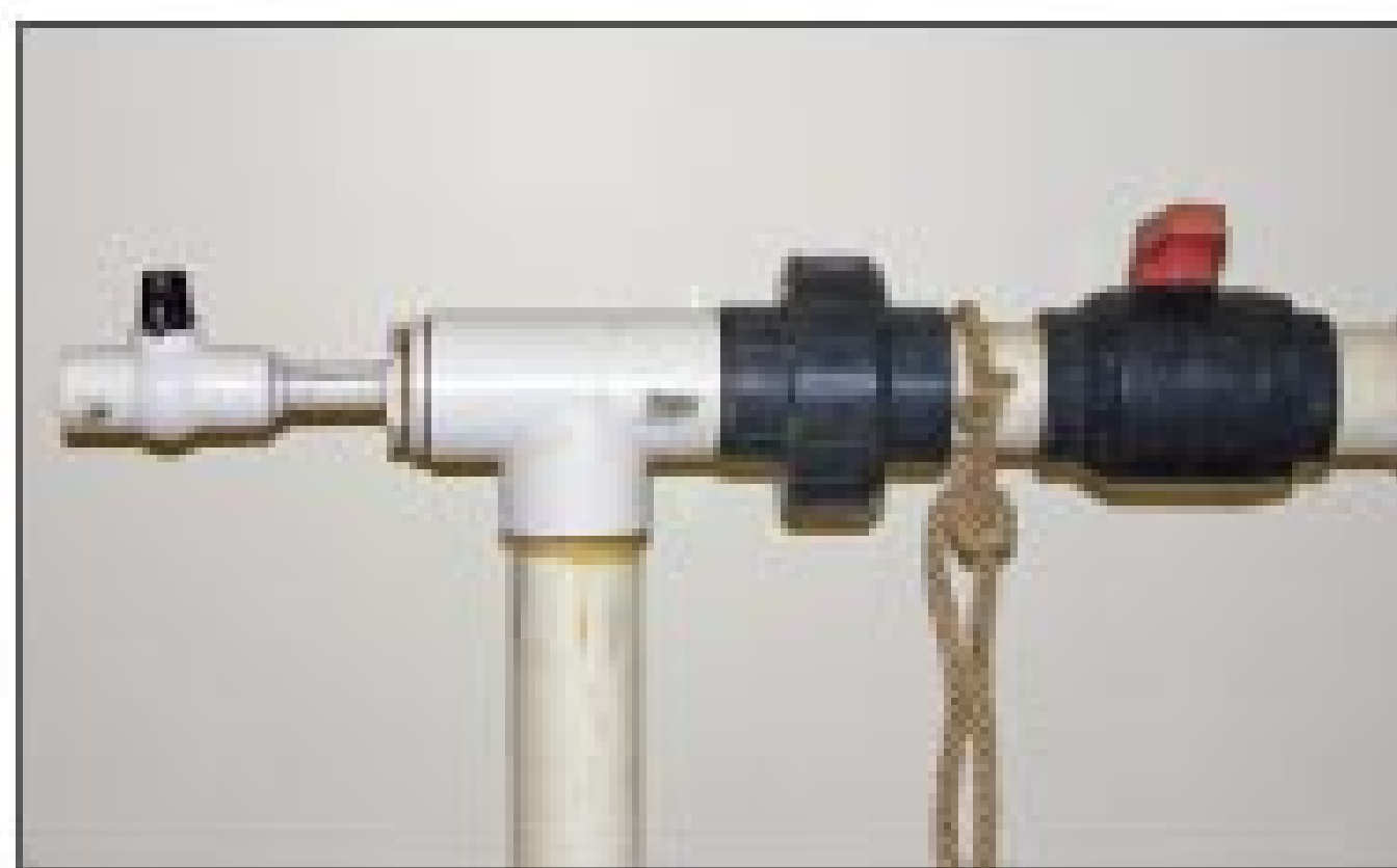
An example of a quick disconnect to remove pumps.
