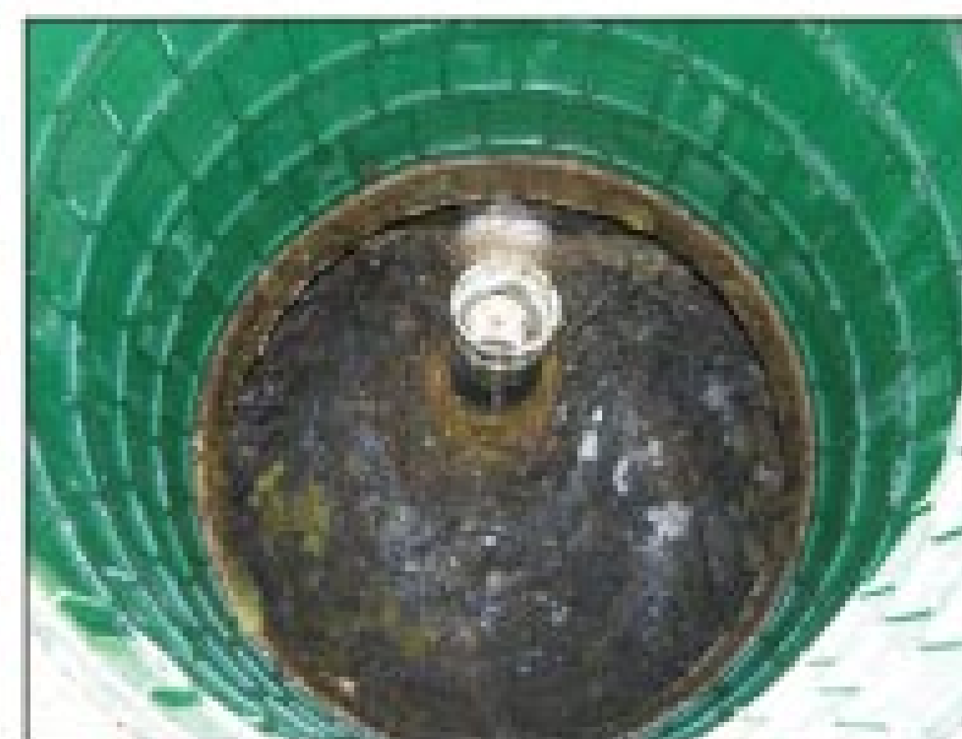
Risers provide easy access to tanks for maintenance.
