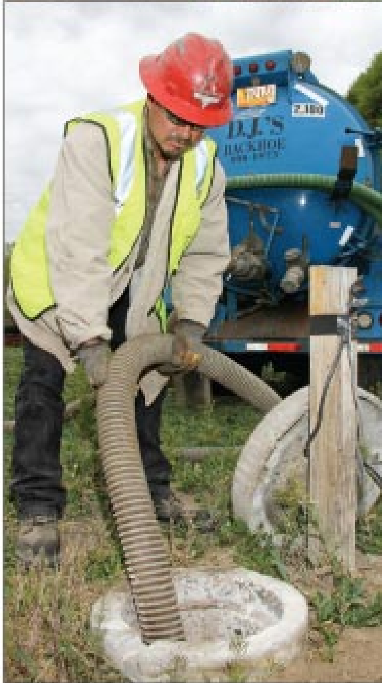
Rodriguez Verela pumps a septic system. Company owner Don Moats Sr. got his start in the pumping side of the onsite industry.
