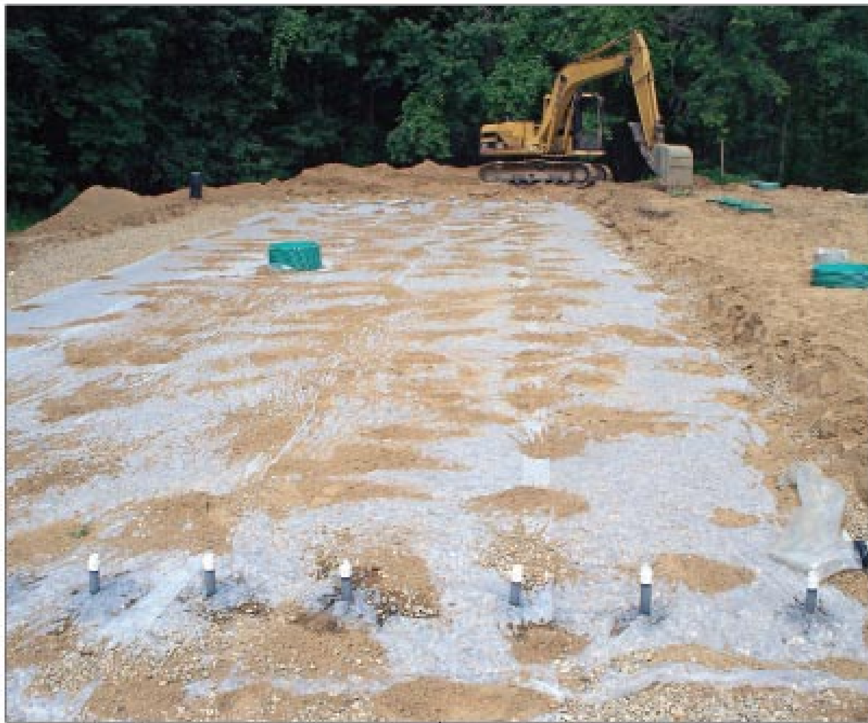
COURTESY OF WRAY'S SEPTIC TANK CO.
