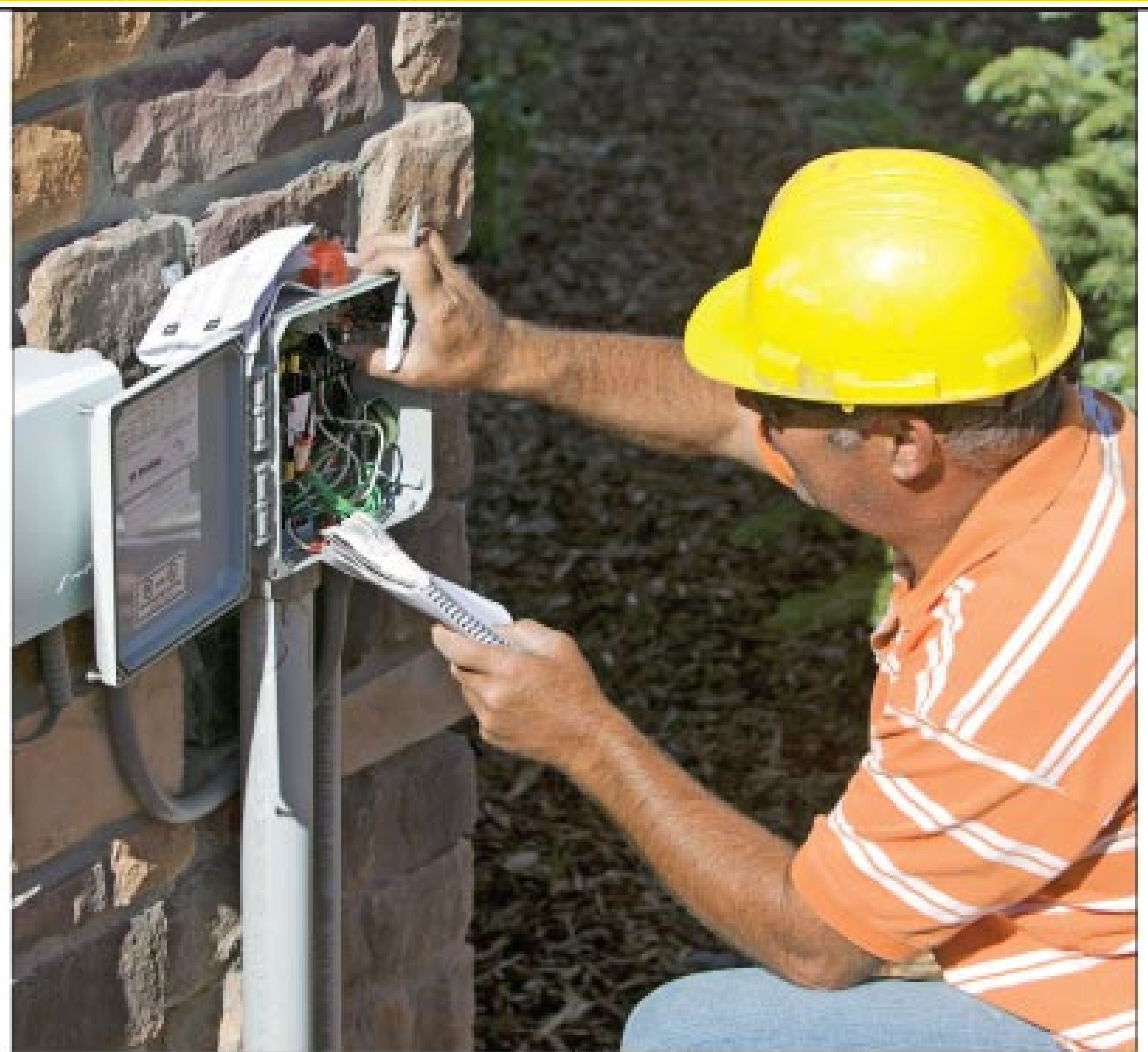
Johansson checks an SJE-Rhombus control panel and records dose cycles while making a service call.
