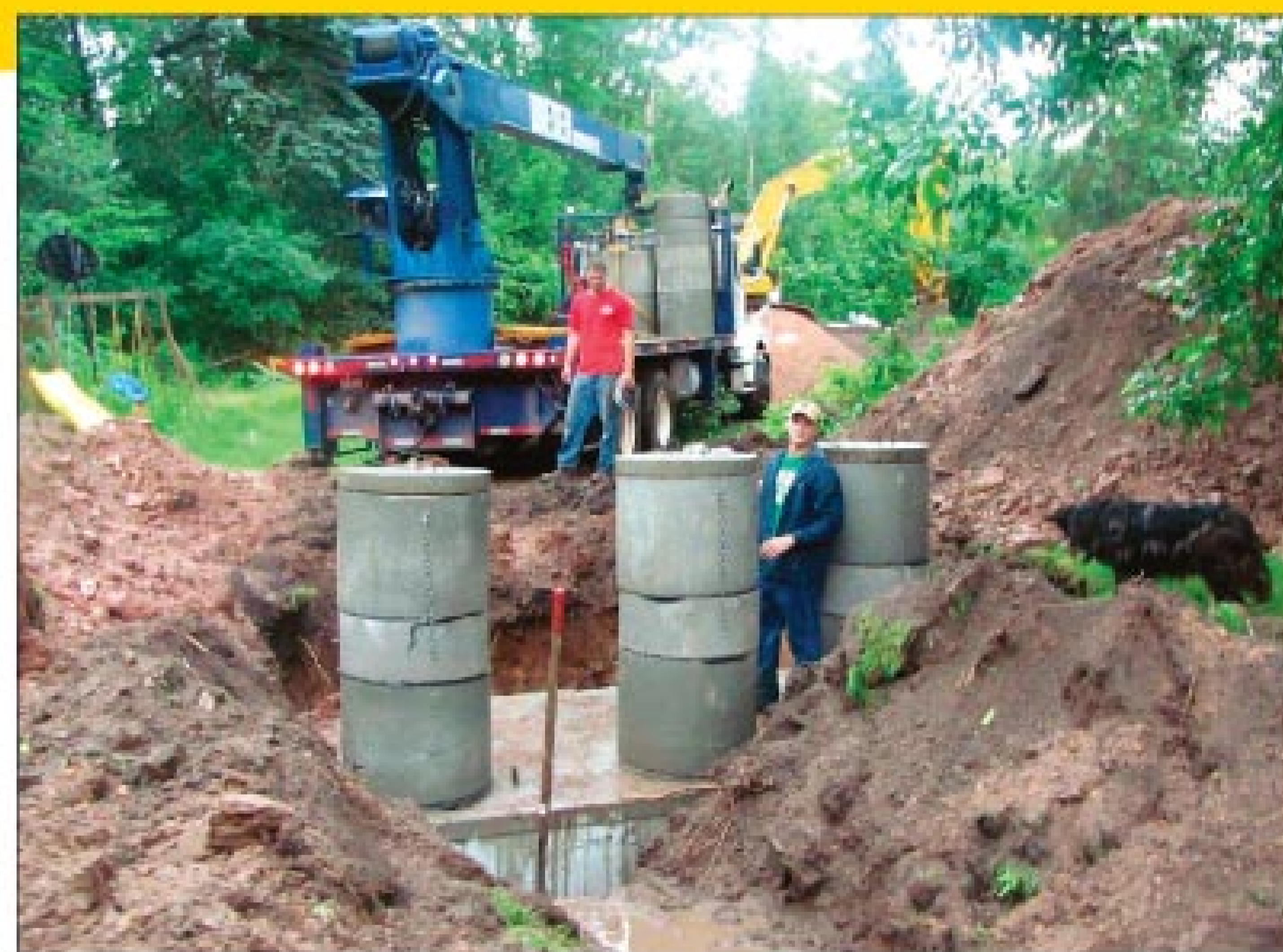
Shawn Hoppwood, left, from Wieser Concrete and Jake Baudhuin from Baudhuin Engineering set the 5-foot-tall risers on the 1,800/1,100-gallon triple septic tank. (Photos courtesy of Brown Plumbing and Heating)
