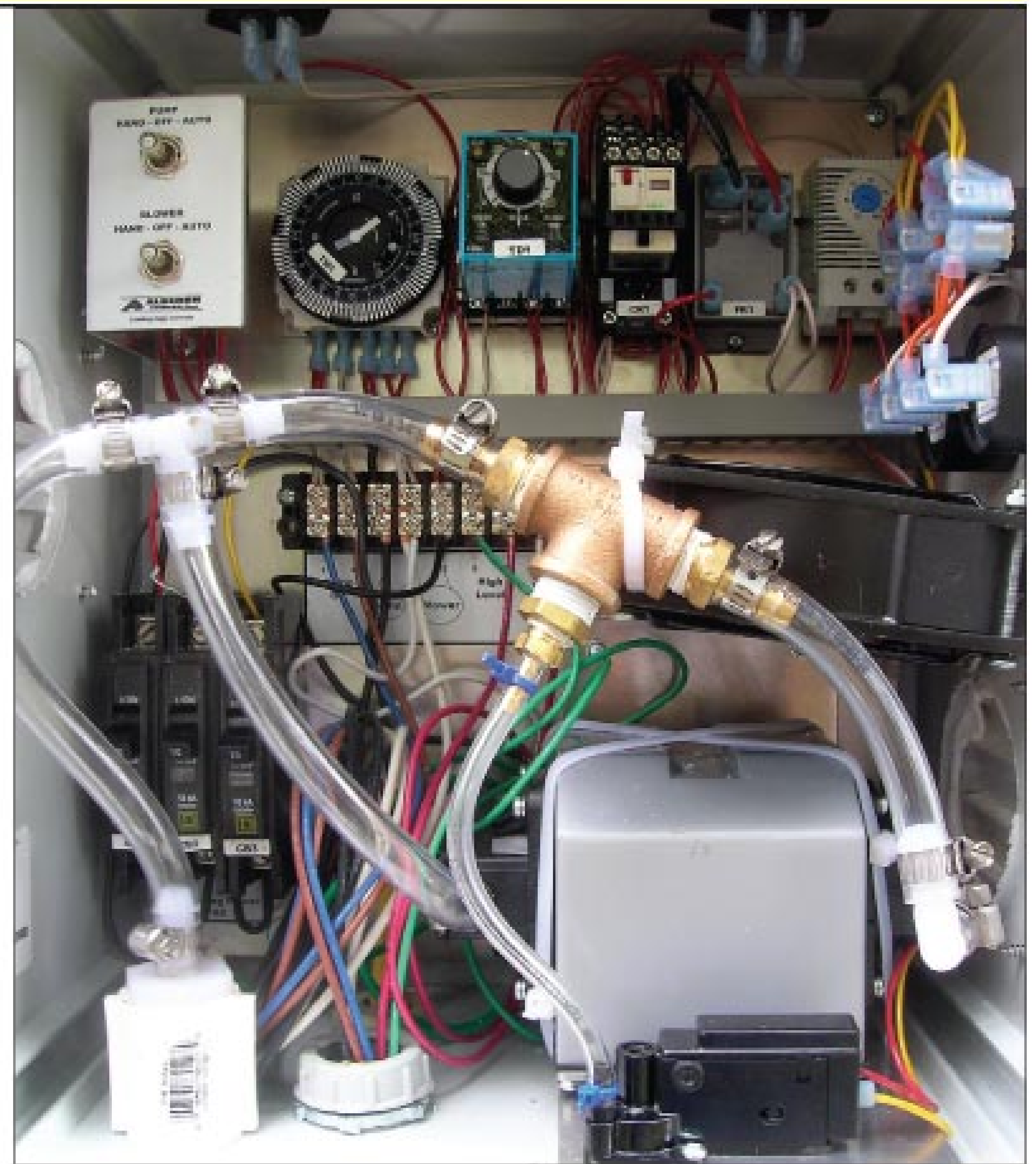
The control panel has a 24-hour timer for the aeration cycle, a timer to delay the discharge pump operation until after the settling cycle, a pressure switch and alarm to monitor the air pump operation, a tank high-water alarm, an air pump and discharge cycle override, and a thermostatically controlled ventilation fan to cool the air pump.
