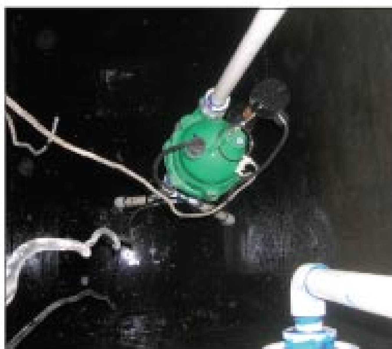
The effluent pump, supported on three 1-inch PVC legs, sends clarified water from the top quarter of the tank to the drainfield.
