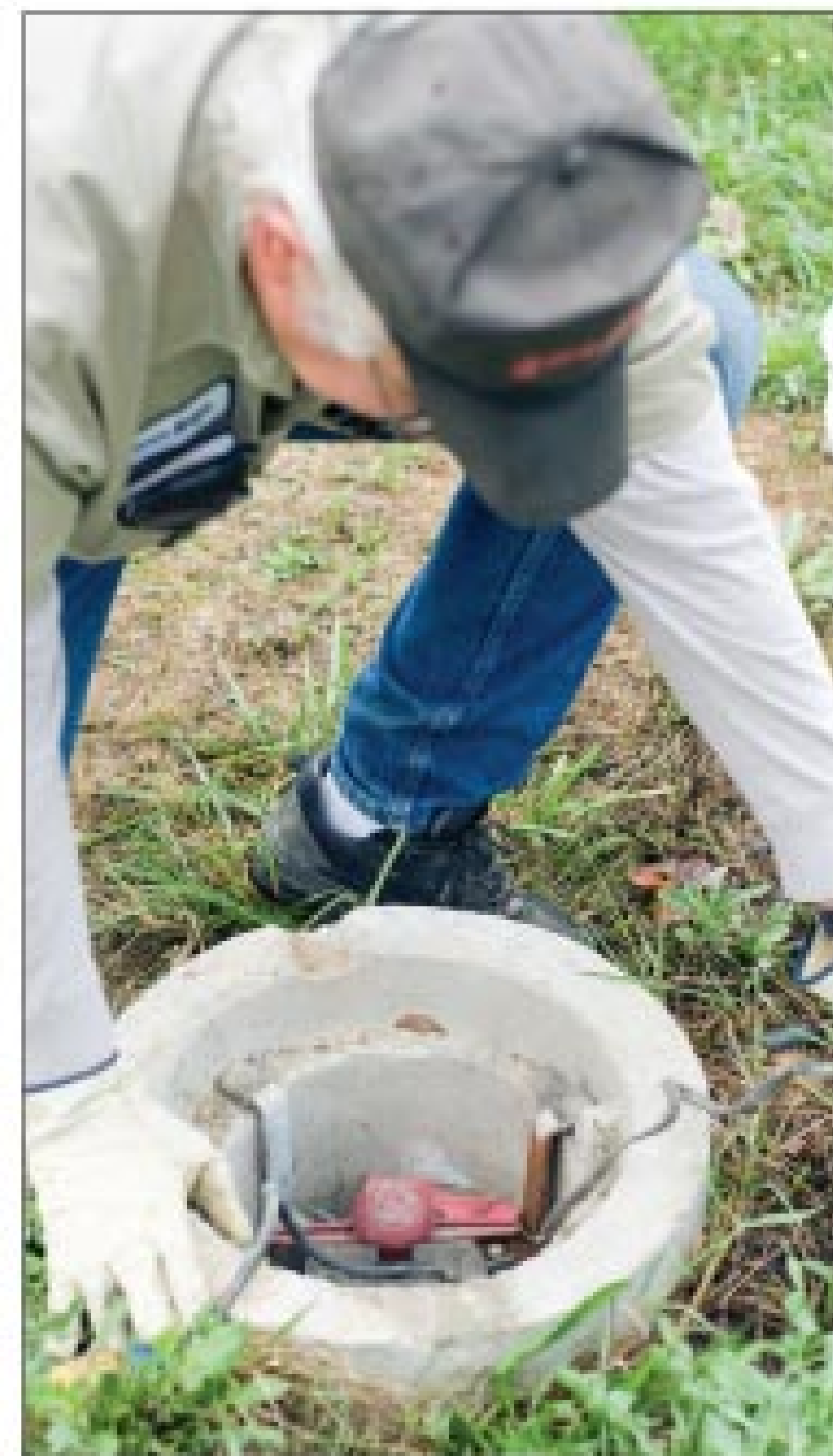
Service manager Jim Bagwell checks the aerator in a residential treatment unit from Jet Inc.
