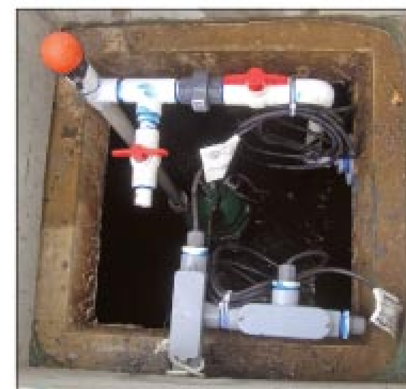
The air line and conduit are in the foreground. In the background, an air-vacuum valve (red circle) prevents air binding and water siphoning from the tank if the pipe should become surcharged. A disconnect union (gray fitting) allows the pump to be removed, and a check valve (red right) prevents backflow.
