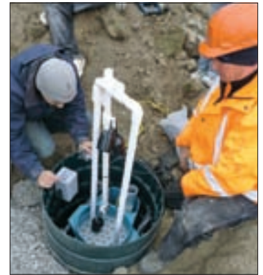
Étienne Bordeleau (left) and Kirk Hastings verify the placement of the Biotube pump vault and final location of the float level alarms.
