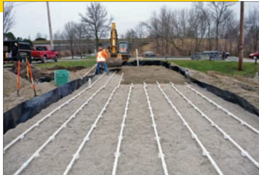
Kirk Hastings adds the final layer of aggregate above the distribution piping while his assistant rakes and levels it. (Photos courtesy of Centre for Sustainable Watersheds)
