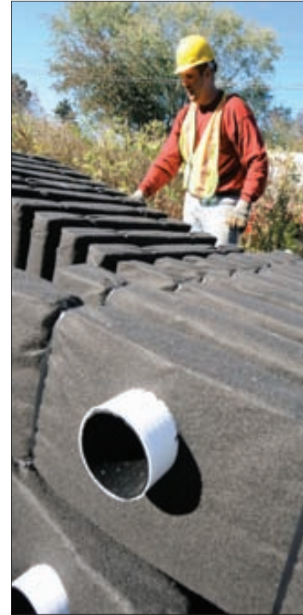
Jason Walter moves a Mantis GSF leaching unit from Eljen Corporation into place.
