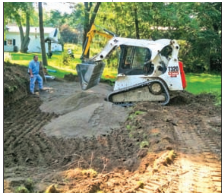
A Bobcat skid-steer deposits System Sand on the edge of the treatment site, while the excavator arm spreads it around. Six inches were added to elevate the system 24 inches above water table.
