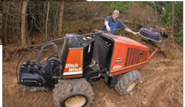
Andy Embry installs drip tubing with a Ditch Witch 410sx vibratory plow.
