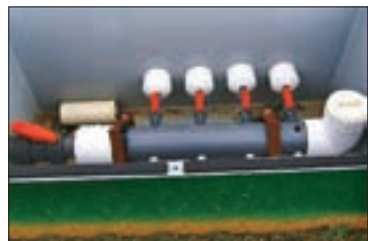
A pressure manifold is another method of pressure dosing to the soil treatment area. (Photos courtesy of Kit Rosefield)
