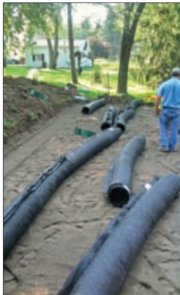
Workers assemble 10-foot sticks of treatment pipe into seven 40-foot-long rows on 18-inch centers. The pipes snap together using a coupler fitting with a tab and slot.
