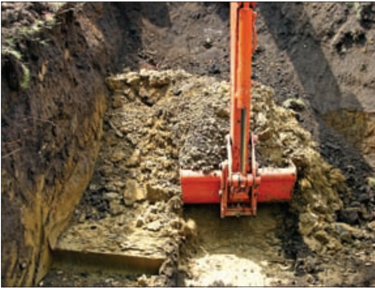
Excavating to a level base allows for the tank to stay watertight.
