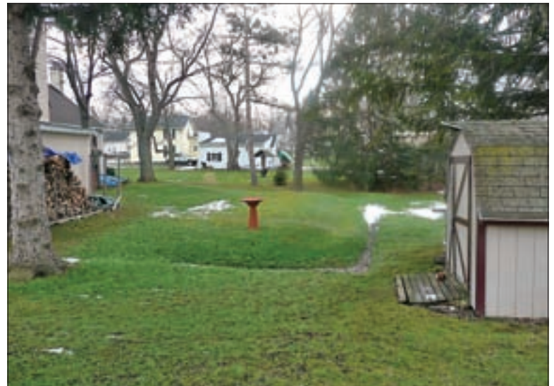
The finished treatment area with the Dirty Bird birdbath camouflaging the lower vent pipe.
