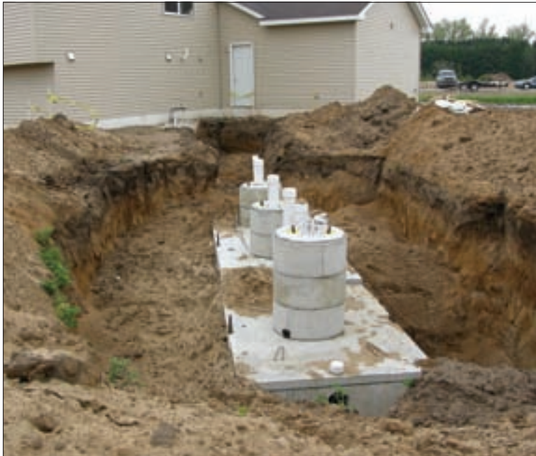
Concrete septic tank and pump tank with concrete risers. Piping from the house has been laid on the proper grade. The trench for the outlet piping has not yet been dug.
