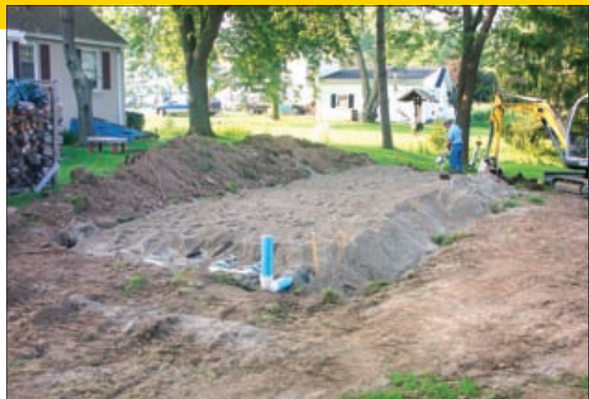
Crew members top the bed with 6 inches of System Sand. A Dirty Bird birdbath from BS Design Corp. will camouflage the lower vent pipe. (Photos courtesy of Meyers Environmental)
