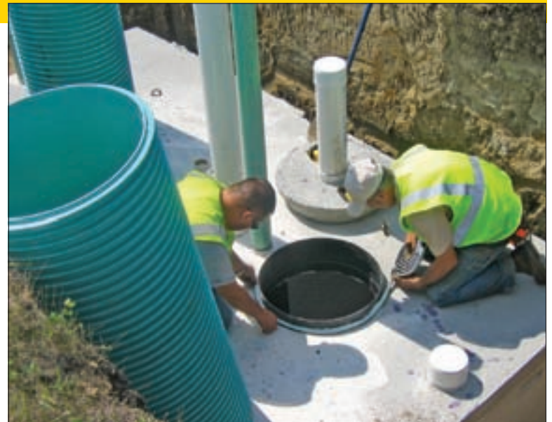
A sound concrete tank with watertight riser connections.
