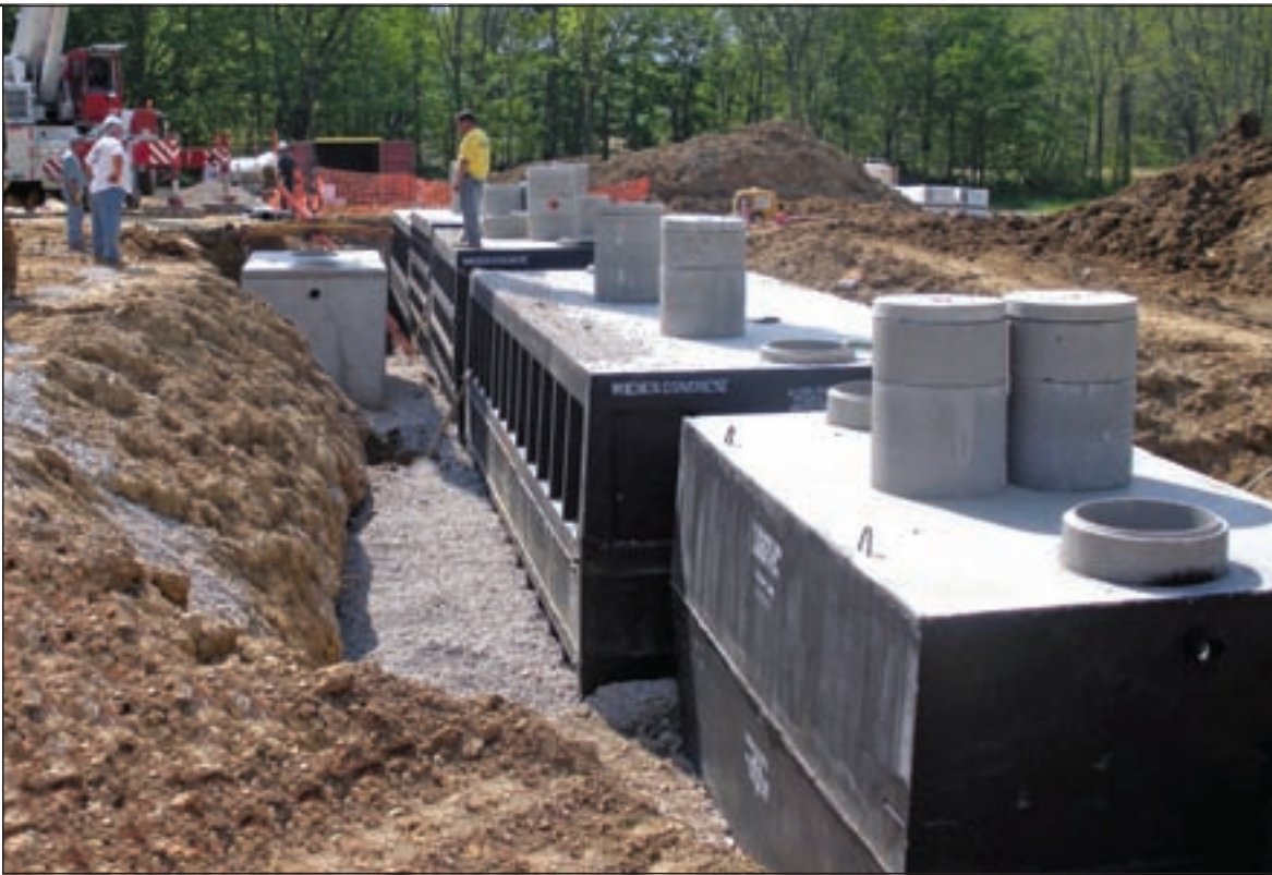
The primary treatment train (right) with the low-flow system — a 2,400-gallon tank with FAST aerobic treatment unit — to the left.
