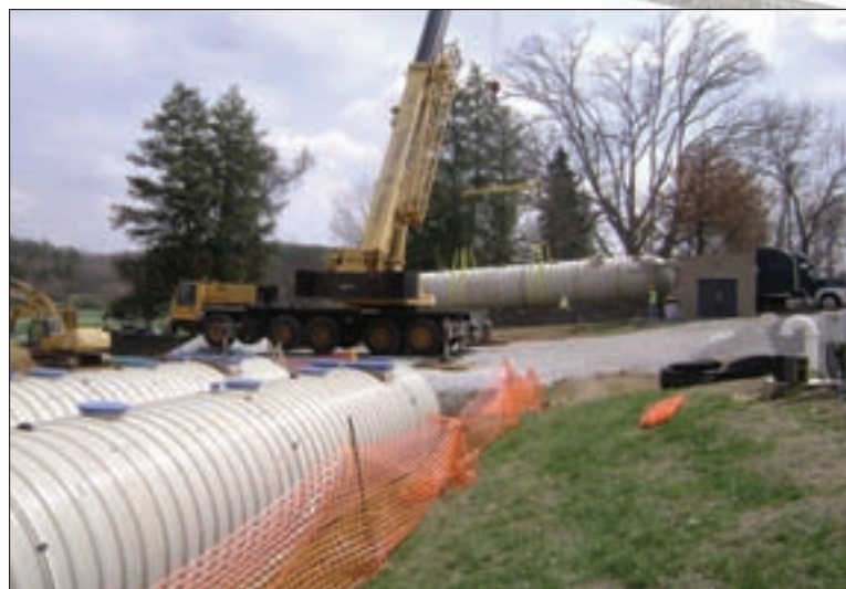
Outriggers support a 200-ton crane as it lifts a 15,000-pound EnviroFilter biofilter tank and prepares to set it 90 feet away on a gravel bed.
