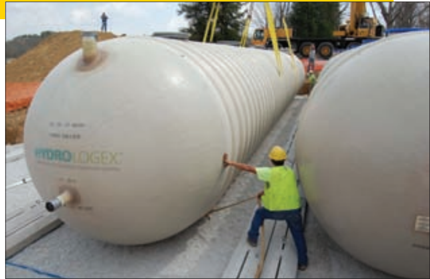
Workers from Dan Cristiani Excavating set the second 10,000-gallon EnviroFilter biofilter from HydroLogex. (Photos courtesy of Saegesser Engineering)
