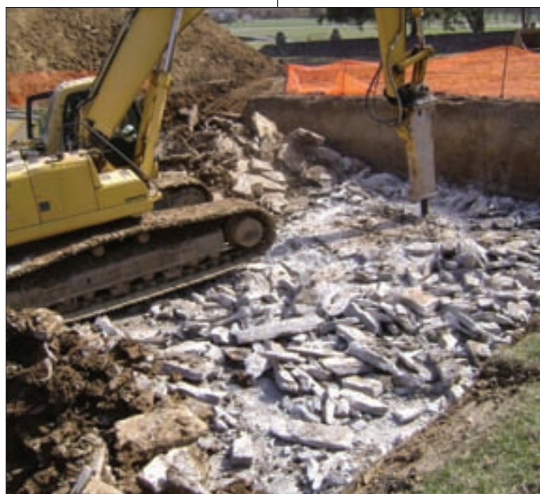
A hoe ram breaks up two feet of limestone before laying a 12-inch gravel base for the last four biofilters.
