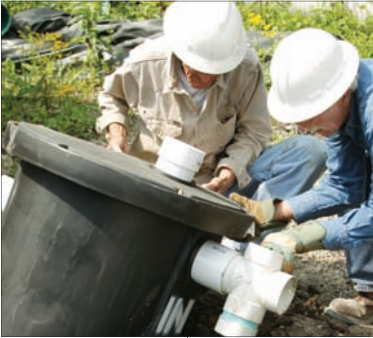
Helper Joe Bobb, left, and technician Phillip Butler check the components on the ATU after installation.
