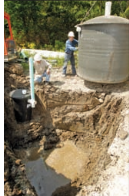
Technician Phillip Butler (right) and helper Joe Bobb work on an ATU installation. Gulf Coast Plumbing is a distributor for Delta Environmental treatment systems.
