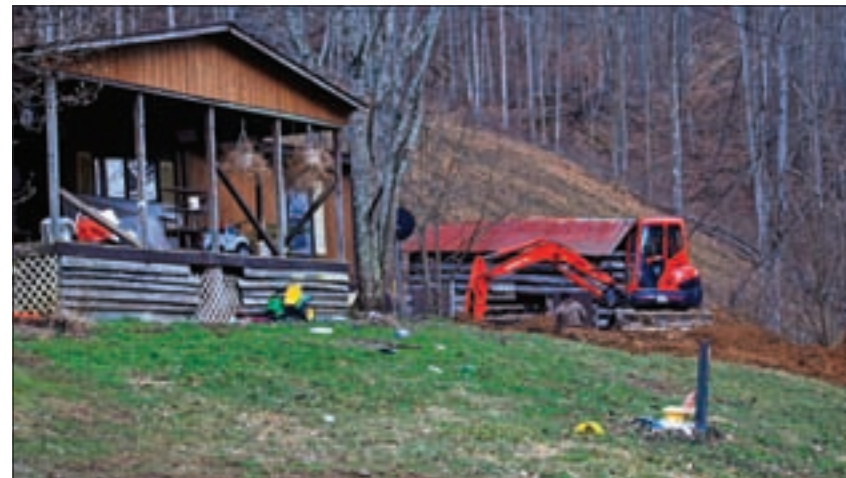
Timothy Davis uses a Kubota U45 tracked mini-excavator to dig holes for the tanks in the small space between the home, property line and creek. (Photos courtesy of Appalachian Photography)
