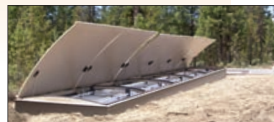
This full-sized AX-Max wastewater treatment system was recently installed at a 50-site campground in the LaPine, Oregon State Park.
