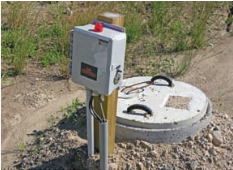
Any electrical connections need to be made outside the corrosive tank environment and located in a weatherproof box near the pump tank or in a nearby building. Shown is a weatherproof box from SJE-Rhombus.
