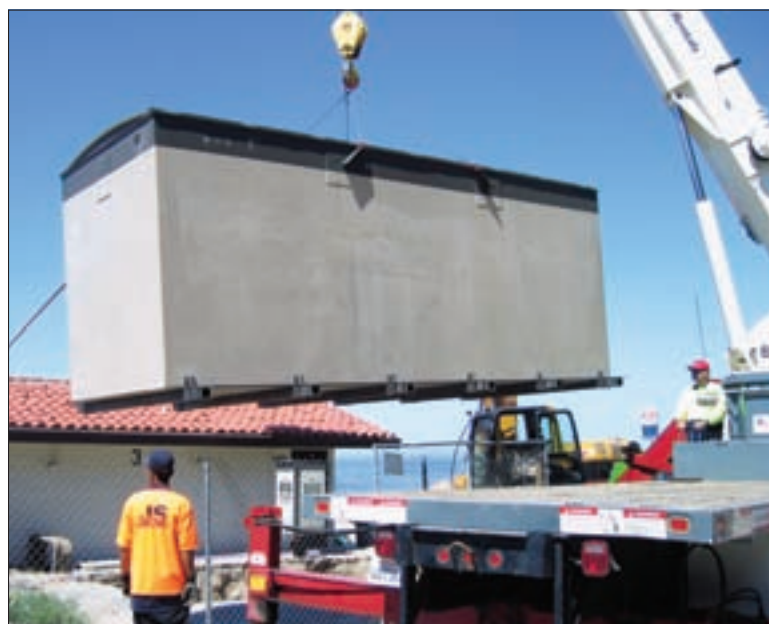
Juan Ramirez of JS Innovative Systems helps a crane operator from United Rentals maneuvering a 6,500-pound AdvanTex AX-MAX module from the delivery truck. (Photos courtesy of BioSolutions Inc.)
