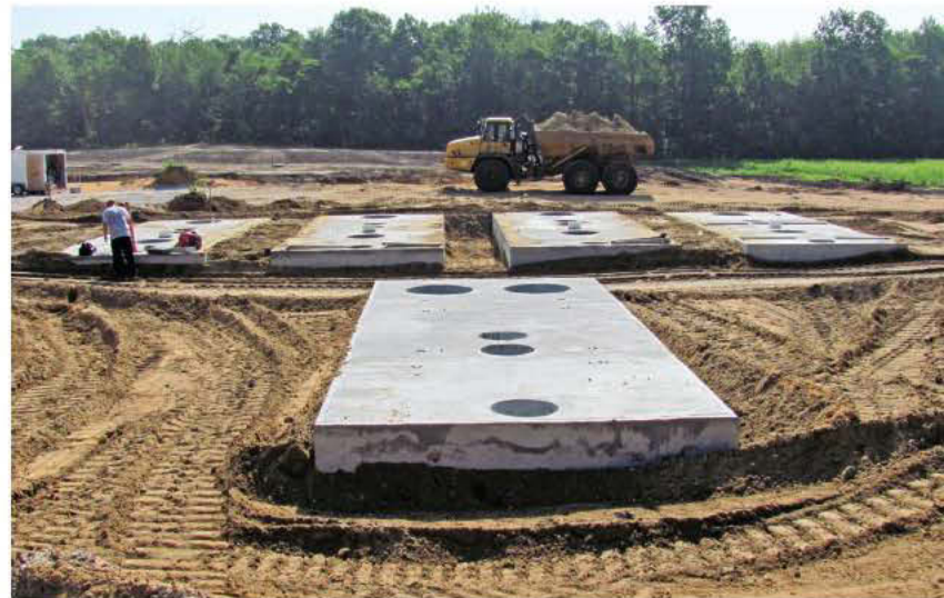
The flow equalization tank with the four FAST treatment tanks behind it. (Photos courtesy of Clear Water Environmental Systems)
