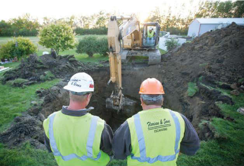
Randy Storey and owner Glen Gonsorowski monitor an excavation for a septic tank.
