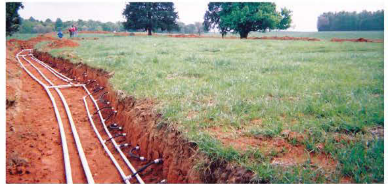
Drip systems are installed shallow and are ideal for sites with difficult, slow draining soils. (Photo courtesy of American Manufacturing Company)
