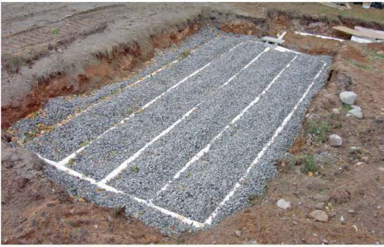
Conventional aggregate systems are still in use after almost a century and serve well in many applications. (Photos courtesy of Infiltrator Systems)
