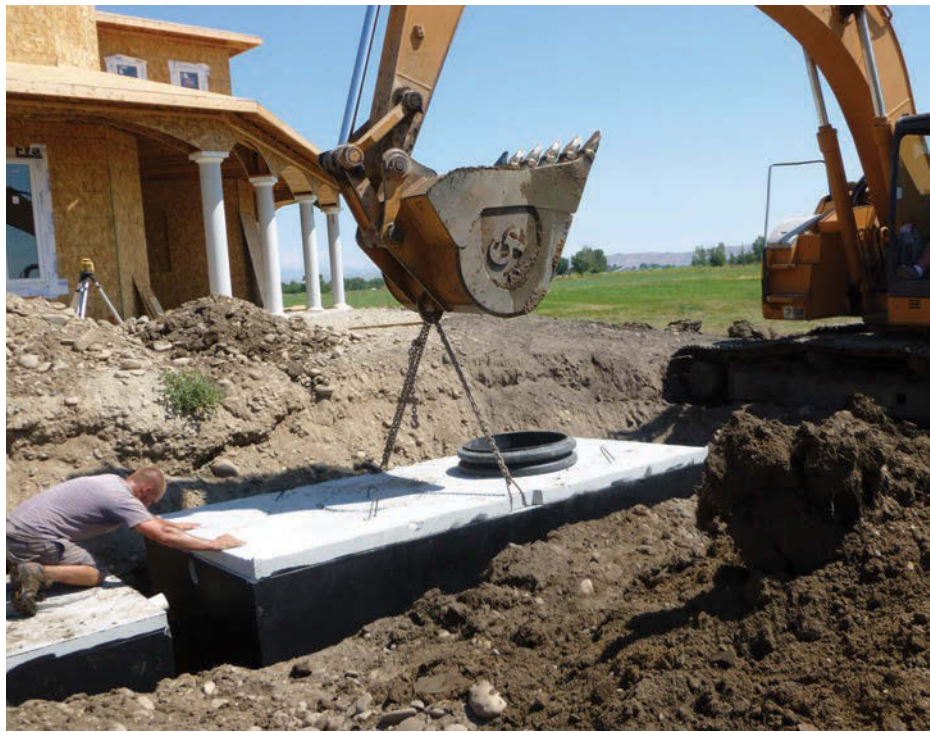
Darren Spiers uses a Case 225 tracked excavator to lower the 1,500-gallon treatment tank as Trevor McCallahan monitors the placement.
