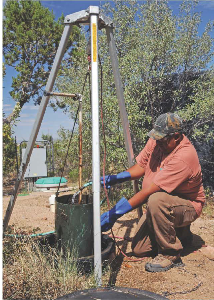
Service technician Steve Sandoval services a SludgeHammer treatment unit.
