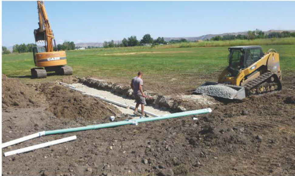
Trevor McCallahan of Spiers Construction prepares to level one of two 60-foot laterals in the drainfield. (Photos courtesy of Spiers Construction)
