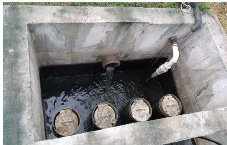
The second compartment of the wet well has four effluent filters installed in 1986. (Photos courtesy of Knight Treatment Systems)
