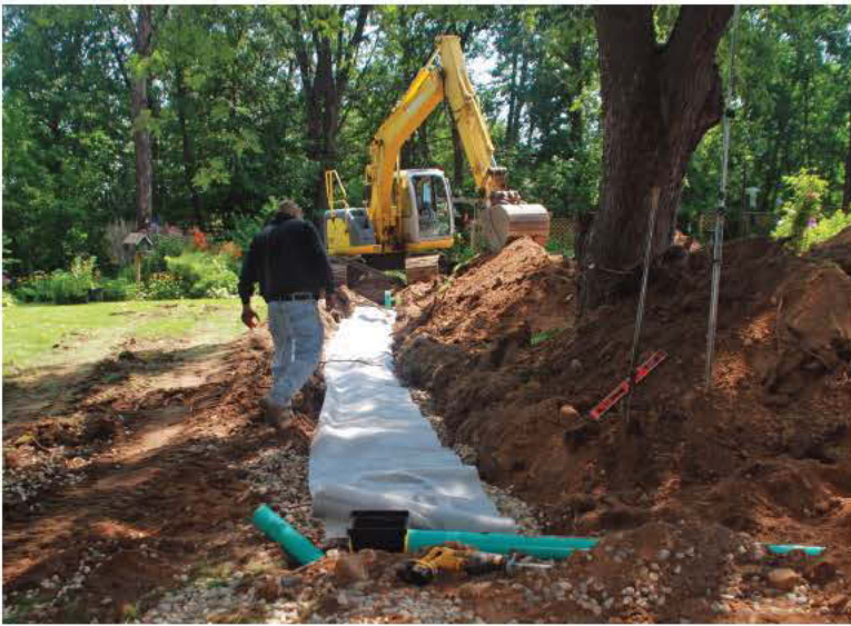
The last drop box feeding the lowest trench in sequence in this system allowed the installation crew to work around a tree.
