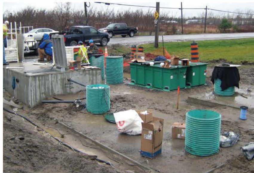
Working beside a heavily traveled road required extra safety precautions for crews setting up the Nibbler SBP treatment tank. AdvanTex AX20 treatment pods with room for a third are shown to the right. (Photo courtesy of Orenco Systems)
