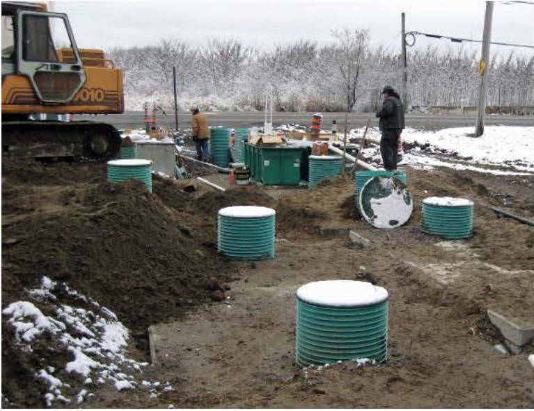
Workers clean up as system backfilling begins. (Photo courtesy of Orenco Systems)
