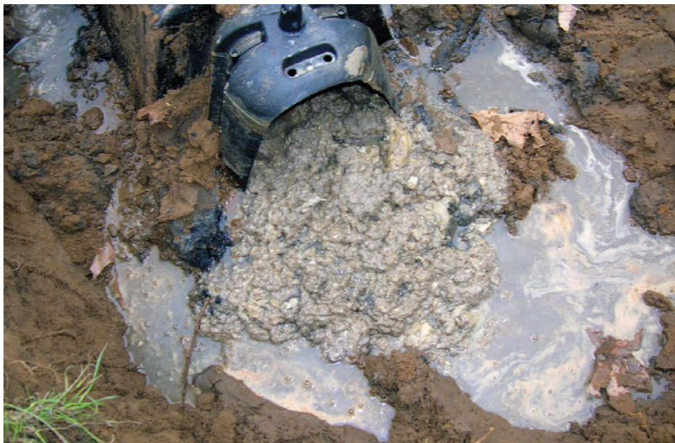
Gray, lumpy material had partially filled the drainfield media, restricting effluent exfiltration. The homeowner would not acknowledge discharging a substance that would have led to this condition.
