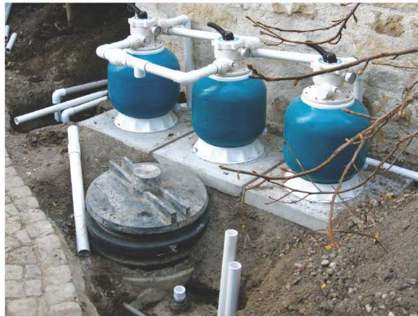
The partially backfilled storage tank sits in front of the skid-mounted filter array. Workers are still installing the underground plumbing lines. (Photos courtesy of Water Recycling Systems)
