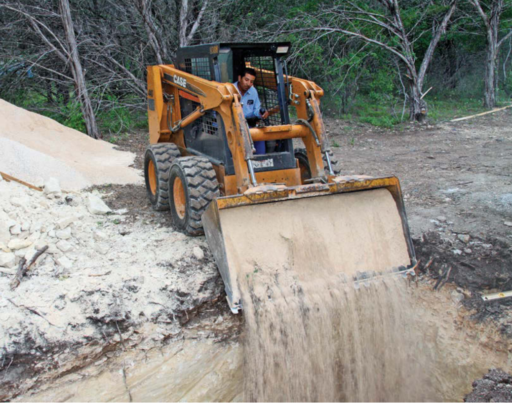
LEFT: Field supervisor Miguel Casas excavates and beds a hole for a septic tank. BELOW LEFT: Ryan Seidensticker (left), manager with Block Creek Concrete Products, and Miguel Casas place a BioRobix B-550 aerobic treatment system from Enviro-Flo.
