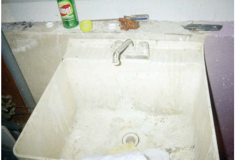
A basement utility sink was coated with up to 1/4 inch of dried latex paint. The drainfield showed evidence of a sealed infiltrative surface, likely from paint discharge. The homeowner admitted operating a painting business and regularly washing brushes and rollers in this sink.
