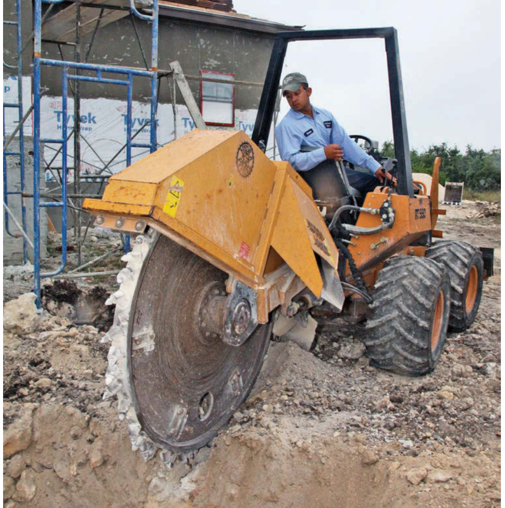
Field worker Anselmo “Chemo” Juarez Jimenez uses a Hydra Wheel rock saw from River City Mfg. to break up the ground for a septic system job.
