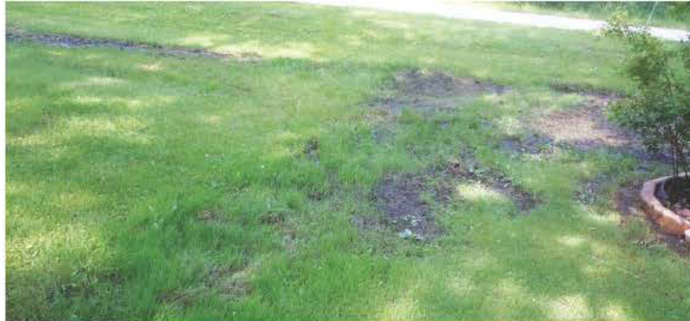
An example of where a hydraulic load test would not be conducted: an obvious drainfield failure.
