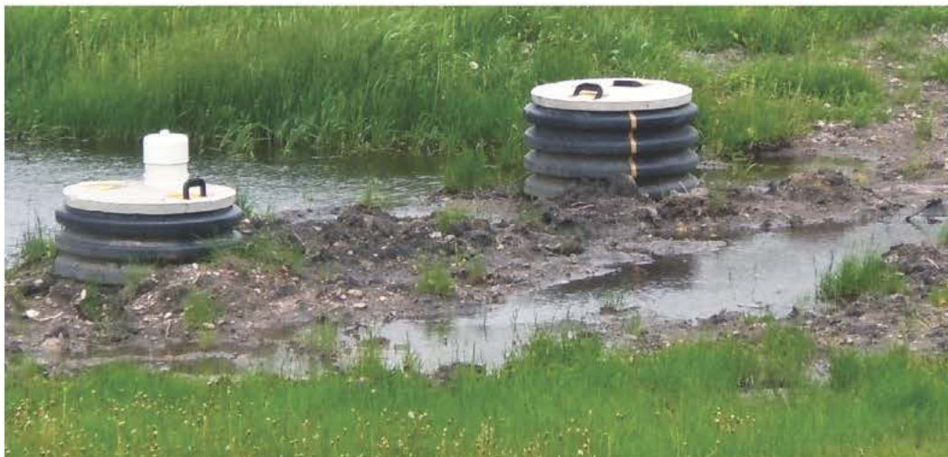
Surface water around the tank risers is a situation where a hydraulic load test would be used to evaluate the system capacity.
