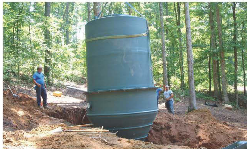
Workers from C.R. Barger & Sons observe as a crane operator sets the 17-foot-high trickling filter. (Photos courtesy of Southeast Environmental Engineering)
