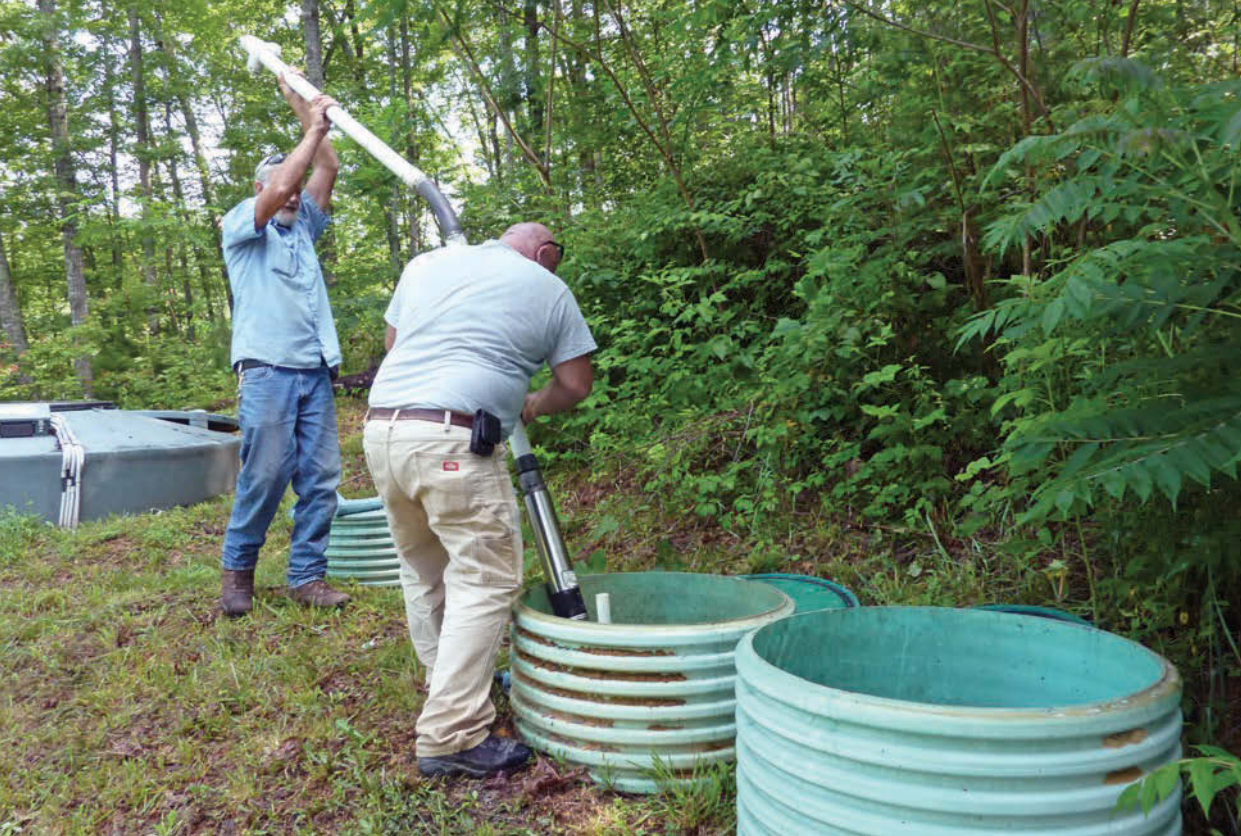
Jim Magill and Johnny Gautreaux from C.R. Barger & Sons install one of two 1 hp, 30 gpm high-head AY McDonald turbine pumps in a concentric vault to dose the drip field.
