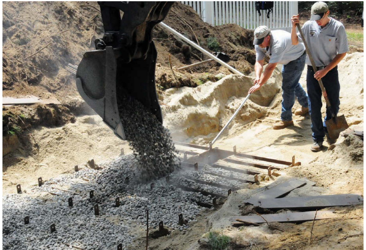
Owner Steve Buttermore, left, and Grant Buttermore install an onsite system using a Geomatrix GST leaching system.
