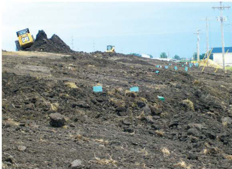
Jim Scott and Doug Bennett backfill using two Caterpillar skid-steer loaders. The drip field has 49 risers.
