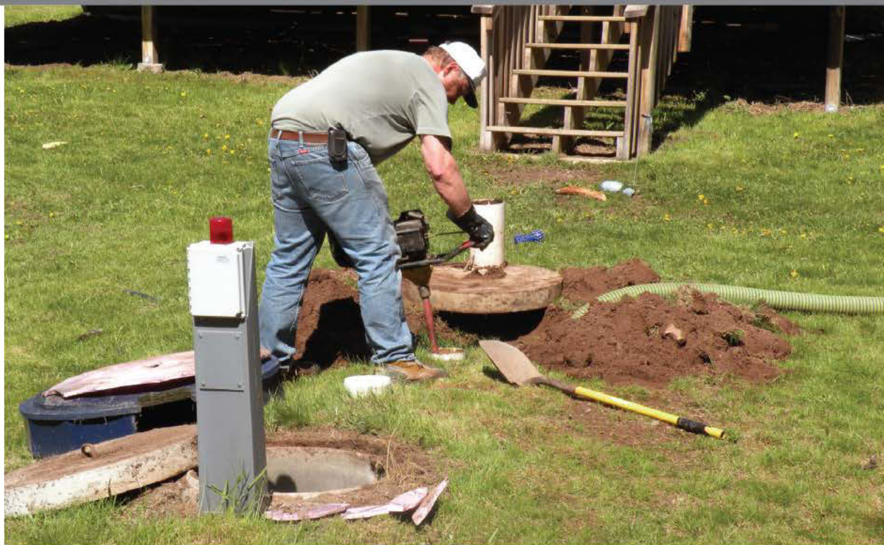
Risers brought to the surface make maintenance of septic tanks easier.
