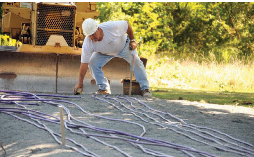
Pete Damiani lays and straightens tubing from American Manufacturing on a dosed system installation.
