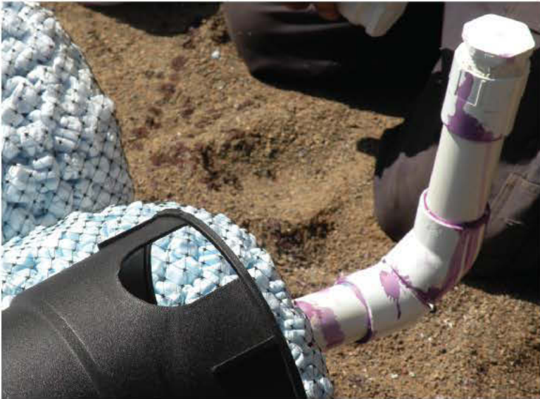
Here are two examples of clean-outs at the end of pressure distribution laterals in treatment mounds. One uses rock media and the other uses a synthetic aggregate.
