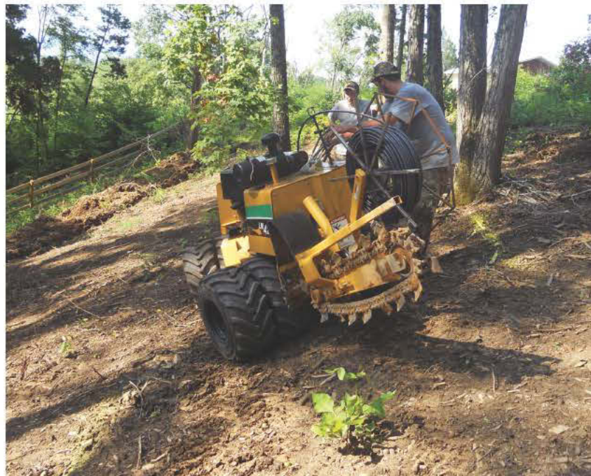
Cliff Kendall (right) and Barry Little install Geoflow drip tubing using a modified LM42 Vermeer walk-beside vibratory plow with 50 hp turbo diesel. The plow has dual wheels on the downhill side.
