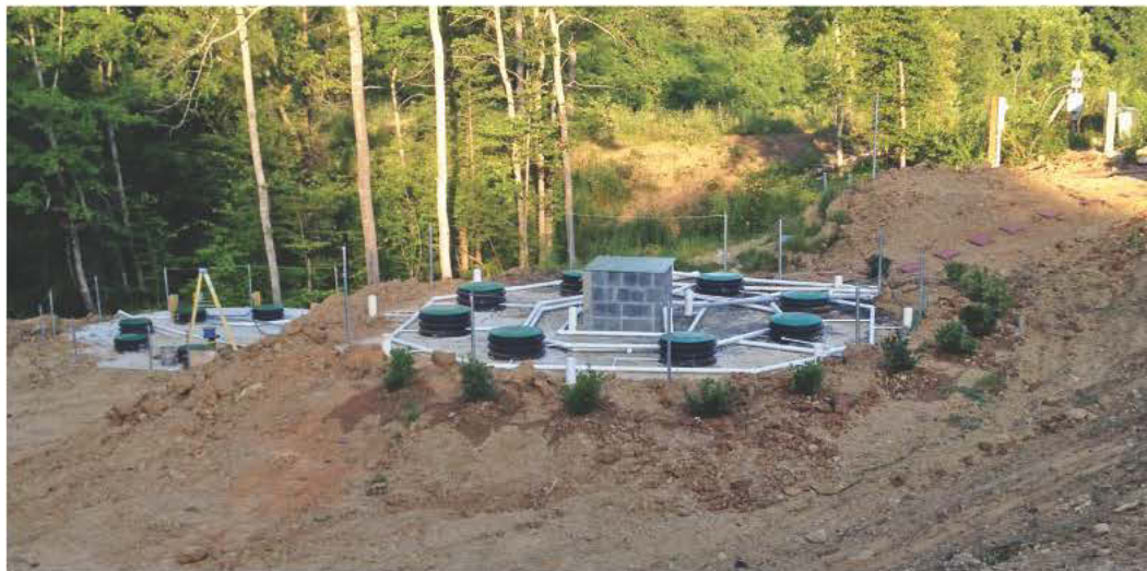
At the left, the 35,000-gallon poured-in-place circular dosing tank; at the right, the treatment tank with shrubs planted around it. (Photos courtesy of Dart Kendall)
