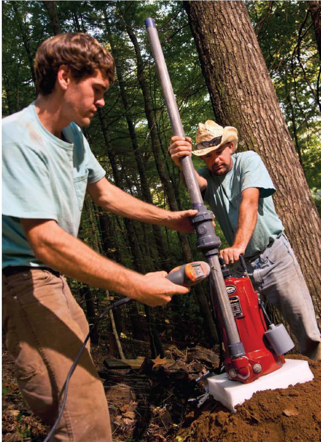
In the process of installing a Liberty pump in a new system, Justin Kilgore drills air release holes, while Heath Kilgore steadies the pump.
