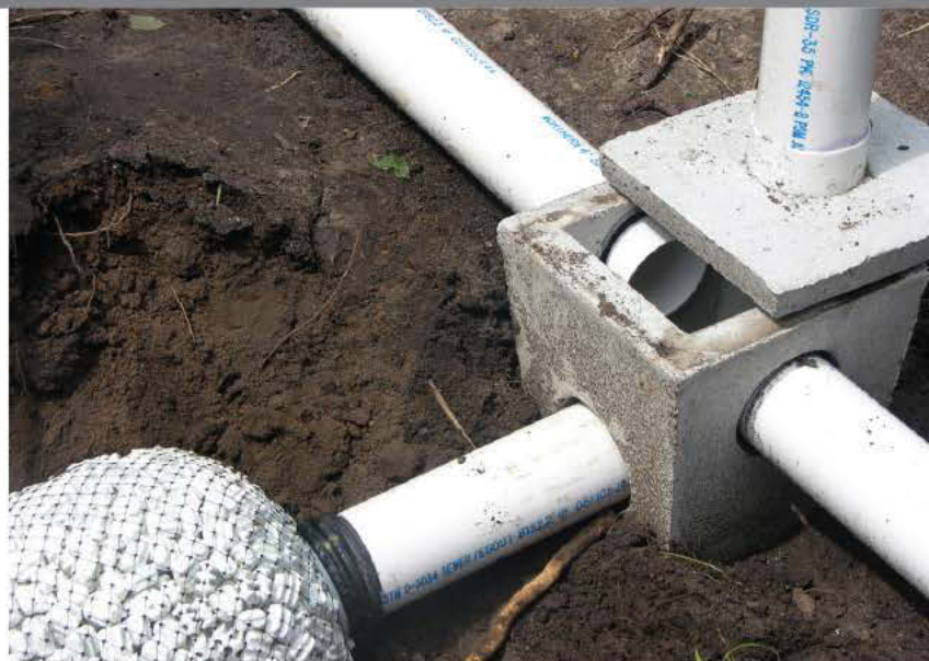
Drop boxes are being installed where EZ Flow media is used.
