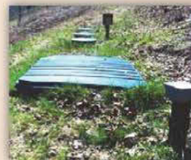
Mud River Project Over 50 Salcor 3G UV Units installed with ANUA peat filters.
