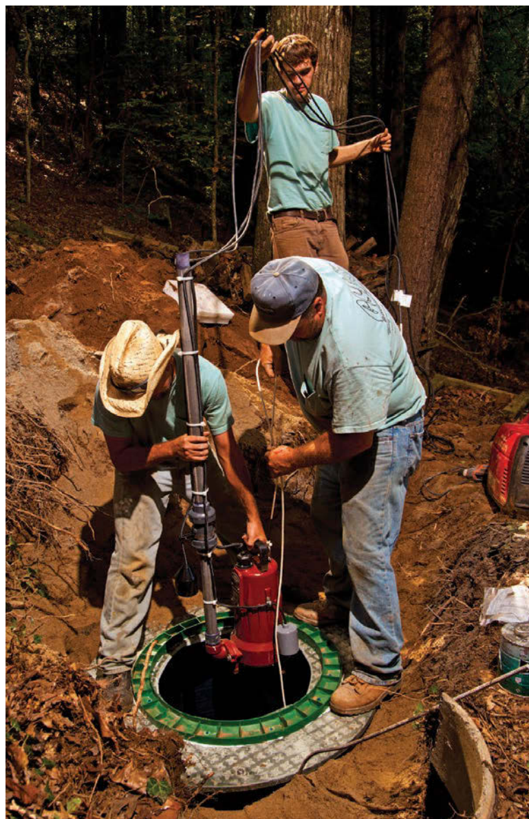
With Justin Kilgore keeping electrical lines under control, Heath (left) and Harold Kilgore lower a Liberty Pump into a grinding station in Blue Ridge, Ga.
