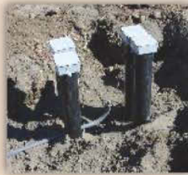
Cascade School Four Salcor 3G UV Units connected in a parallel/series array
