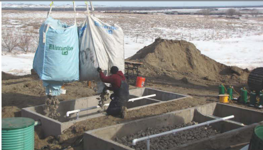
Justin Buchanan of E-On Northwest in Bozeman, Mont., empties MetaRocks into the treatment chamber of an Eliminite fixed-film bioreactor. (Photos Courtesy of Eliminite, Belgrade, Mont.)
