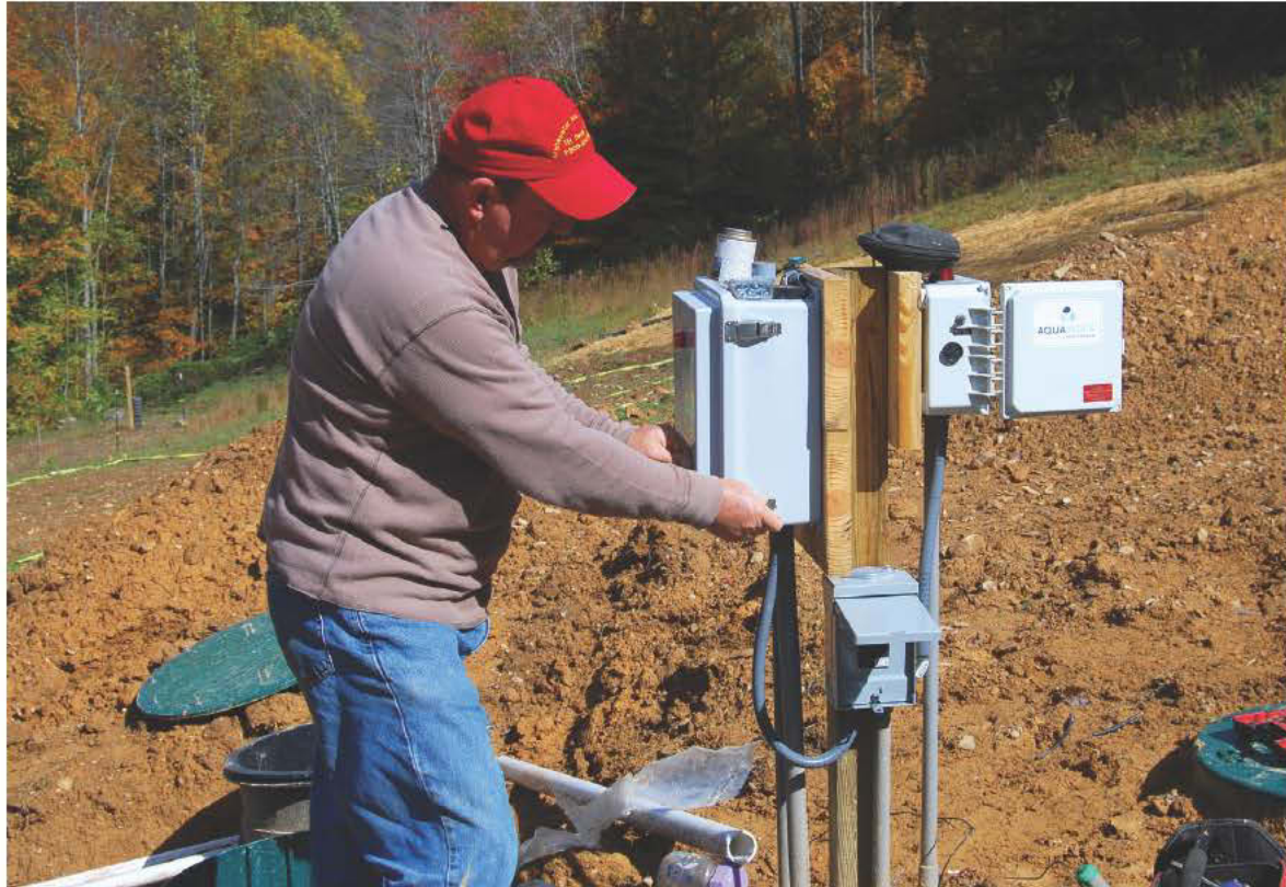
ABOVE: Timothy Davis checks control panels from Delta Environmental (large box he is touching) and Aquaworx by Infiltrator (small open box on right). (Photo by Ric McDowell) BELOW: Davis (left) and equipment operator Bob Adkins use a Bosch laser level to measure lines and level the ground for trenches.
