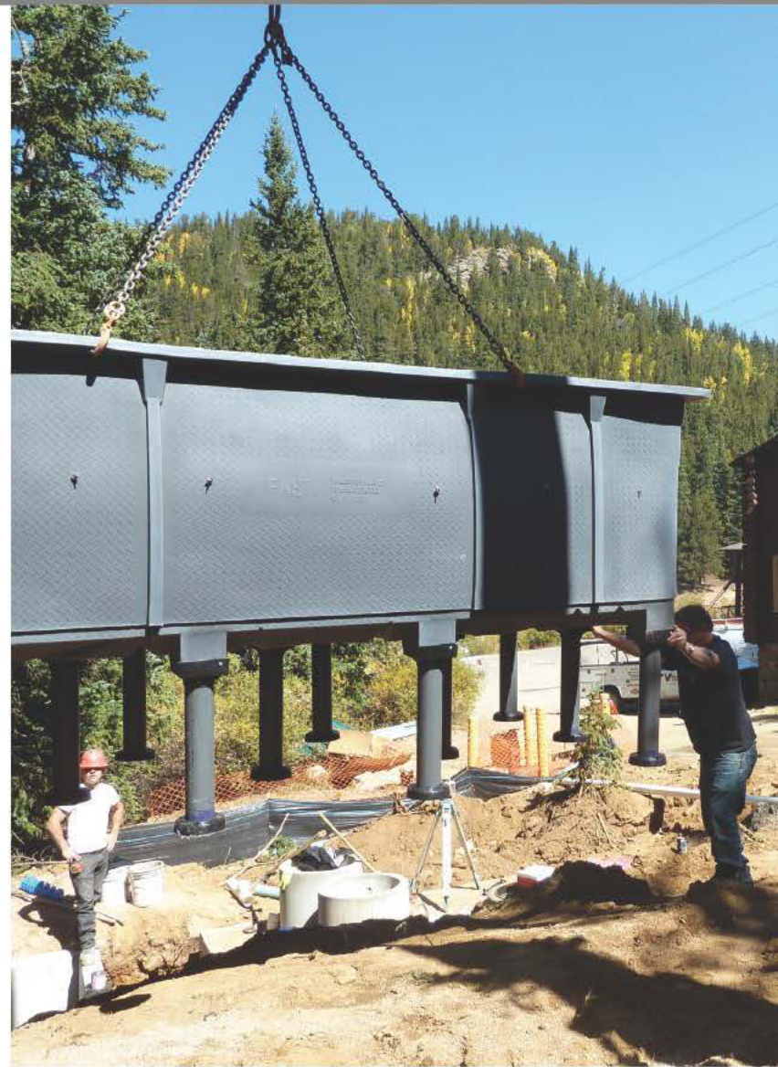
An Esco Construction Co. backhoe operator lifts the 1,600-pound Bio-Microbic's HighStrengthFAST 4.5 bioreactor as Leo Castro of All Service Septic helps steady it. (Photos courtesy of All Service Septic)
