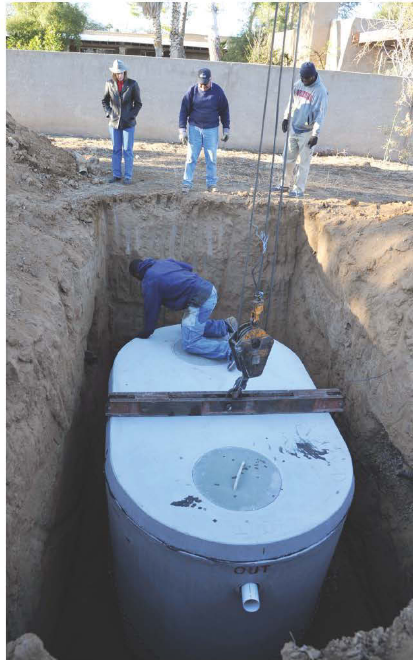
Top (from left) Farrell-Poe, Roberto Rozco, co-owner of Arizona Precast, Brian Lewis, owner of Guaranteed Contractors Inc., and Marcus Lewis (bottom) of Guaranteed Contractors Inc. position a septic tank at a Green Valley home.
