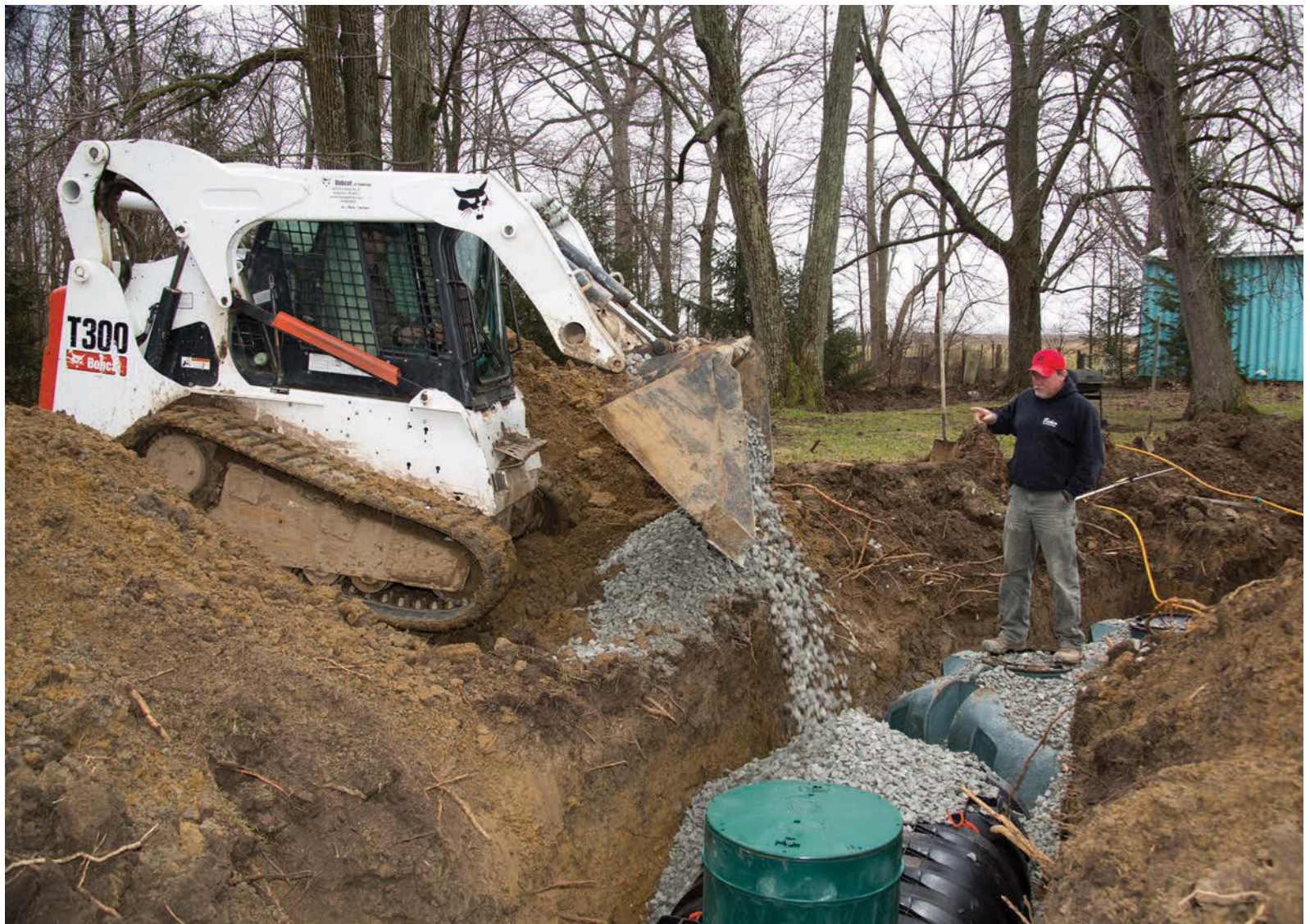
Baker oversees John Frye, who is dumping rock over Infiltrator Systems and Norwesco tanks placed in series during a new system install.
