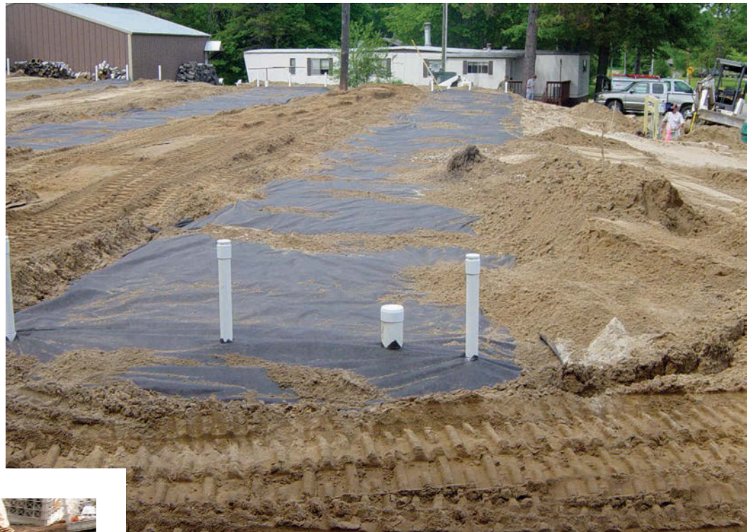
ABOVE: Having inspection ports installed assists in future system management. LEFT: Consult the as-built drawings as the installation proceeds.
