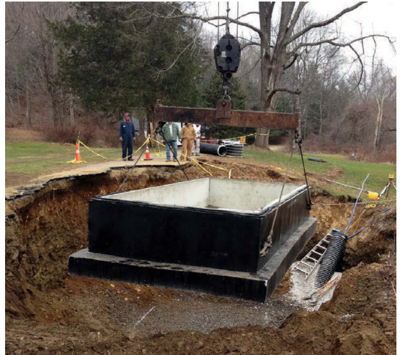
Mark Green (left) and Tommy Dauti and workers from Dauti Masonry oversee installing the bottom section of the pump tank. (Courtesy of Mark Green)
