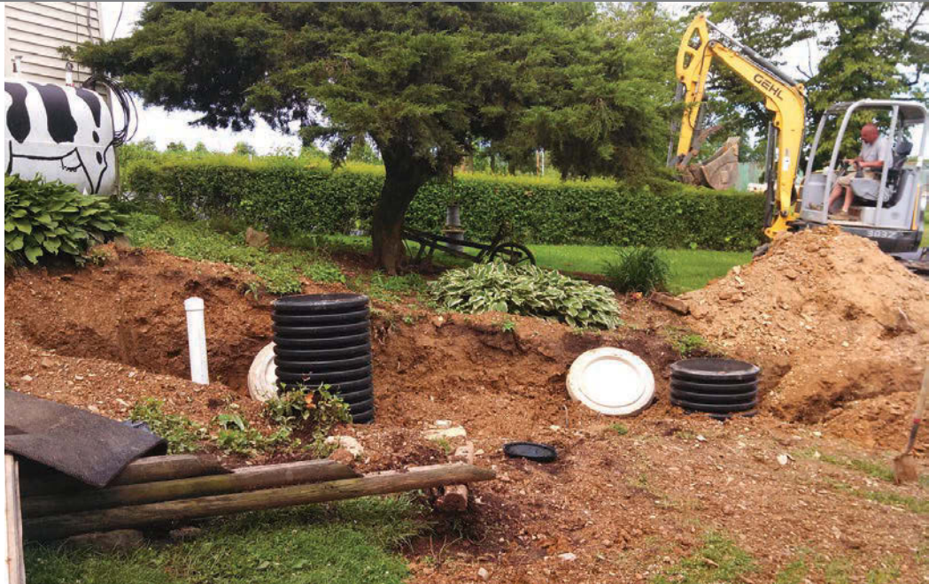
Tom Erb moves the Gehl 383Z mini-excavator into position to backfill around the septic tank.
