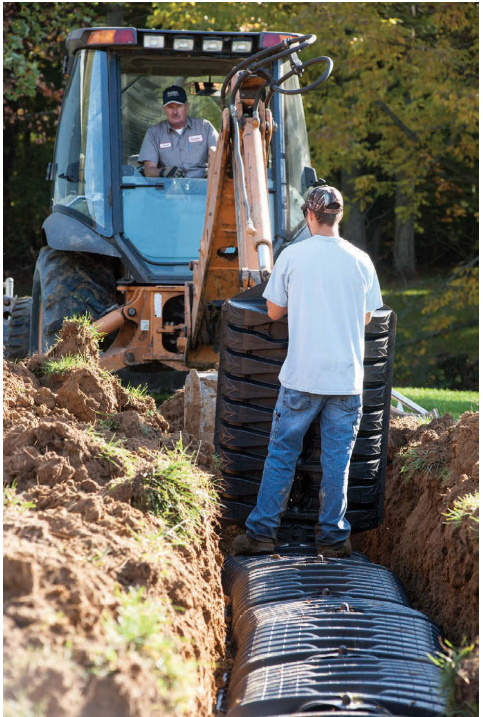
Owner Mark Hacker uses a backhoe to dig a field bed, while Jordan Winning installs a Quick4 Plus low-profile chamber system from Infiltrator Systems.
