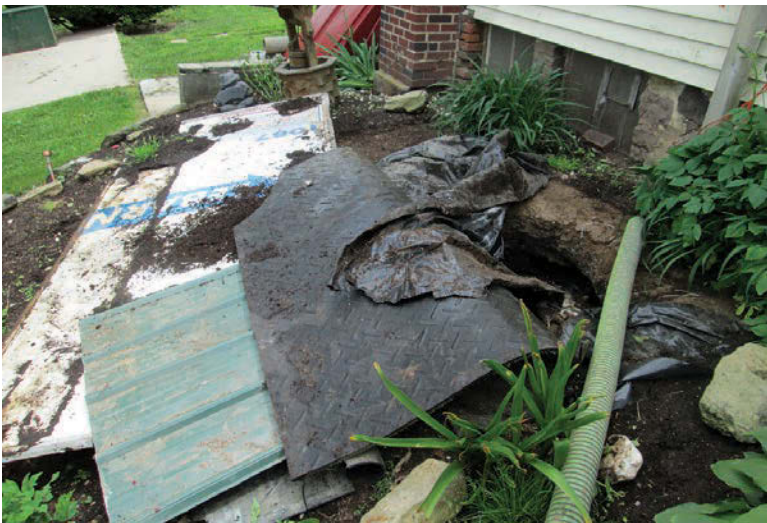
The rear door of a semi-trailer and other material cover the collapsed 350-gallon metal septic tank. (Photos courtesy of Thomas H. Erb and Sons)
