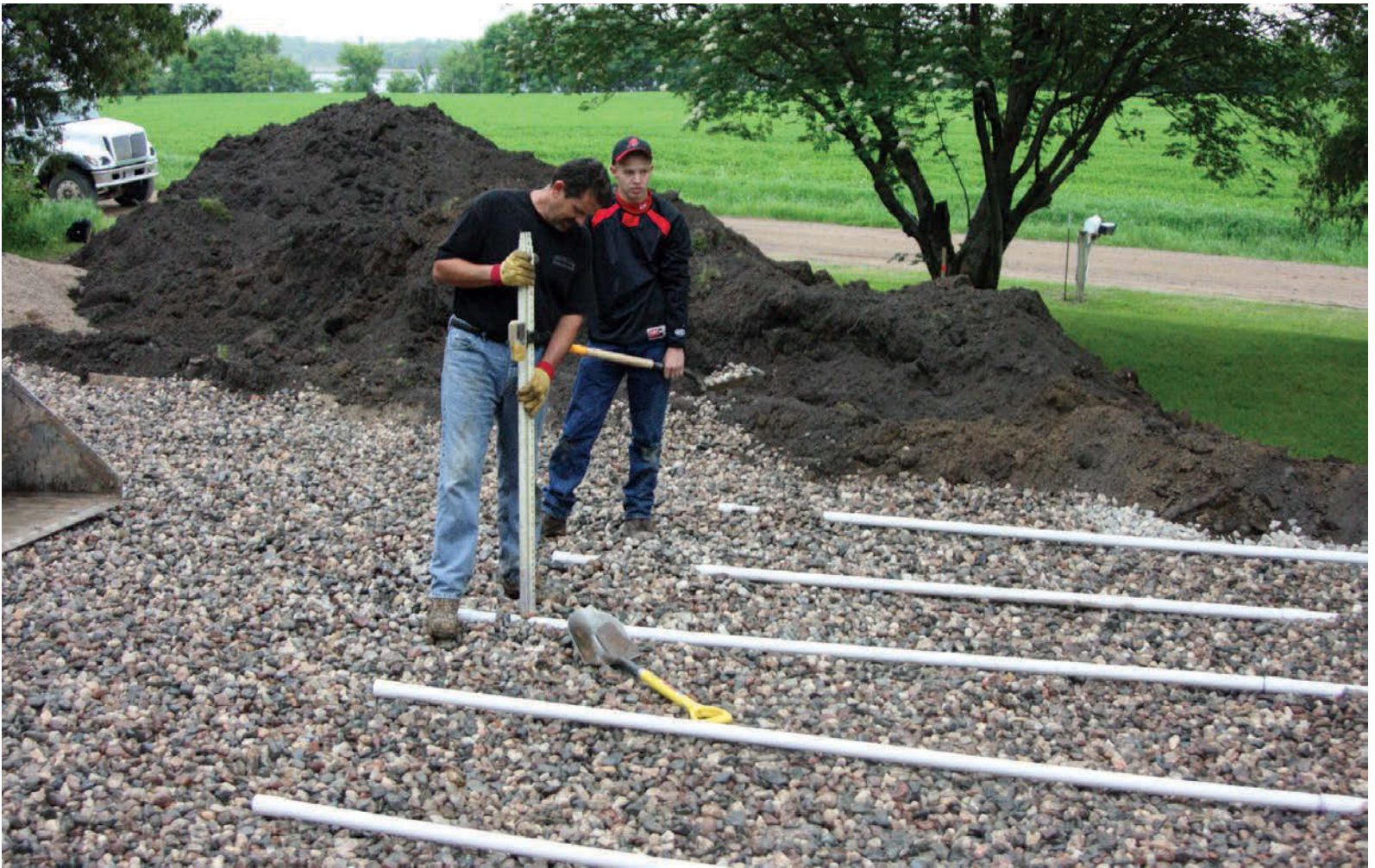
Dean Flygare and David Hoiem use a Crain grade rod with a Spectra Precision laser receiver to level laterals while installing a new system.
