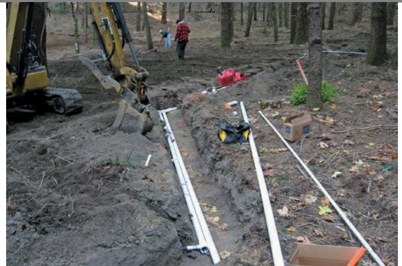
The subsurface drip irrigation system at URJ Camp Newman consists of 13,800 linear feet of 1/2-inch-diameter Geoflow pipe set 12 inches deep.
