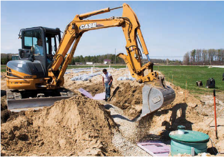
Chad Christiansen, left, and Mike Fellner begin to cover the mains taking treated wastewater to the distribution field. On top of the pipes are two pieces of 1-inch-thick R-5 Foamular 150 insulation. "This is Wisconsin. We insulate everything," says installer Doug Fellner.
