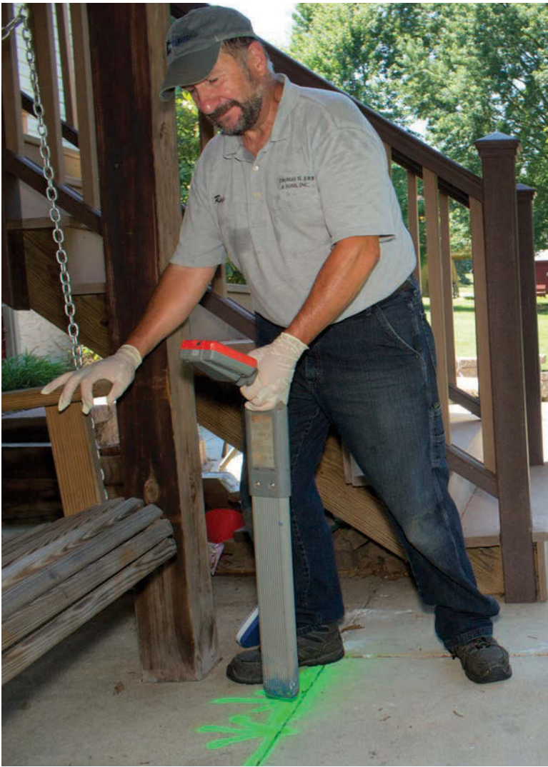
Thomas Erb and Sons Inc. president Ray Erb uses a RIDGID KD-4550 locator/receiver to locate the edge of an existing septic tank to connect a public sewer line to a home.
