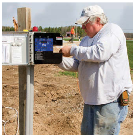
Doug Fellner installs the SJE-Rhombus control panel for the wastewater system at Door County Coffee & Tea Co. The panel is mounted next to the 5,000-gallon dosing tank and controls timed dosing between two distribution beds. The red light on top signals a malfunction, but Fellner also repurposed a float from the old septic tank so it will sound an alarm inside the business if a pump fails.
