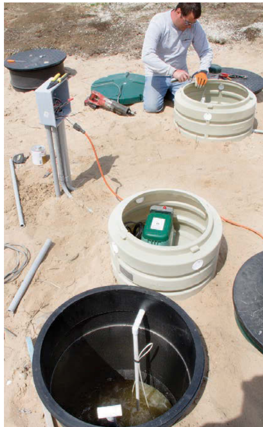
The SludgeHammer S-86 units at Door County Coffee & Tea Co. are aerated by Hiblow pumps. Mike Fellner, at top, installs PVC pipe to connect the pump in its riser to the pretreatment tank. The pump at bottom is being tested. All power wiring meets in the elevated junction box at top left.
