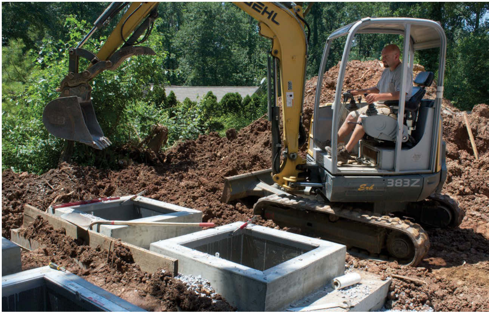
Tom Erb fills in stone with a Gehl 383Z mini-excavator during the installation of a sand filter at a residence in Brickerville, Pa.
