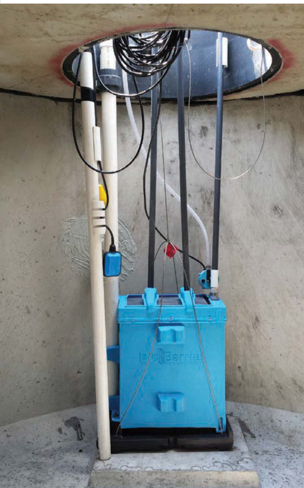
The BioBarrier unit in place inside the new concrete tank.
