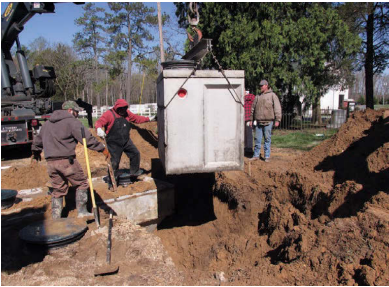
Brody Towers (left), Paul Hayes (second from left) and Robert Blockston (right) set the filtration tank for the company's Hydro-Kinetic installation. The tank has suspended growth media to increase the removal of organics.
