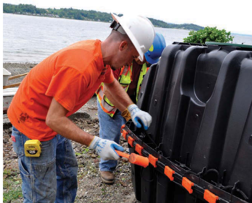
BELOW: Ian Midgette hammers the locking seam clips into position on the septic tank.
