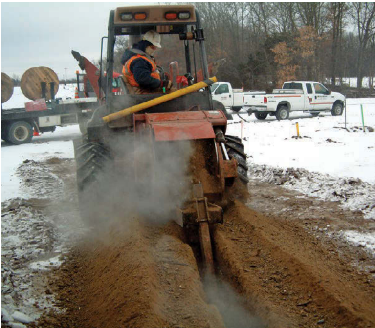
When working in cold weather, give your equipment time to warm up before putting it to work. (Photo courtesy of Ditch Witch)
