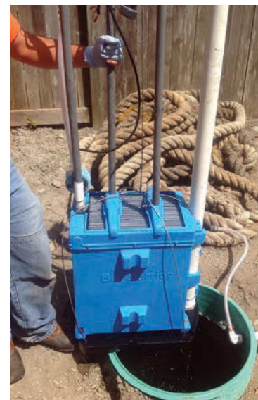
A worker prepares to lower the plumbed BioBarrier membrane bioreactor into the treatment tank.
