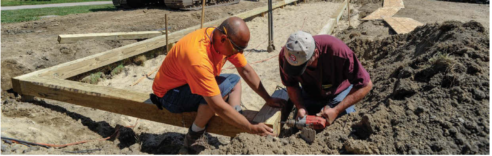
Excavator Kevin Wilkie, left, and installer Brendan Cory attach timbers used in the construction of the box to contain a bottomless sand filter for an ATU system.
