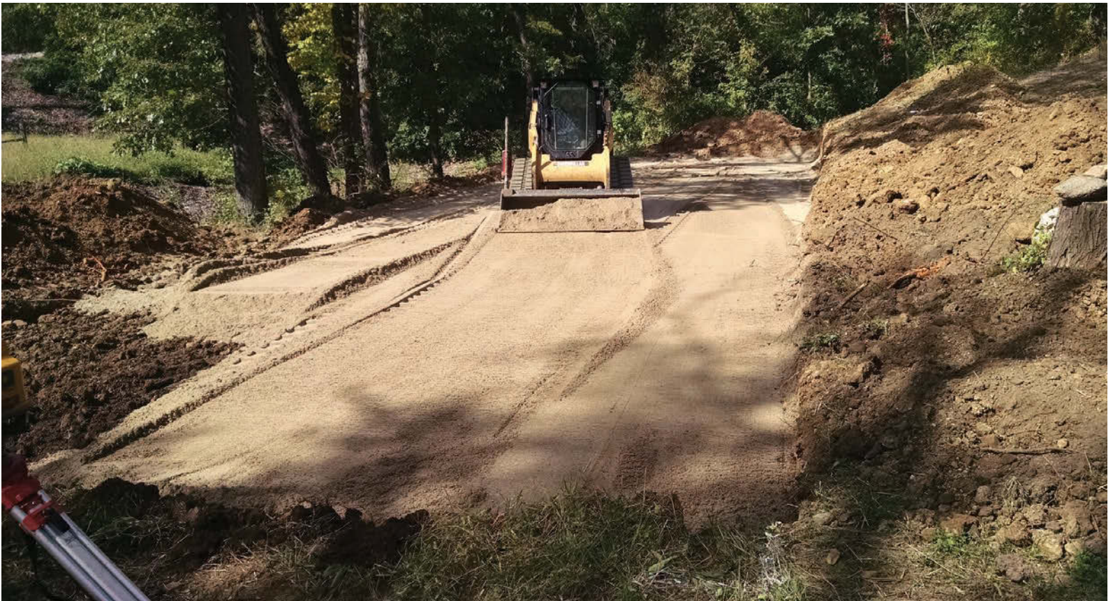
ABOVE: Maguire Backhoe places 6 inches of sand with a Caterpillar 259 rubber-track skid loader to create a sand bed with 1 percent slope.
